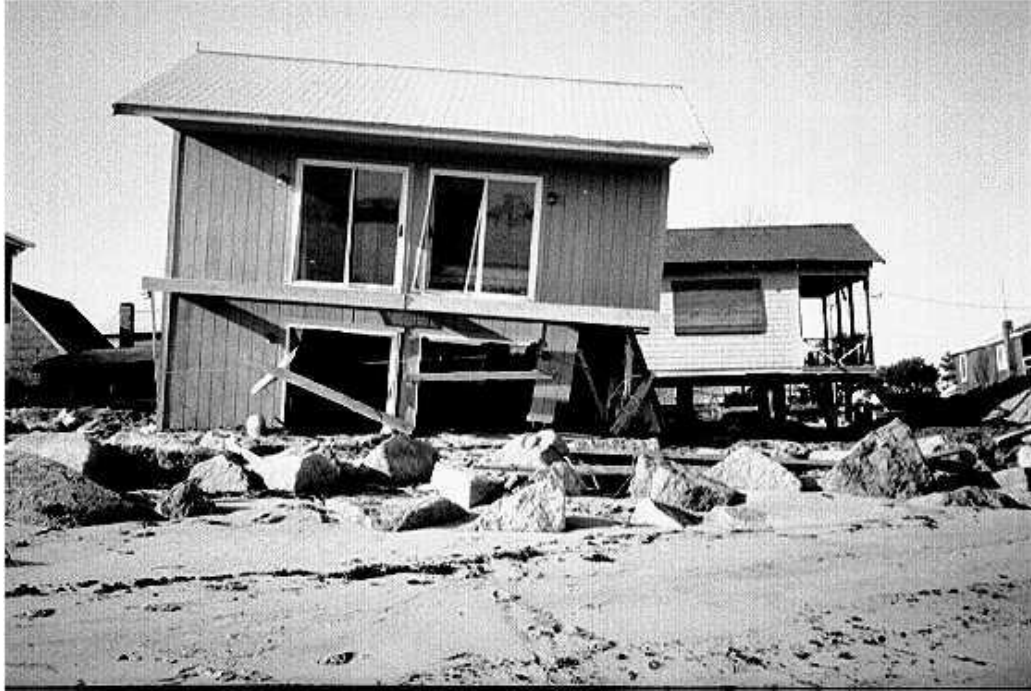
Figure 1. Shore front erosion. Topics of land use, slop and erosion as well as a number of related issues are brought together by what is happening along portions of the Maine coast. While the situation at Camp Ellis probably shows a worst case scenario, many other places along the coast have the potential for scenes such as this.
