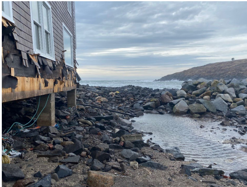
Harbor Breakwater and Damaged Building, Monhegan Island
