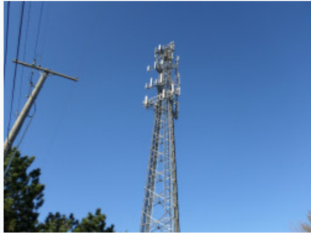
A cell tower carrying antennas of four cellular networks. Notice how this does not resemble a weather balloon.
