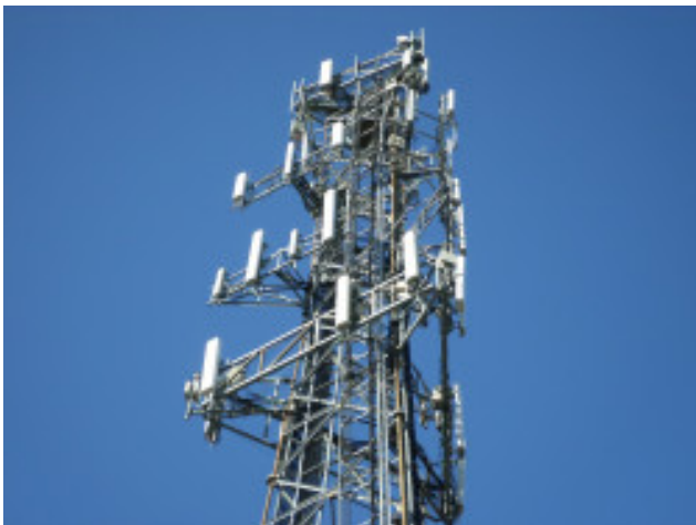
Cellular antennas on a lattice tower with four carriers.
