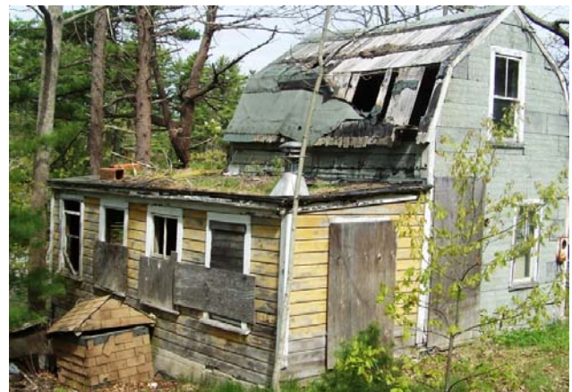
(Brunswick, ME) The spring 2007 storms that pummeled Knox County significantly damaged this home. Photo by Lance Carpenter, FEMA.
