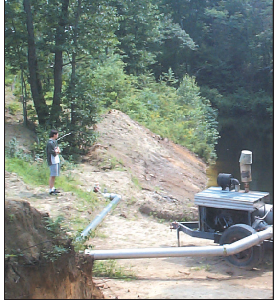
Streamside Pumping Station
