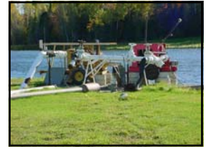
Pond pumping station.
