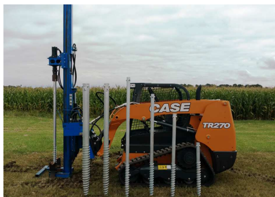
Ground Screws Source: Solar Power World
