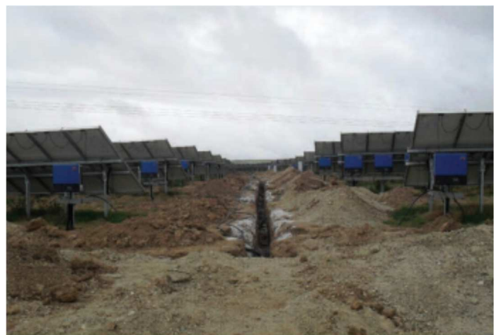
Image of a conduit trench with topsoil and subsoil separated on opposite sides. Note the blue inverters attached to the racking structure.
