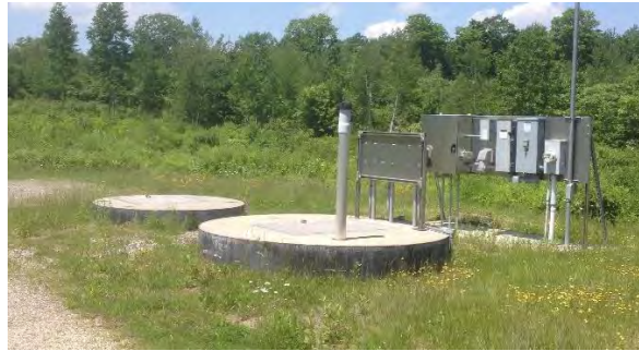
Sewer Pump Station on RT 26
