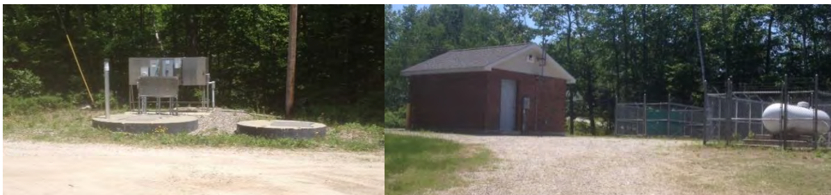
Sewer Pump Stations on RT 122
