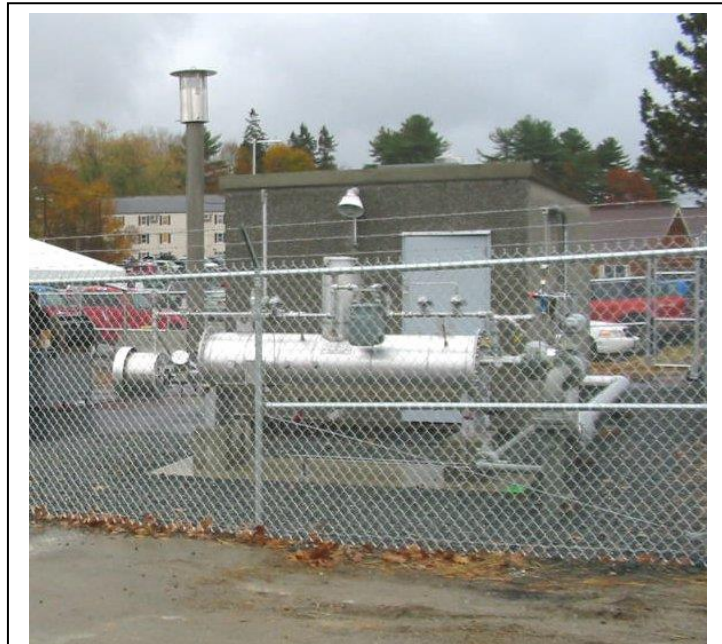
2013 Natural Gas Pressure Reduction Station at 3 River Road serving downtown Bucksport businesses & residences.
