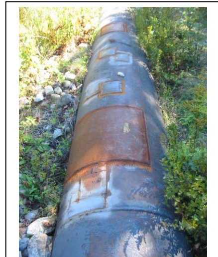
The 36" pipeline near Alamoosook Lake has needed some work over the years.
