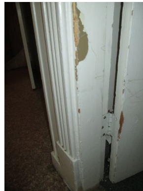
Paint in poor condition
