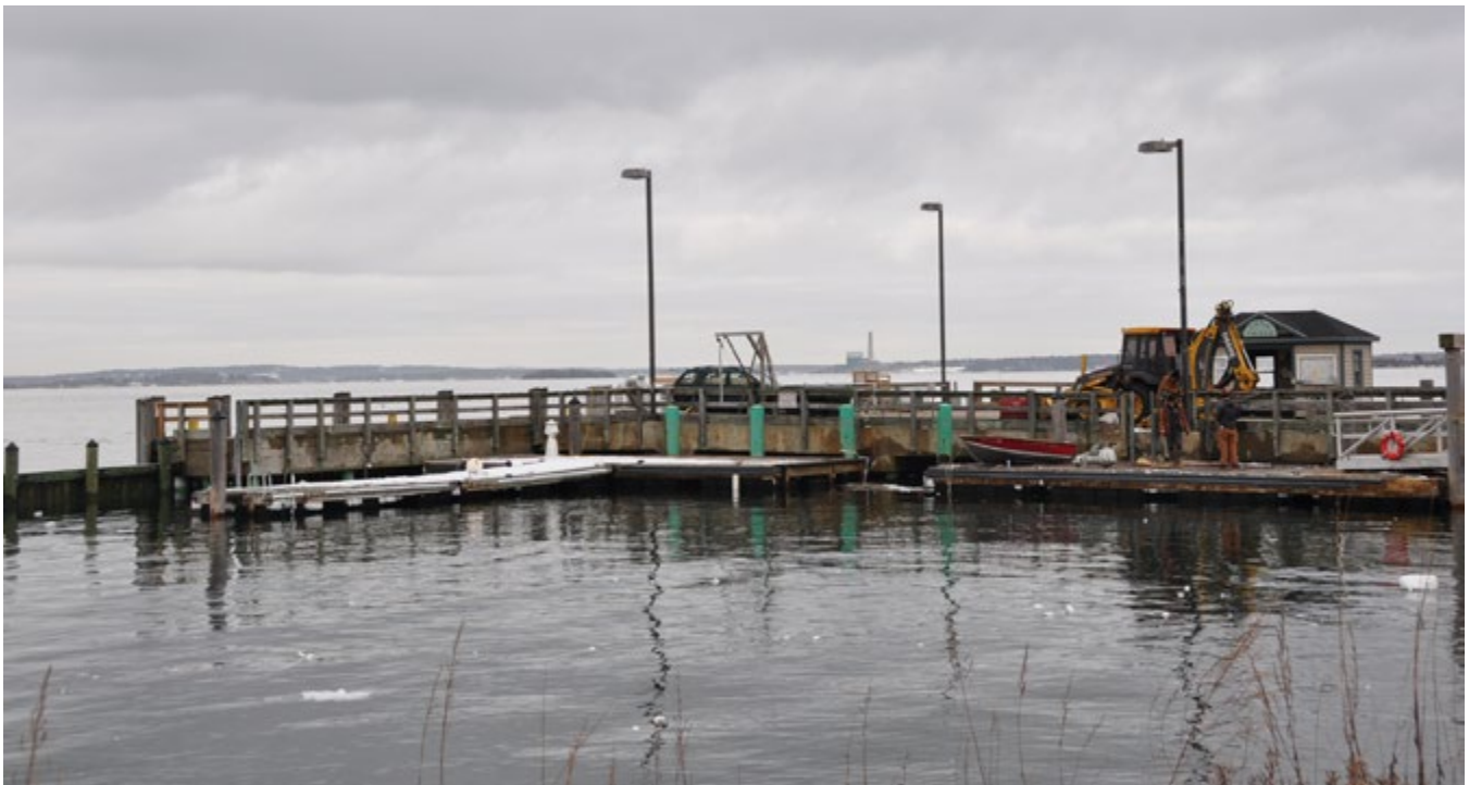
Mariner's Wharf under repair after a January 2022 storm. The town held emergency meetings after the storm to assess damage and plan repairs. Photo: Elizabeth Marchak
