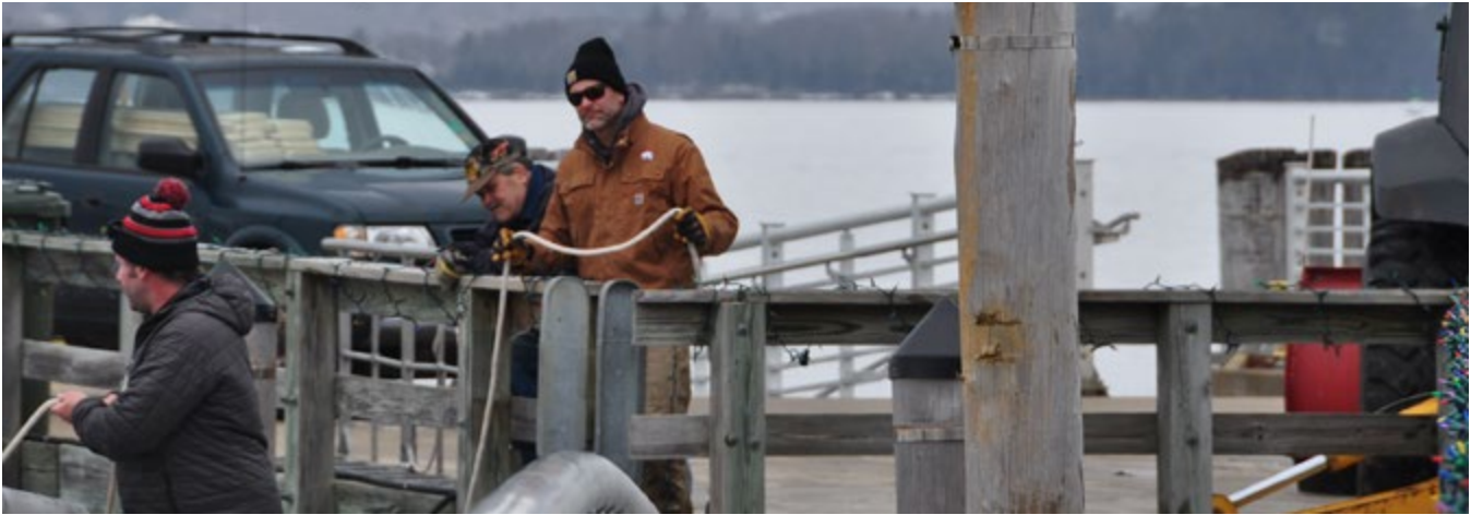
Volunteers work on repair efforts at Mariner's Wharf following the January 2022 storm that damaged floats and pilings. Photo: Elizabeth Marchak
