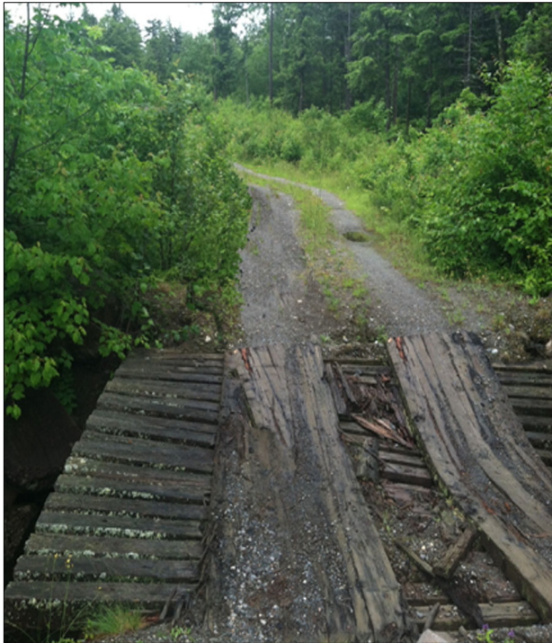
Photo 24. A broken bridge on the access road limits vehicular travel to Punchbowl Pond
