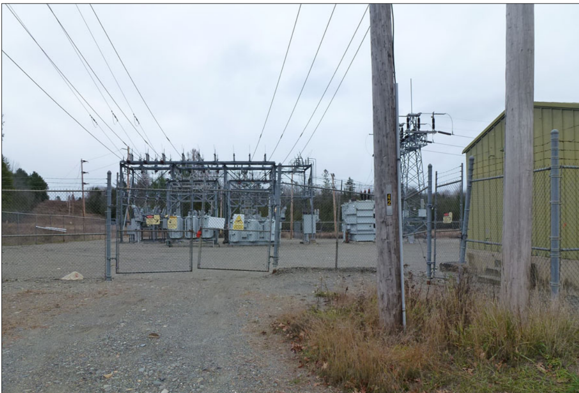
Photo 38. Guilford substation that the generator lead will feed into
