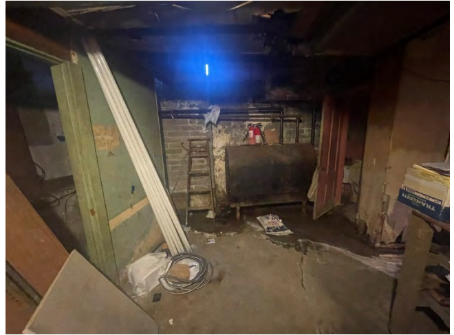
Description: Pawn Shop Basement, Sample AS-2 location
