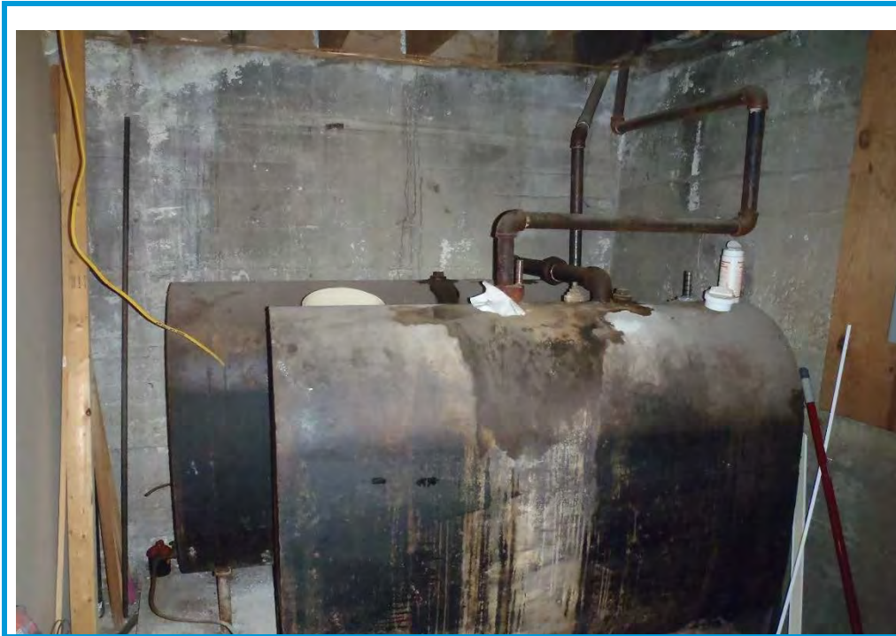
Photo No. 5 Photo Date: June 19, 2019 Site Location: 148 French Street, Bangor, Maine Description: View of the #2 fuel oil ASTs. Photo By: BDS
