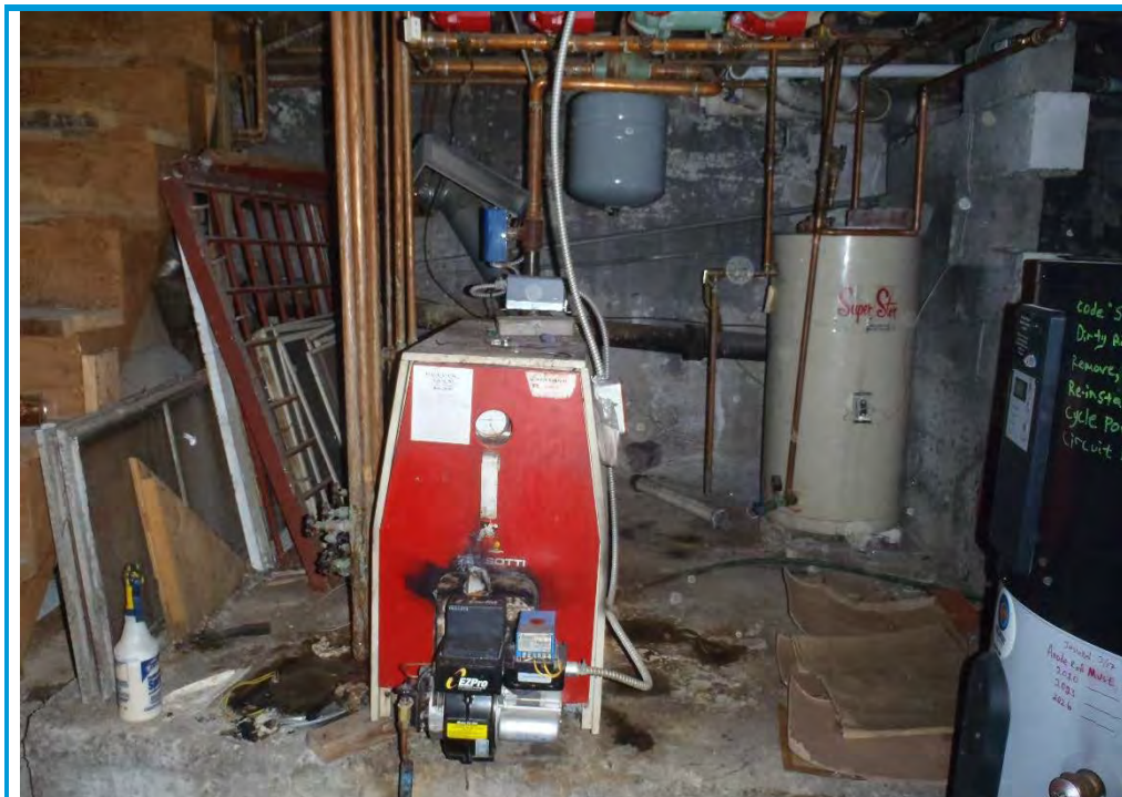
Photo No. 4 Photo Date: June 19, 2019 Site Location: 148 French Street, Bangor, Maine Description: View of the boiler within the structure basement. Photo By: BDS
