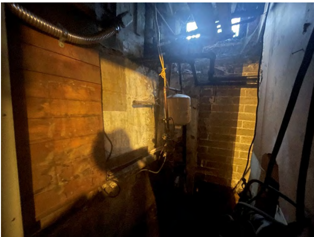
Description: Pawn Shop Basement, water heater
