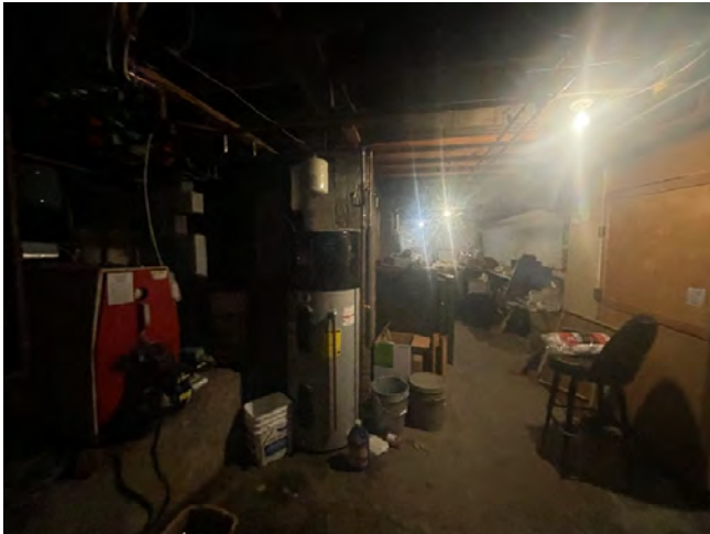
Description: Photo Studio Basement, water heater.
