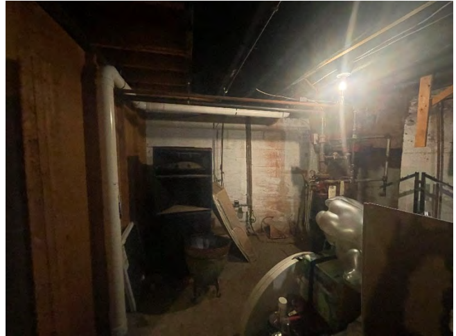
Description: Photo Studio Basement, Vapor Mitigation suction point.
