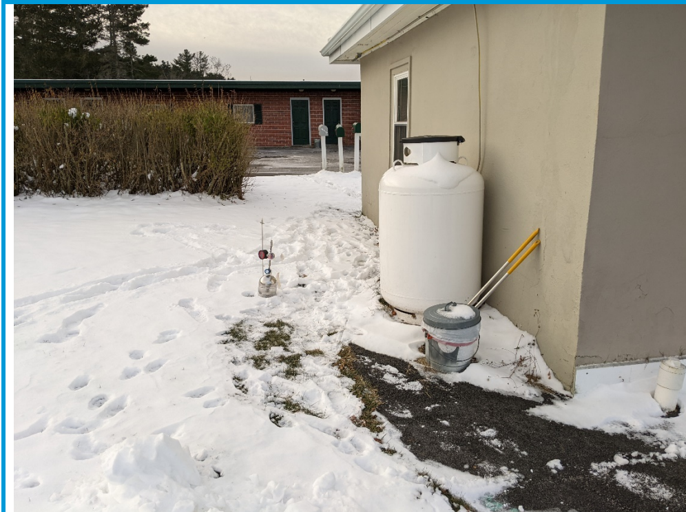
Photo No. 1 Site Location: 211 US Route 1 Falmouth, Maine Photo Date: December 21, 2021 Description: SV-101 to the east of the Lazy Bones building. Photo By: JKC
