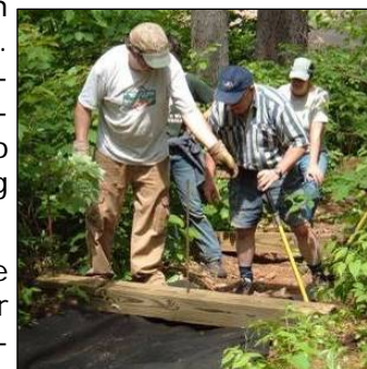
Volunteers build infiltration steps and spread mulch on an eroded path to the lake.
