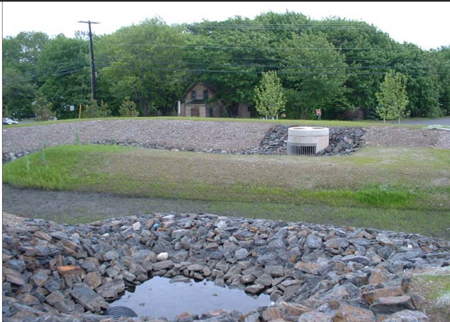
The proper functioning of Stormwater Best Management Practices is critically dependent on regular inspection and maintenance. Learn more about inspection and maintenance of these BMPs and become an inspector by attending this Fall's training sessions. See page 2 to register.
