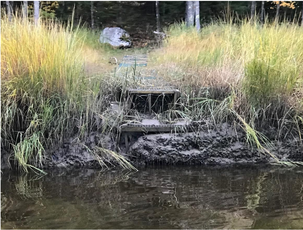
Photo 13: Steve Chef - walkway mowed/cut through saltmarsh (permanent structure laid into marsh grass as walkway & steps) - commenter, likely unpermitted
