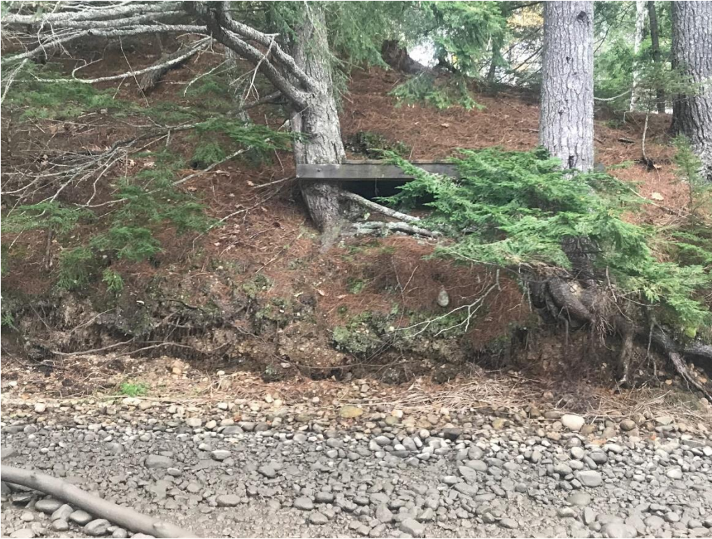
Photo 36: Bolen - unpermitted 'platform' structure adjacent to wetland
