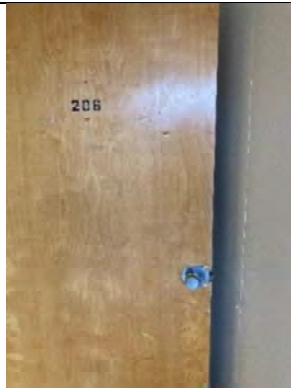
Non-compliant door hardware.
