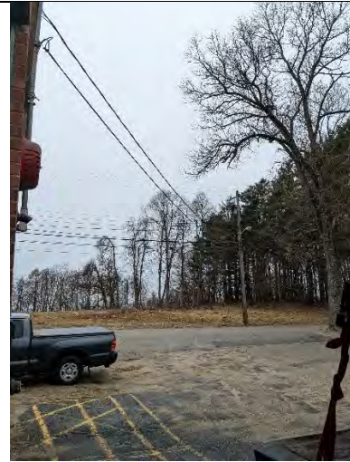
Incoming Overhead Power
