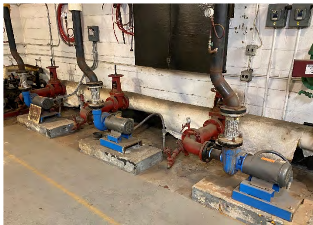
Figure 7 - Main Heating Pumps
