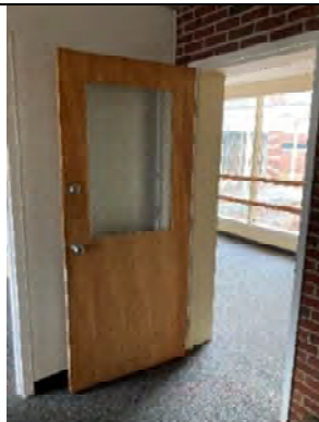
Non-compliant door hardware.
