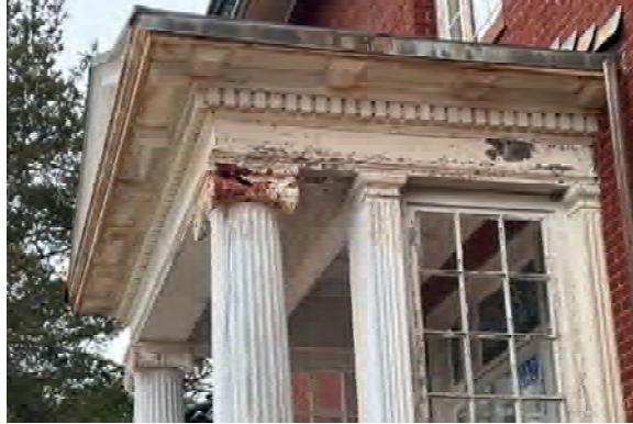
Wood deterioration near door A2
