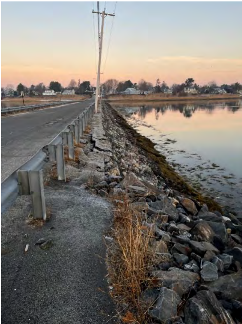
Fig. 11. West Causeway - Northside Armoring in Need of Repair
