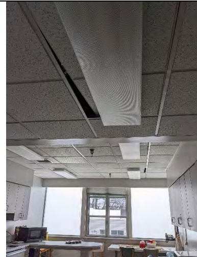
Ex. Space – Needs Daylight/Vacancy Controls
