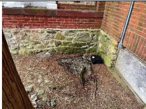
Root infiltration at masonry
