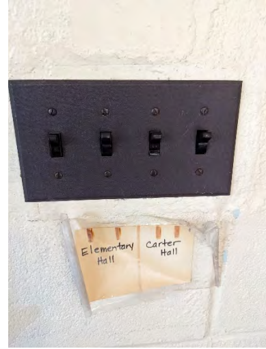
Existing Lighting Controls
