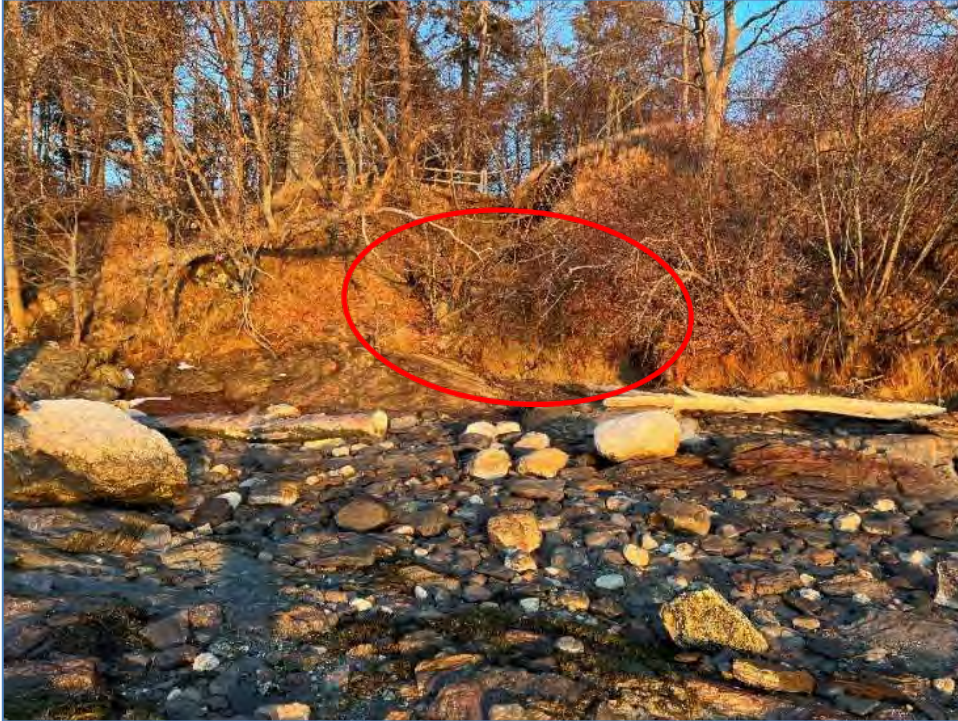
Fig. 16. Pocket Erosion in the Area where the Embankment Toe is Exposed
