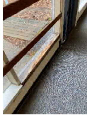
Water damage at sill.
