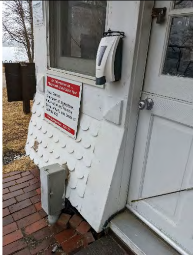
Power Entry to Gatehouse
