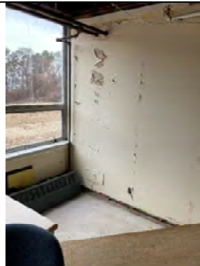
Deterioration at existing partition wall.
