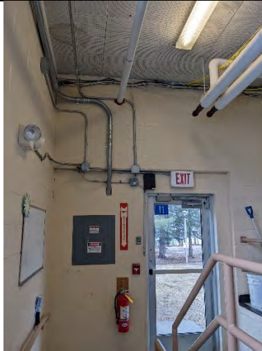
Lights, Elec Pnl, Exit Lights
