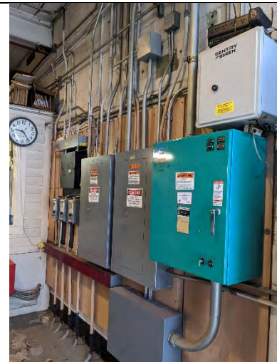
Electrical Panels and Transfer Switch.
