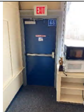
Non-ADA compliant approach at exterior door.
