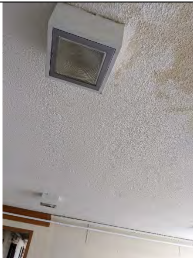
Existing Light Fixtures
