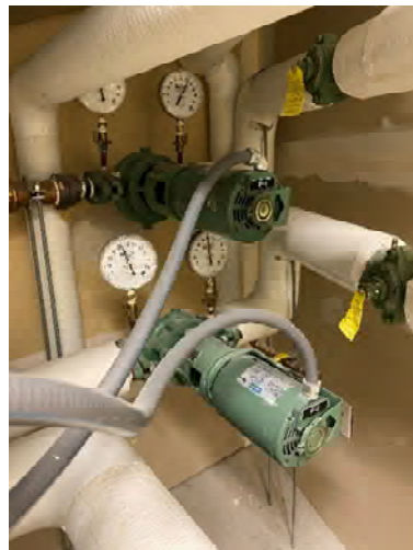
Figure 4 - Radiant Floor Pumps
