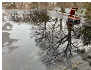
EPDM Roof ponding
