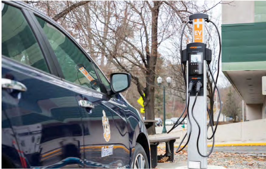
▲ EV chargers at MeDOT powering electric vehicle fleet.
