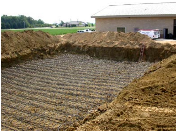
Source: Capital Electric Cooperative, n.d.
