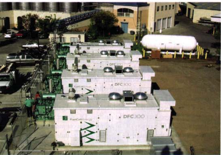
■ The installation of four DFC300 high temperature, high-efficiency carbonate fuel cells provide the brewery virtually all of its baseload electrical power. >> Photo courtesy of Sierra Nevada.
