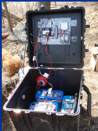
-> Powers 12V Batteries
