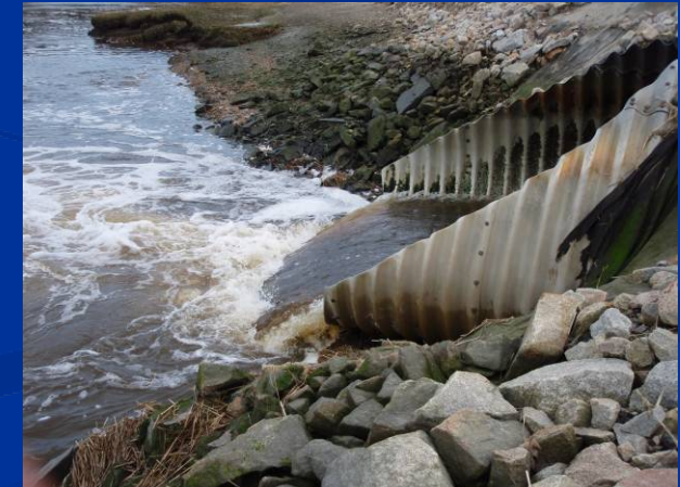
Hanging Culvert, Cascade Brook, ME
