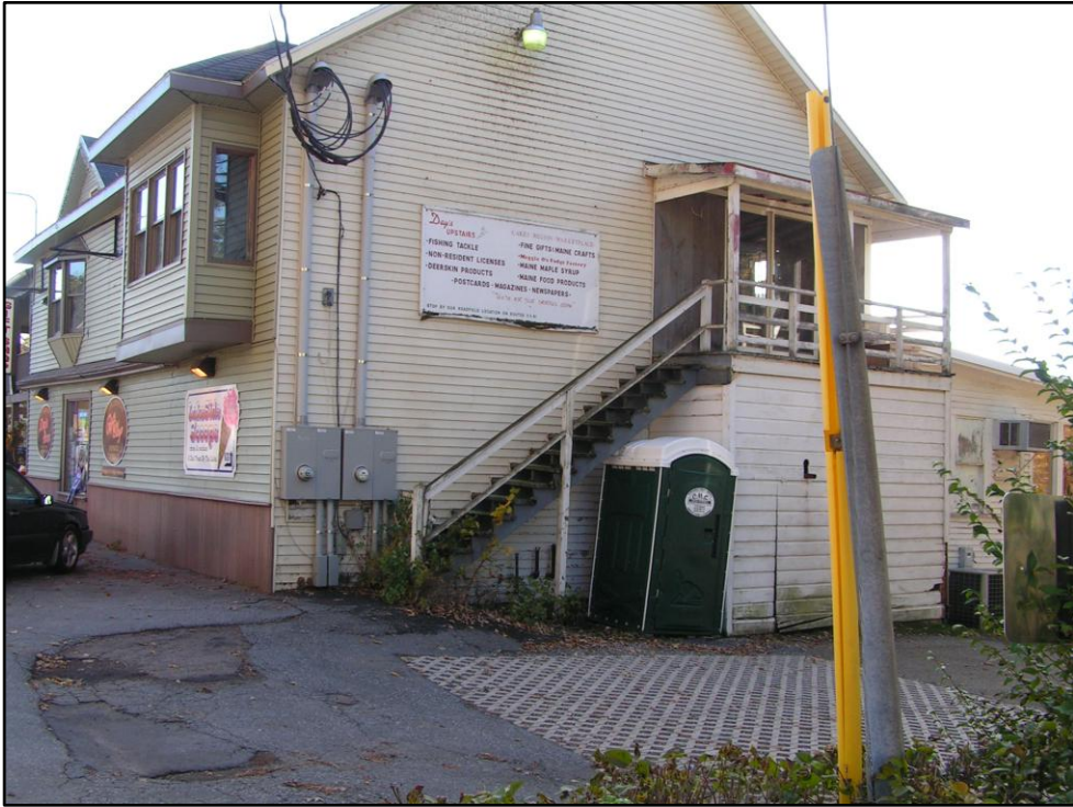
Here is another view of porous pavers at Day's Store in Belgrade.
