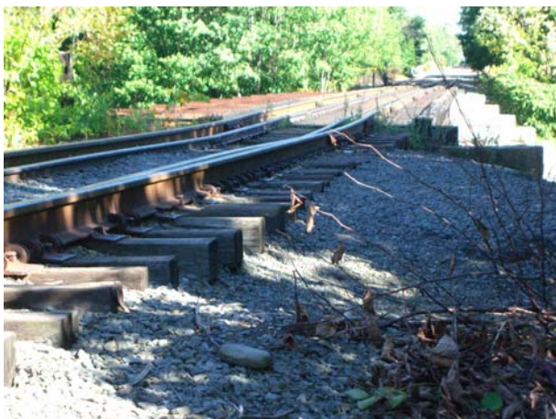
Figure 3-5- Settlement at west abutment
