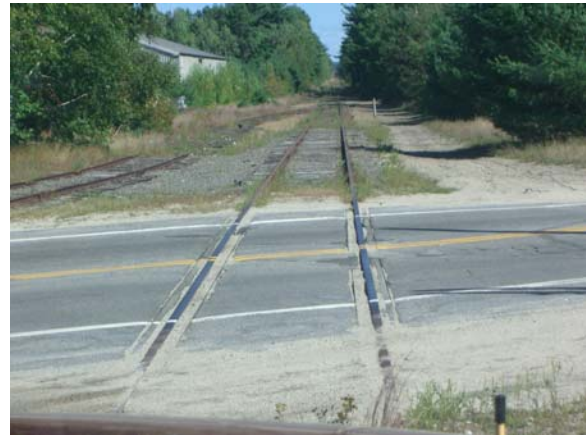
Figure 2-15 – Typical major crossing with Nelson Chair Rails installed
