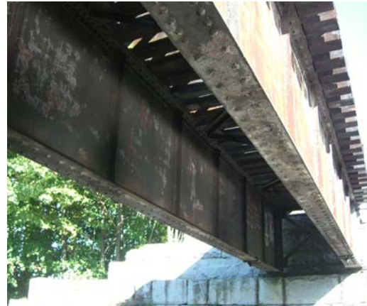
Figure 3-4 -Presumpscot River, East approach deck girder span. West approach the same. Note lack of intermediate diaphragms and cross bracing.
