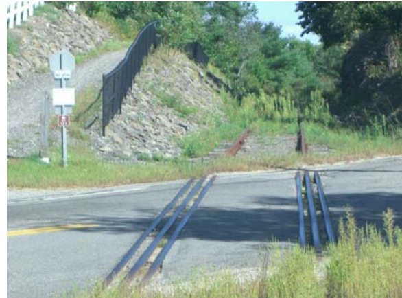
Figure 2-2 – Slope for rail trail above filled in ditch along the railroad. Water now flows between rails during heavy rains.
