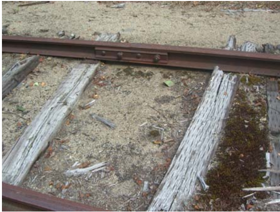
Figure 2-7 – Large gap (spacing) resulting from bunched and skewed ties
