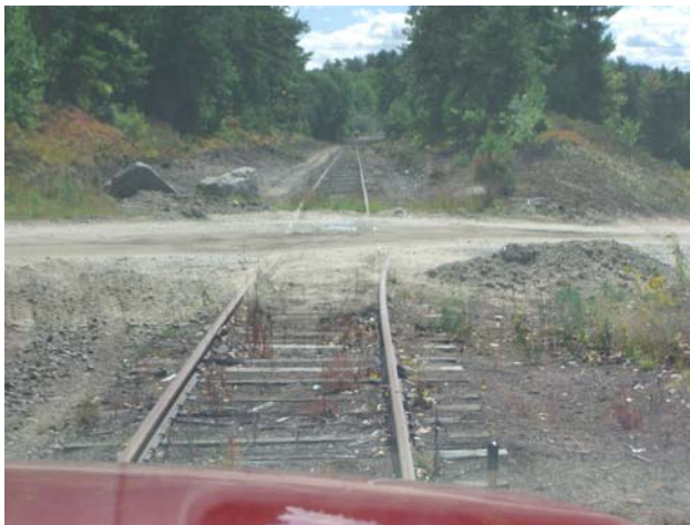
Figure 2-9 – Note the broken rail on right side of crossing and depressed surface.
