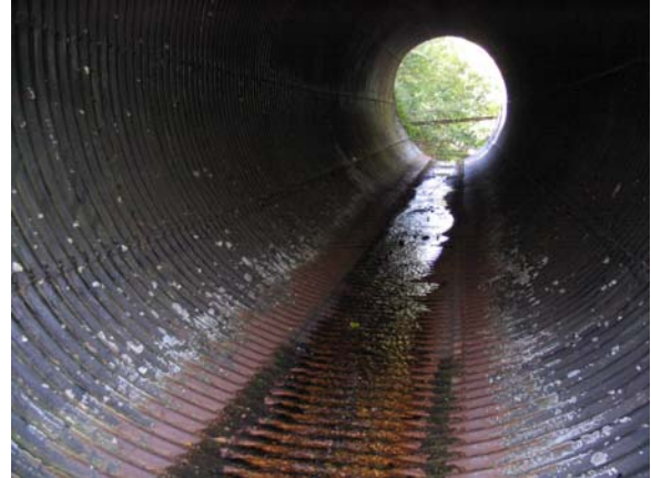
Figure 3-48 – Interior of pipe culvert showing corrosion along invert
