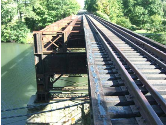
Figure 3-1 - Presumpscot River, Looking east Note provision for second track on main truss span but not on approach span
