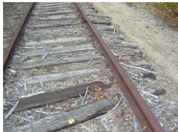
Figure 2-6 – Bunched Ties (Note overall poor tie condition)
