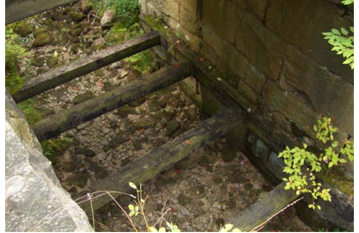
Figure 3-26 – Timber struts between abutments
