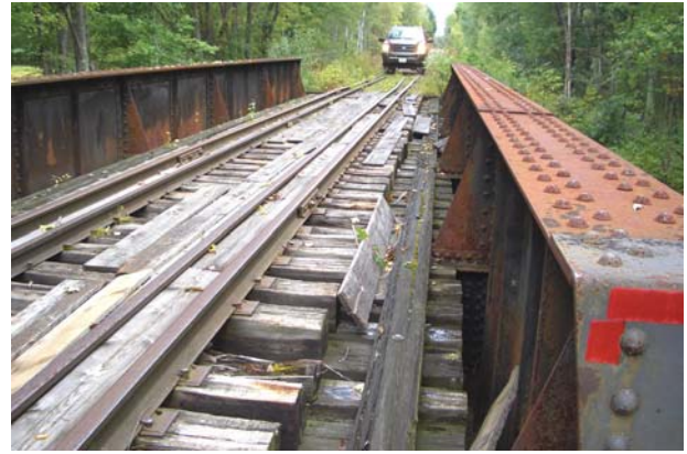
Figure 3-34 – Bridge deck and through girders. Note additional set of timbers on top of main girders.
