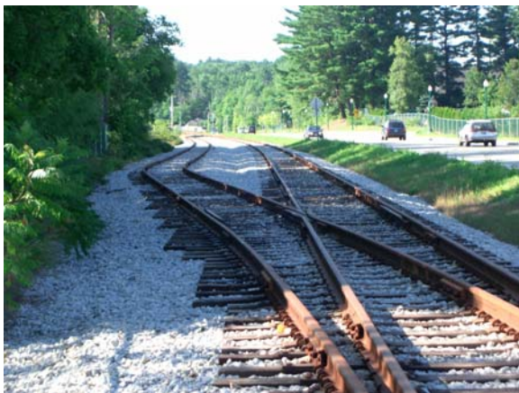
Figure 2-12 – Segment of Reconstructed Railroad in North Conway showing new runaround track, portion of turnout.
