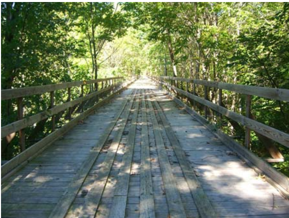
Figure 3-39 – Looking west from east end of bridge. Note that entire deck has been planked over for snow mobile use and railings installed
