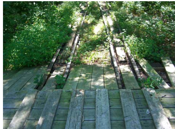
Figure 3-40 – Detail at end of bridge where decking has been installed up over both running and guard rails
