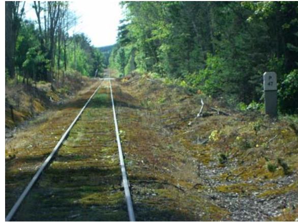
Figure 2-8 – Moss covered roadbed and ties
