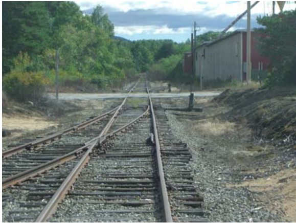
Figure 2-11 – Typical 85 Lb RBM Frog Turnout, Fryeburg, ME
