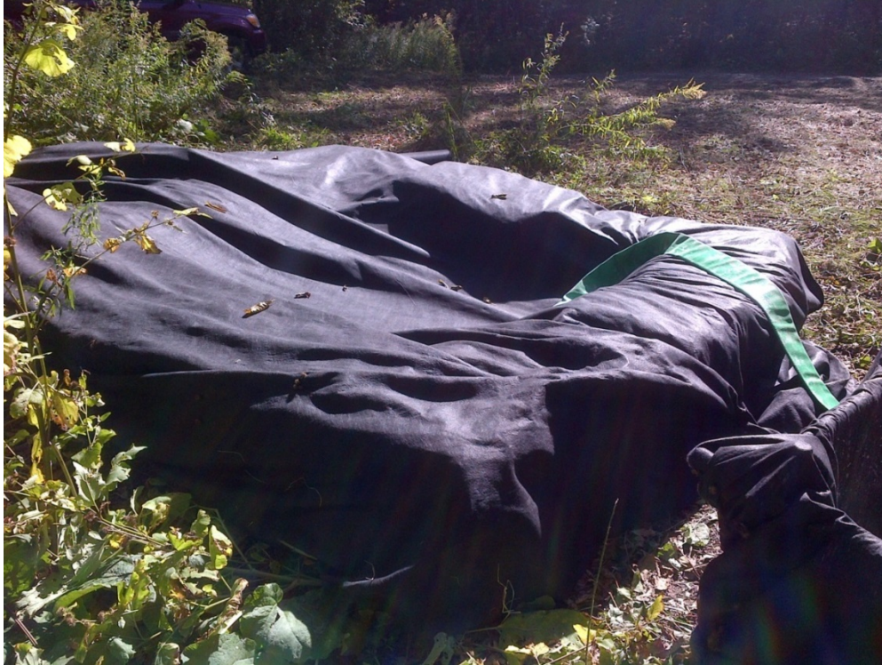
Figure 3-14. Hay bales and geotextile fabric used as part of a dirty water treatment system.
