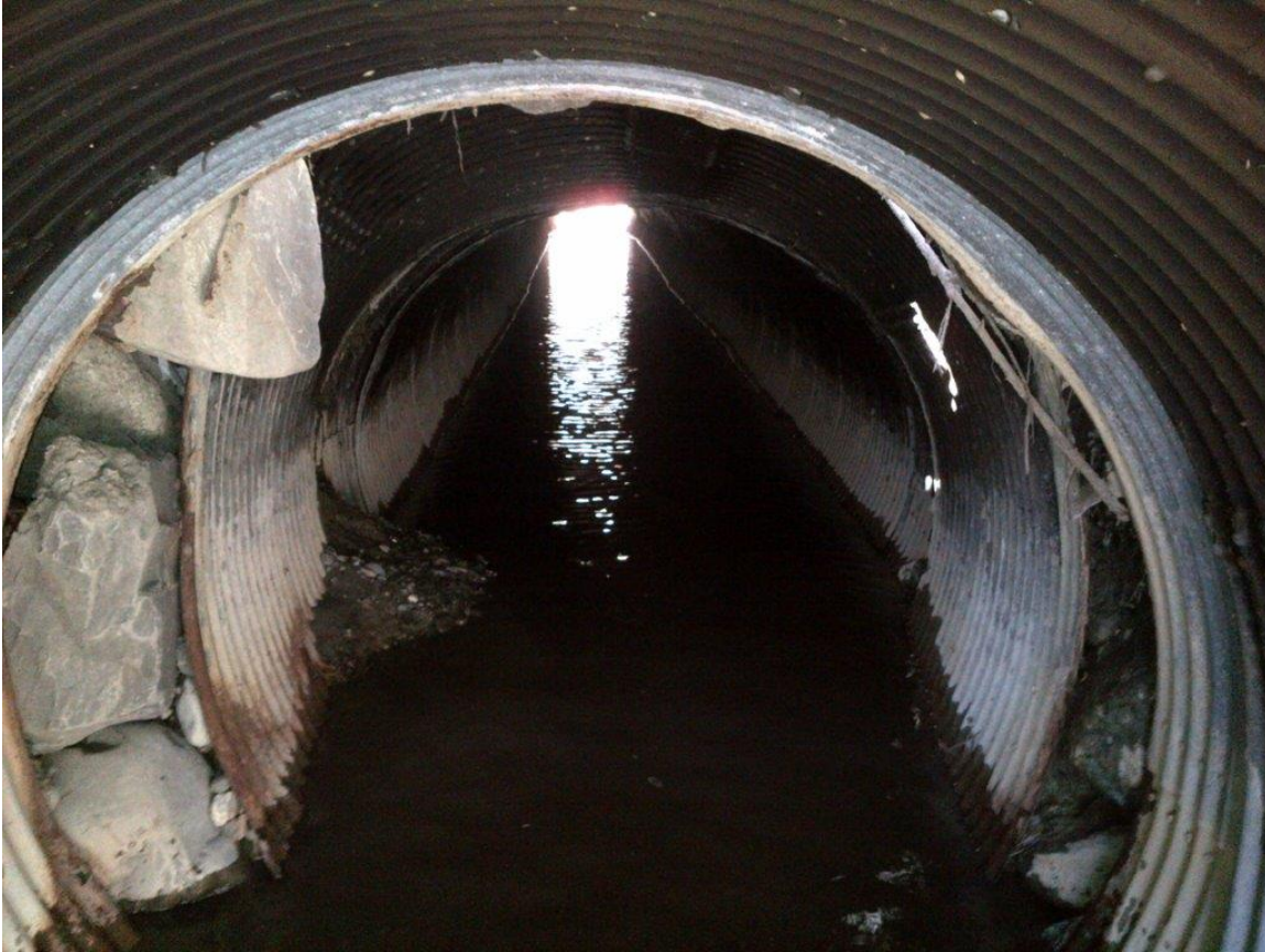
Figure 3-27. View of a culvert where the end has become separated.
