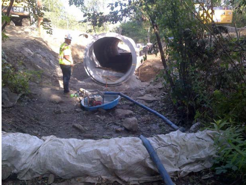
Figure 3-13. A dewatered work area with a small pump to maintain the dry work area.
