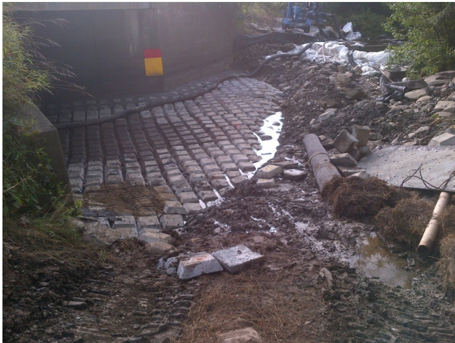
Figure 3-31. Concrete cable mats “toed in” on the upstream edge of a bridge.
