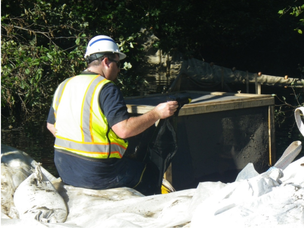
Figure 3-15. Box and screening used as a pump intake screen.
