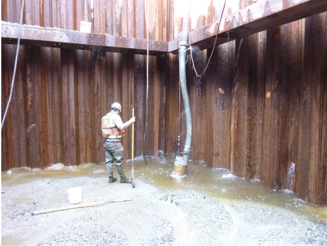
Figure 3-24. After excavating the substrate, concrete is poured across the entire bottom inside of the sheet pile cofferdam to create a “dry” work area for constructing the pier. A maintenance pump is still necessary for maintaining the “dry” conditions.
