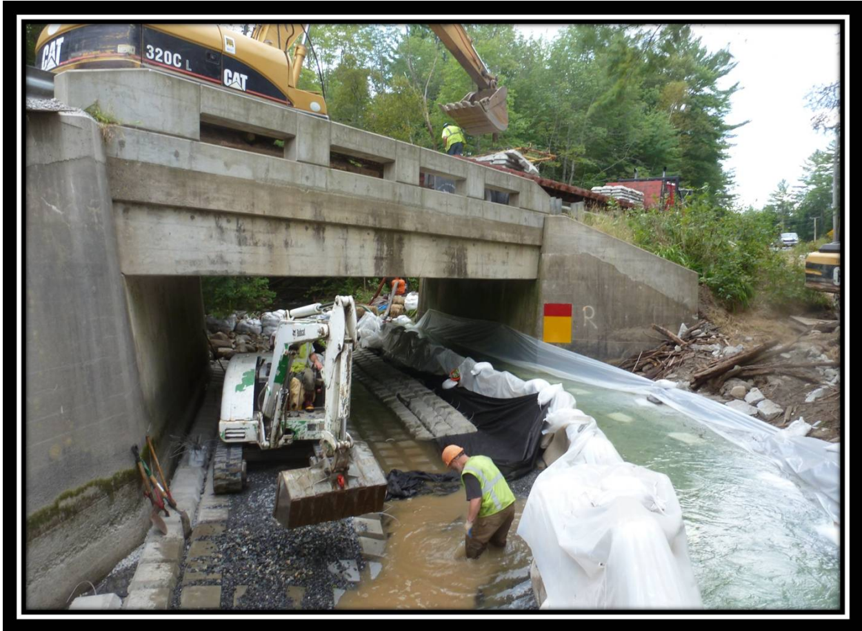
Figure 3-30. Concrete cable mat installation. A migratory pathway will be maintained throughout the construction process in situations where stream width will allow.
