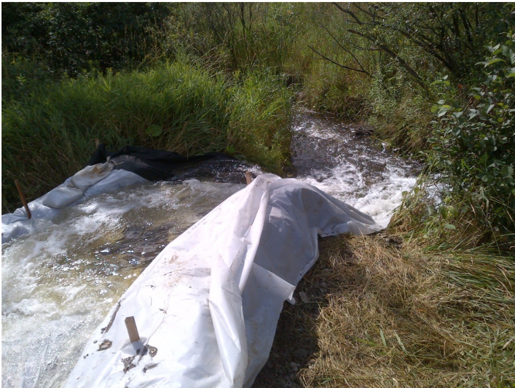
Figure 3-16. Plastic sheeting and hay bales can be used for a pump outlet or outlet of a bypass channel.
