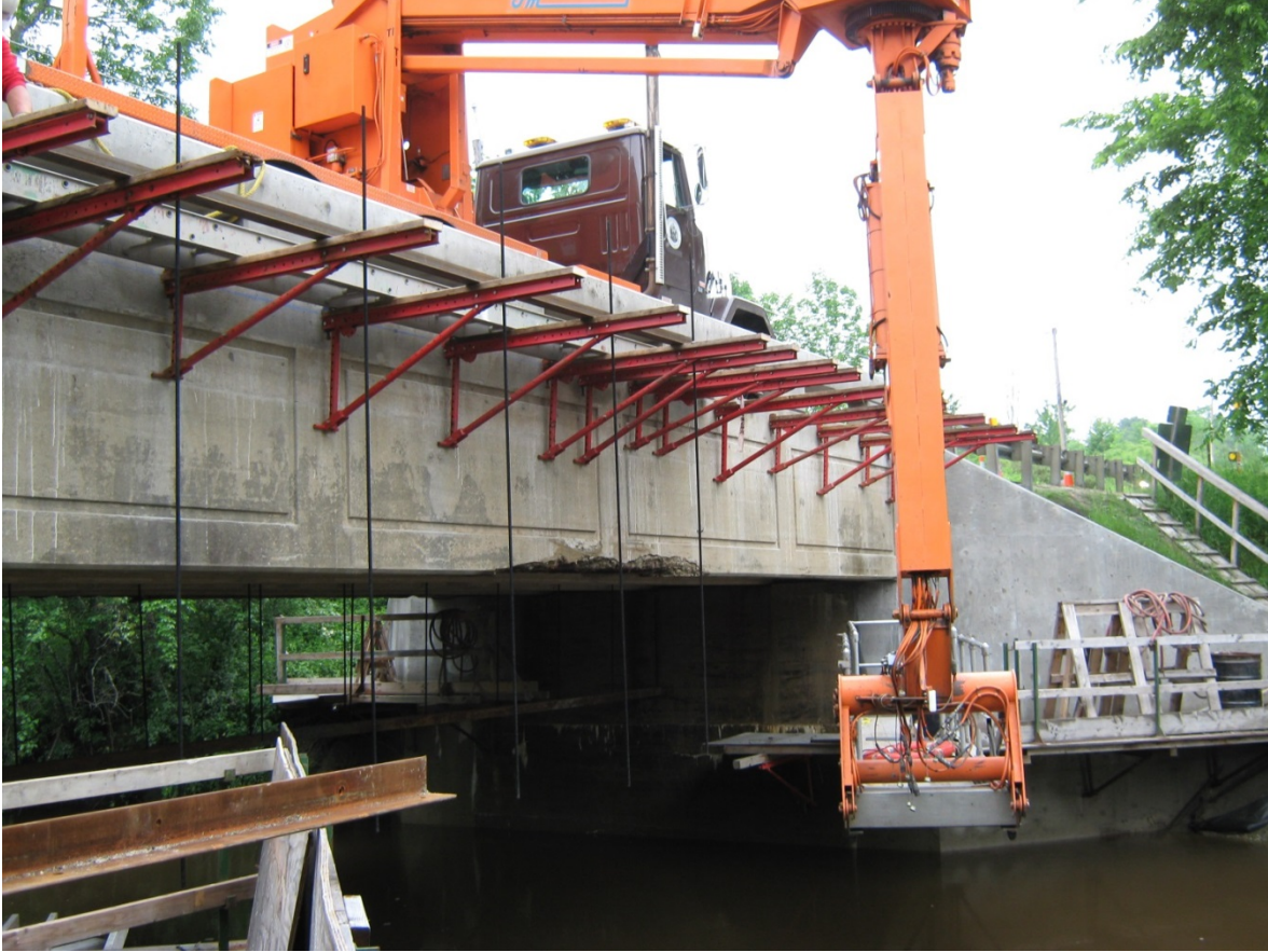
Figure 3-34. Concrete repairs on beams will be completed from staging. In this photo, the staging is attached to the wing wall.
