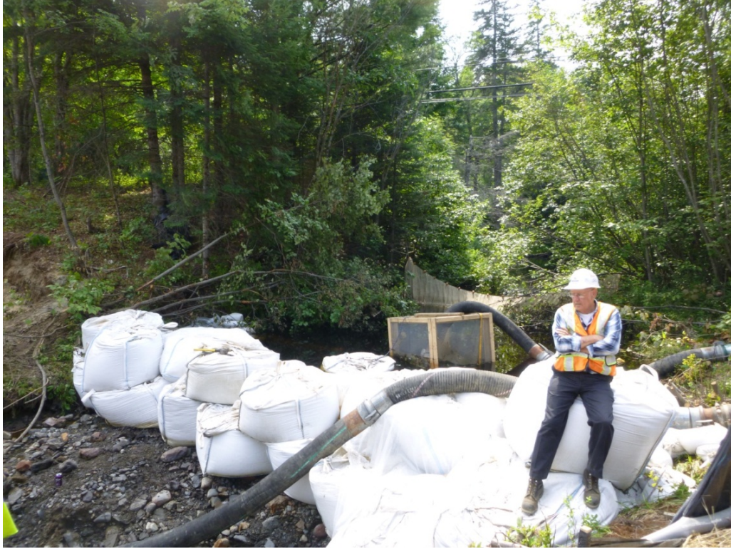
Figure 3-2. Cofferdam made of industrial sandbags. Bypass pump intake upstream of the cofferdam.
