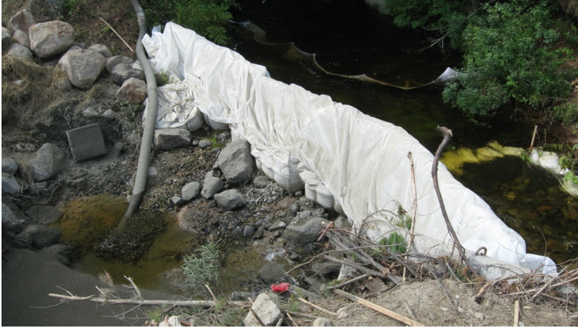
Figure 3-6. Cofferdam made of sandbags and jersey barriers draped with plastic sheeting. Pump intake in the photo is maintaining water levels in the work area.
