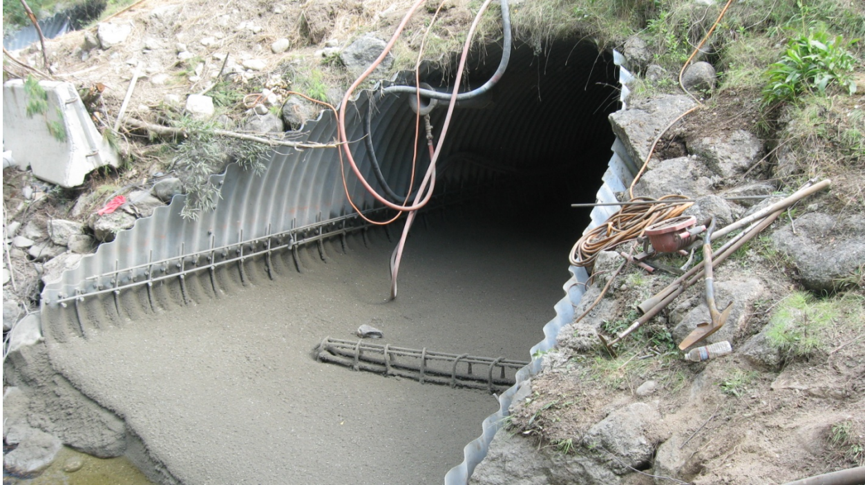
Figure 3-37. Concrete freshly placed during an invert lining. Note the rebar cage for fish weir support.
