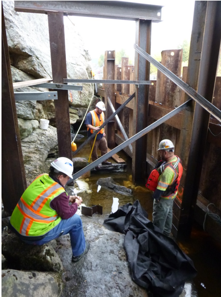
Figure 3-22. Example of the inside of a sheet pile cofferdam used for abutment construction on a bridge replacement project.
