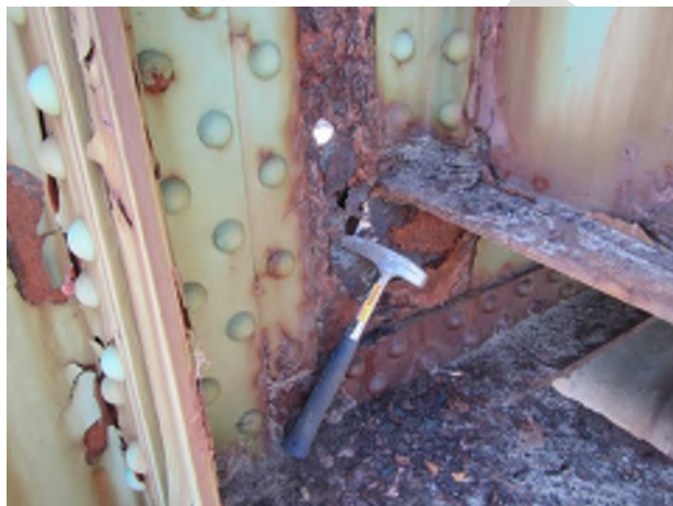
Figure 8: Hole in floorbeam
