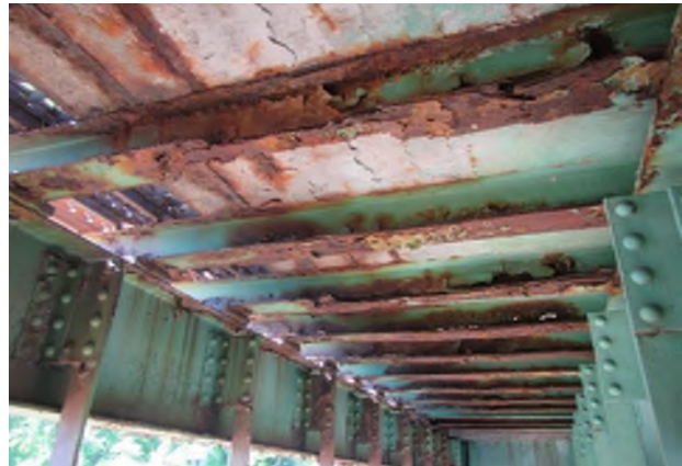
Figure 7: Deteriorated cross beams & deck
