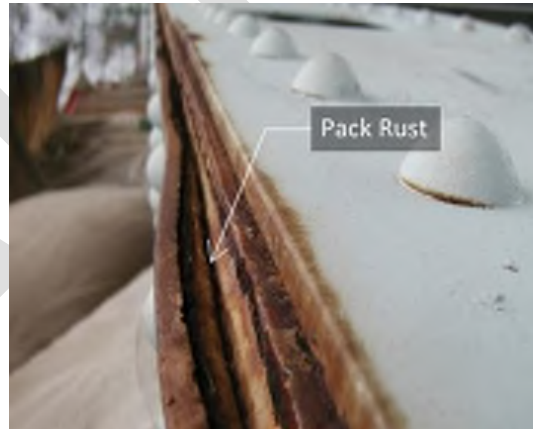
Figure 14: Pack rust is corrosion in the crevice between two plates of steel that are bolted or riveted together. As the rust progresses, it gradually pushes the pieces of steel apart, bending them and sometimes breaking bolts or rivets. The only way to truly fix pack rust is to take apart the plates of steel and clean them, which is usually not feasible.
