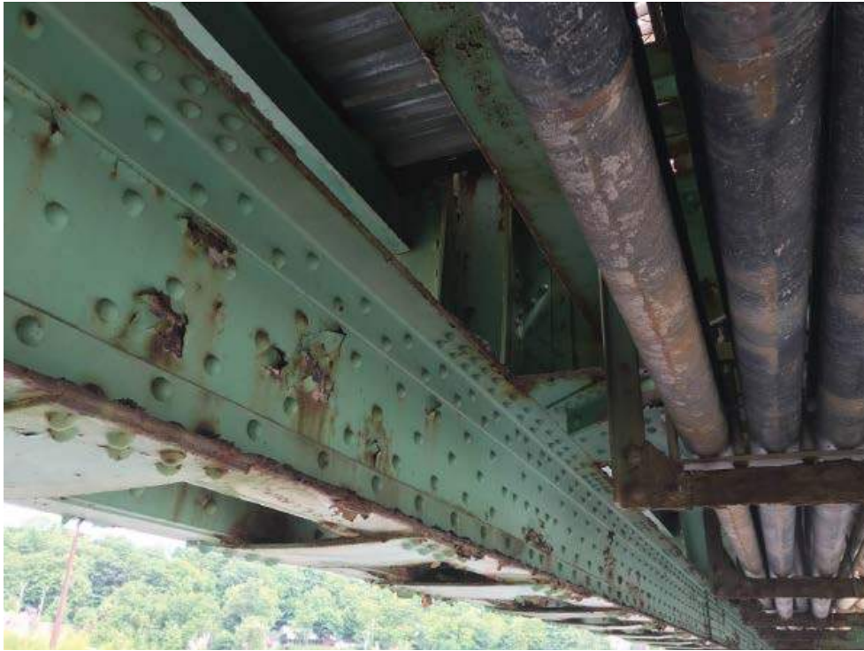
Photo # 9: General view of paint loss and corrosion to bays below the open grid decking in the travel way shoulders on the sidewalk side (western) of the bridge (8/1/16)
