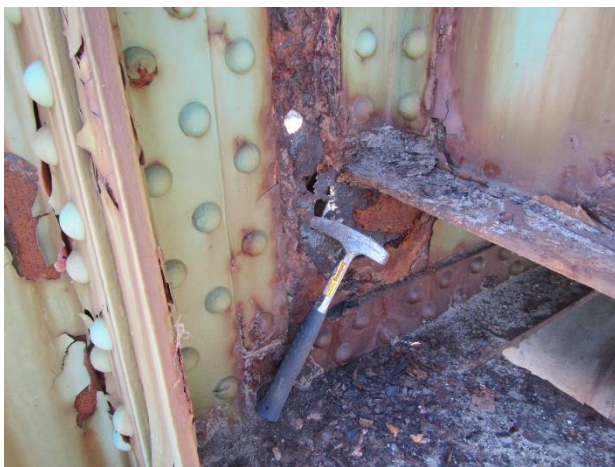
Figure 9: Hole in floor beam
