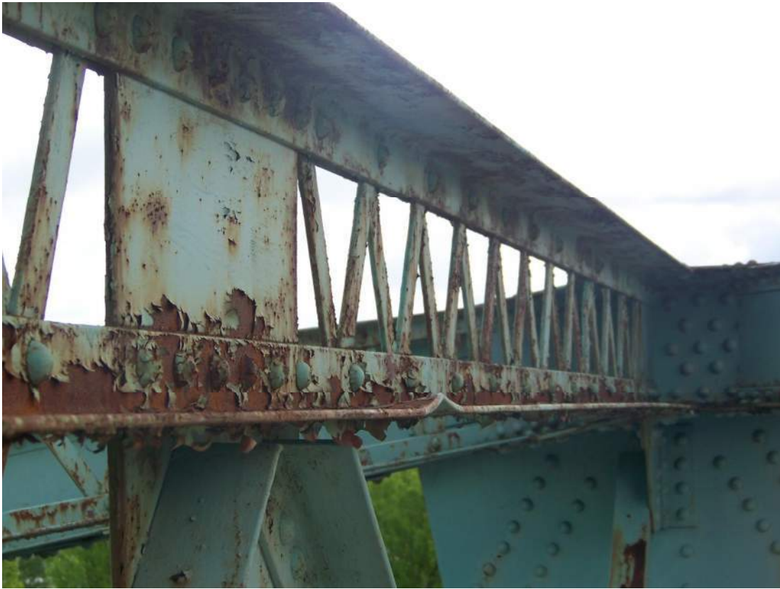
Photo 69 – The Span 3 U5 upper chord lateral bracing transverse top strut has a \frac{3}{4} inch upward bend in the south side lower angle edge at one foot east of roadway centerline.
