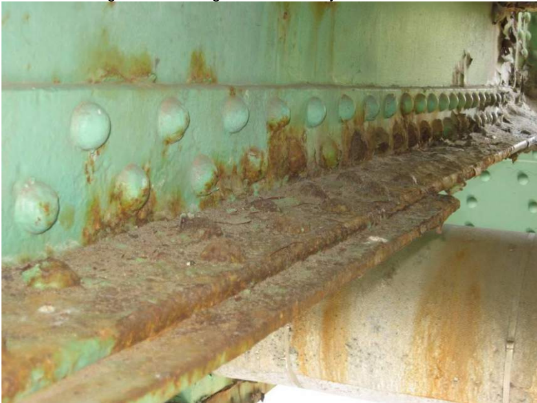
Photo 42 – Span 1 FB3 has moderate active corrosion to the bottom flange on the south side of the web between S6 and S8. View looking east.
