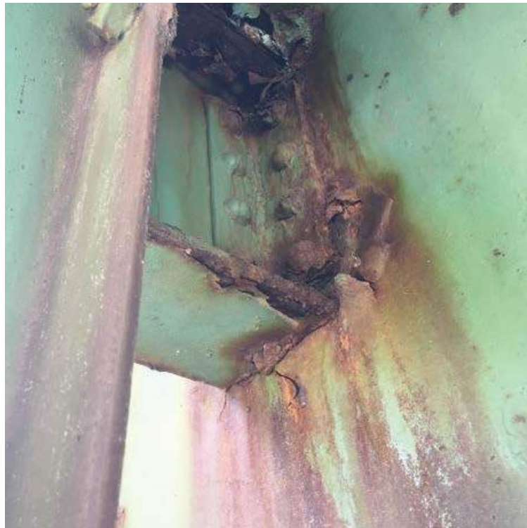
Photo #28: Moderate corrosion with pack rust between the connection angles and floor beam, at S8 in span 3 near FB5 (8/2/16)
