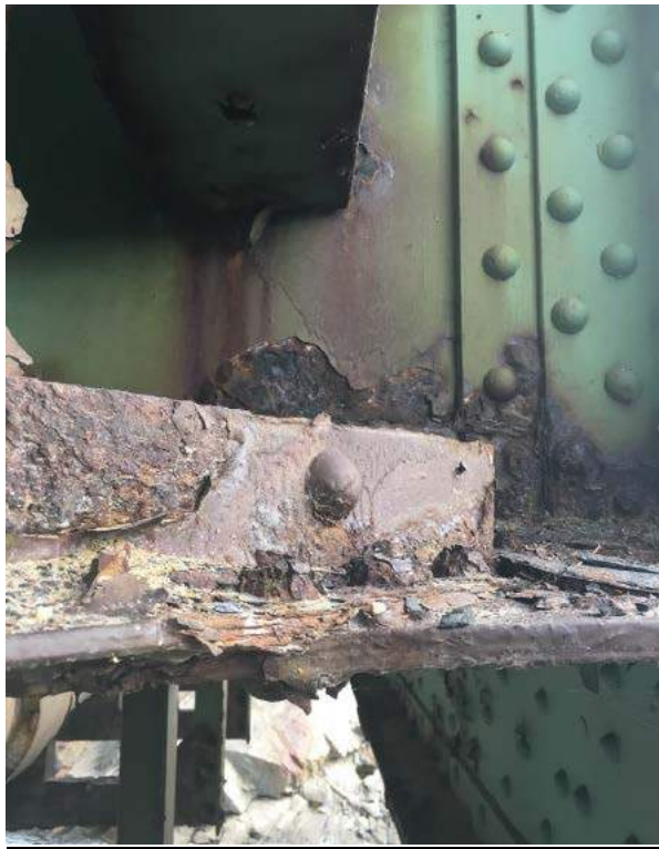
Photo #54: Corroded lateral bracing end at its connection to the horizontal plate at FB8 span 2 (8/2/16)
