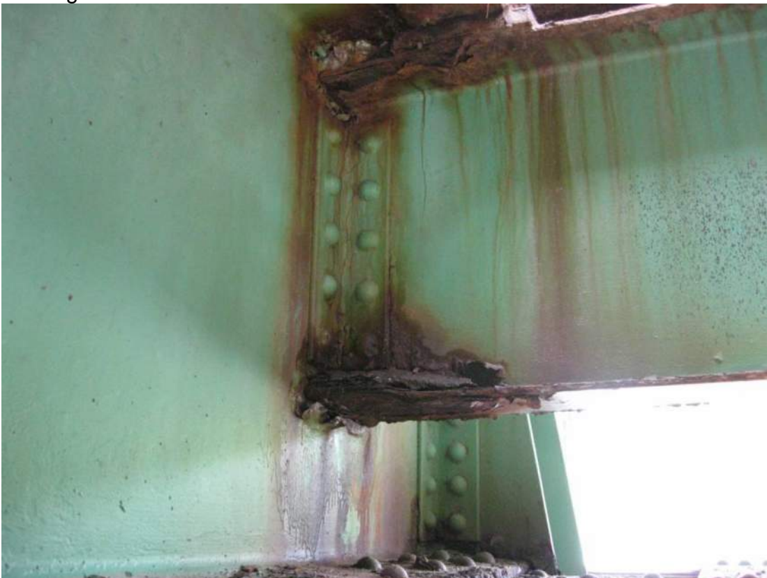
Photo 56 – Stringer S3 has pack rust on bottom flange and bottom of web at connection to north face of Span 3 FB3. Similar conditions noted at three other S3 stringer ends.
