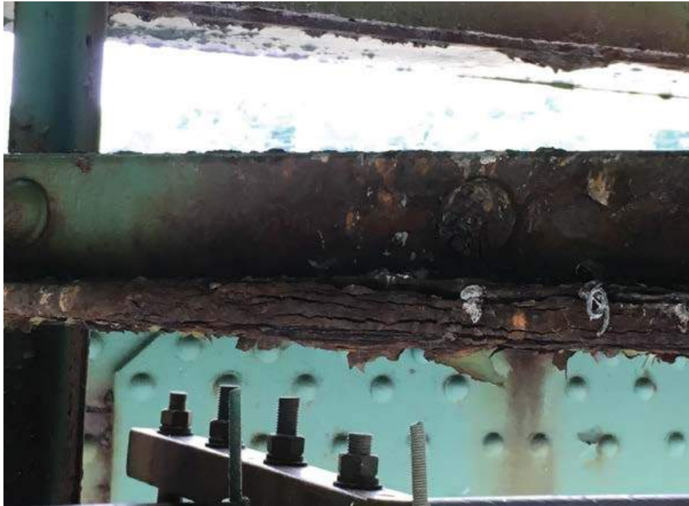
Photo #55: Pack rust and section loss to the lateral bracing near FB6 in span 1 (8/1/16)
