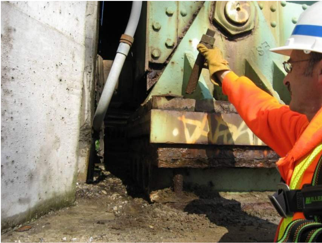
Photo 73 – The roadway truss bearing at the south abutment has a loose anchor bolt which was removed, photographed and loosely re-inserted by the inspection crew.
