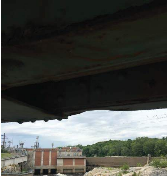
Photo #41: “Dent” to the exterior member making up the bottom chord on the sidewalk (western) truss at the same location of the previous photo (8/1/16)
