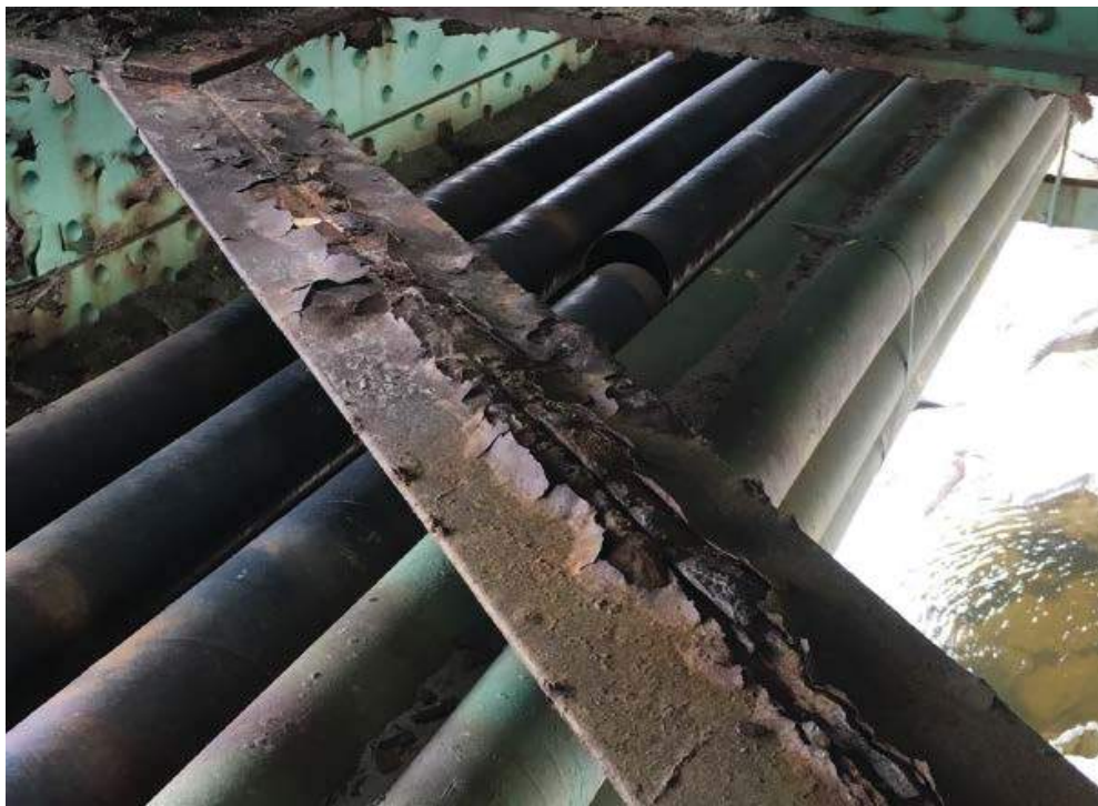
Photo #50: Severely corroded lateral bracing member view from top of double angle in spans 1 & 2 (8/1/12)
