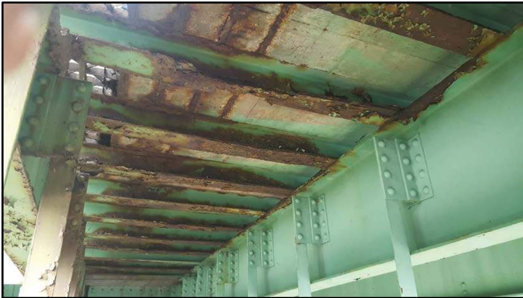
Photo A21 – View showing Needle Beams between Stringers 7 and 8. Area between stringers 3 and 4 are similar.
