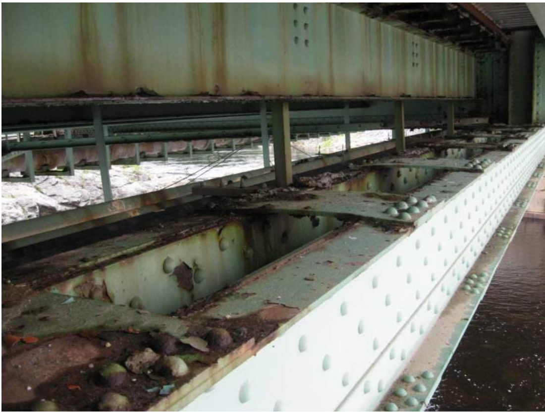
Photo 29 – Top face tie plates are similarly bowed in the upward direction due to pack rust at the interfaces with the top of the lower chord side channels.
