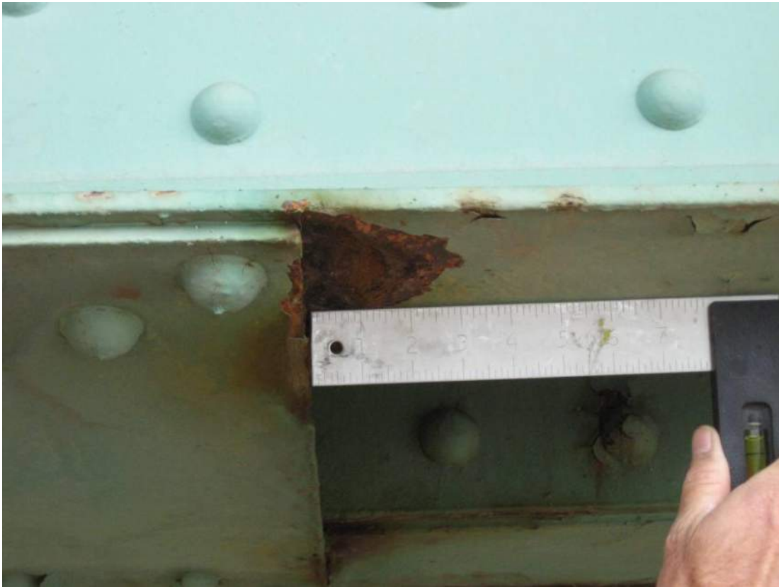
Photo 31 – Zone of 1/8 inch deep by 3 inch wide section loss to Span 3 L4-L5 sidewalk truss outboard side channel located at corner of first tie plate south of center splice.
