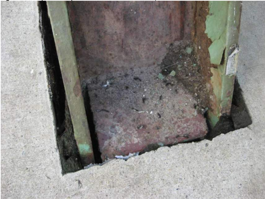
Photo 38 – Sidewalk truss verticals and diagonals have welded plates at sidewalk level openings. These plates represent FSD's in FCM's (wherever base members are FCM's).
