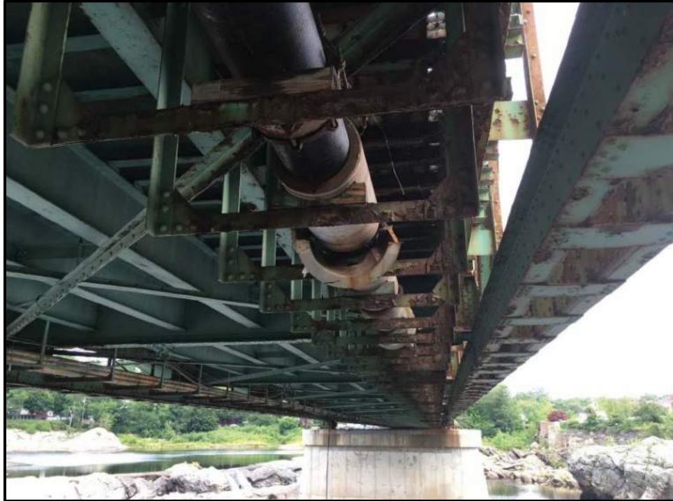
Photo A23 – View of steel insulated utility pipe extending across the bridge on the Roadside Truss side.
