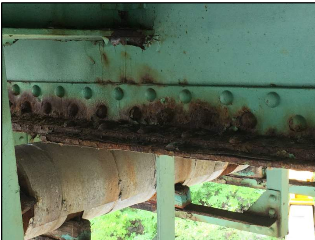
Photo A4 – Floorbeam 2 coverplate particularly between Stringer 7 & 6 is an area of concern which will be closely monitored.
