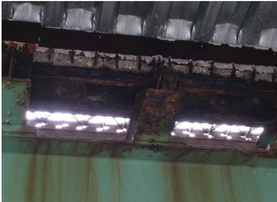
Photo #46: Severe corrosion to a cross beam (needle beam) on the sidewalk (western) truss (8/1/16)
