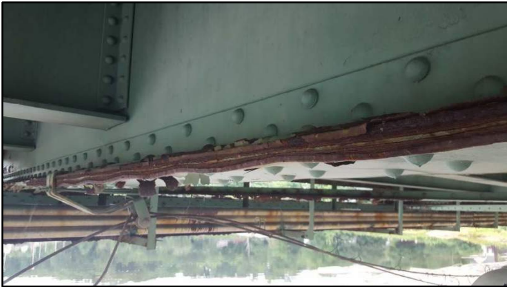
Photo A7 – Floorbeam 8 bottom flange midspan plies showing pack rust and deformation which may lead to repair activity within the next 5 years.
