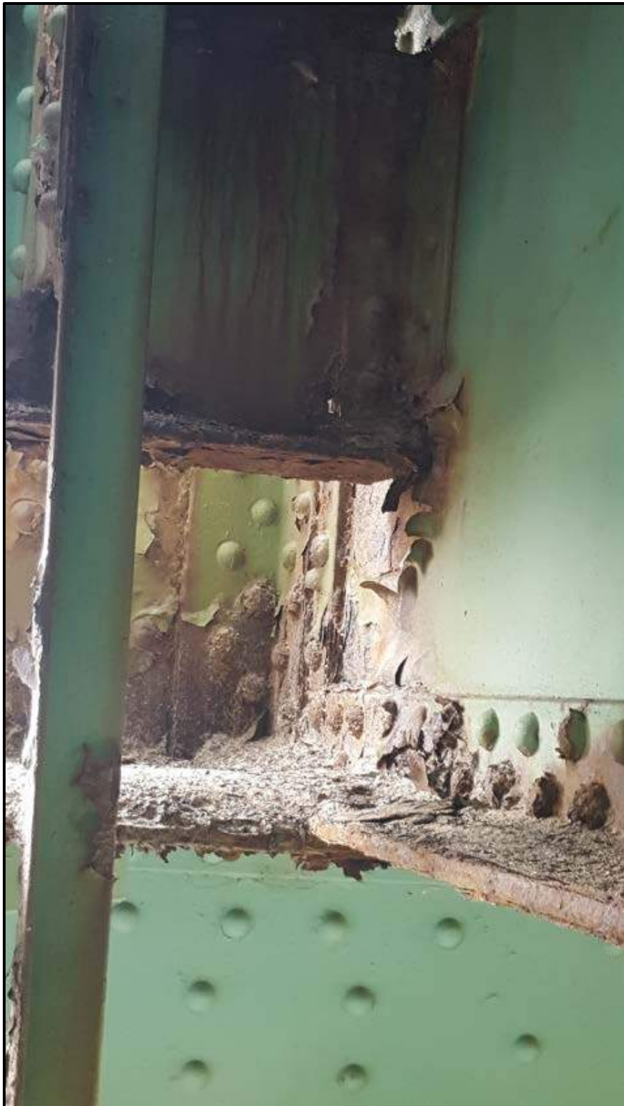
Photo A12 – Stringer 8, Roadway Truss @ Floorbeam 2 has section loss revealing a web hole.
