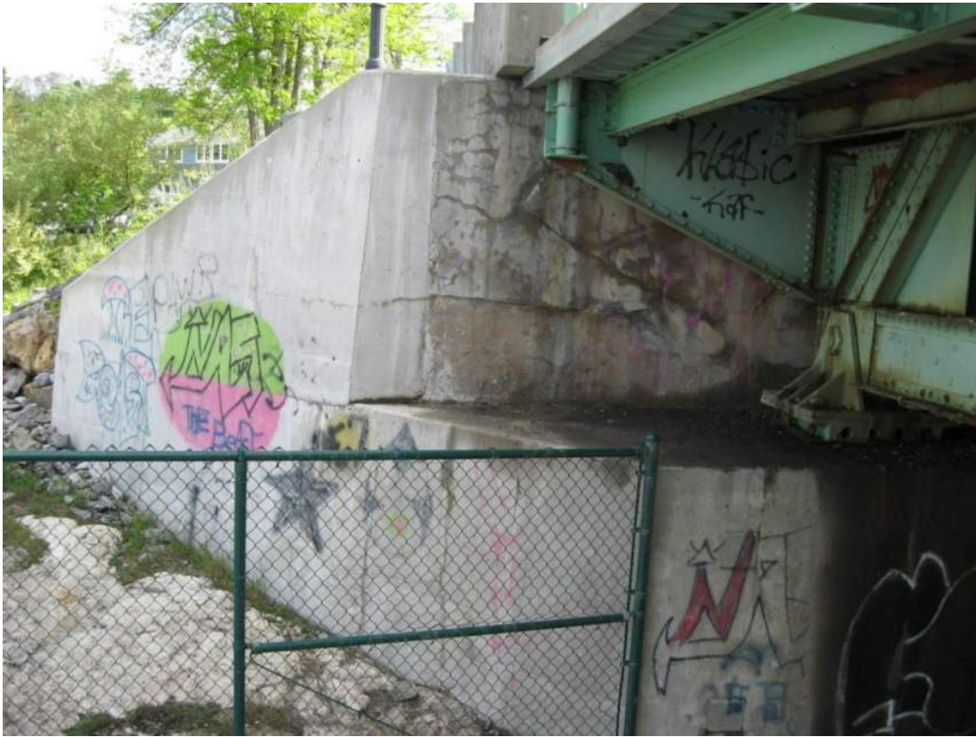
Photo 79 – The north abutment backwall has numerous medium diagonal cracks in the portion below the sidewalk. View looking north along sidewalk truss.
