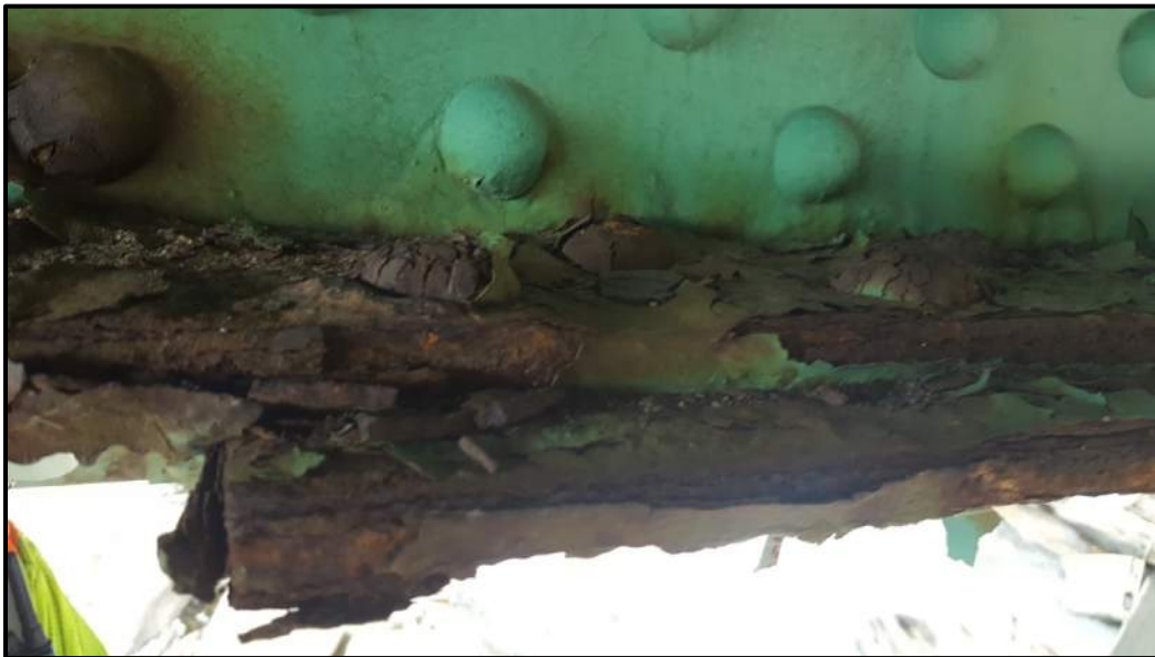
Photo A6 – Floorbeam 6 exhibiting excessive pack rust and rivet deterioration.
