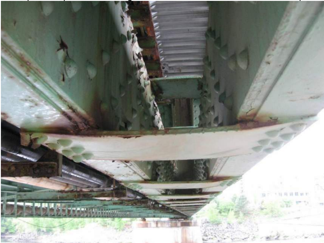
Photo 28 – Span 2 sidewalk truss lower chord bottom face tie plates bowed downward due to pack rust at the interfaces with the bottom of the lower chord side channels.
