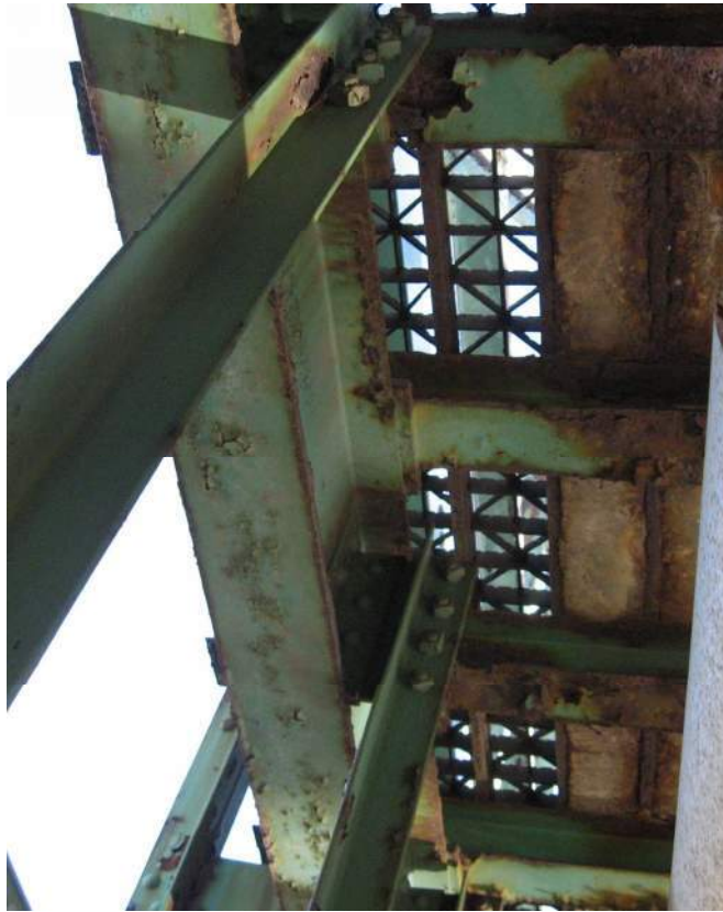
Photo 63 – Perforations at the flange edges and in the bottom flange of the cross-beams was observed in Span 3 near L6 in the ends of the cross beams.
