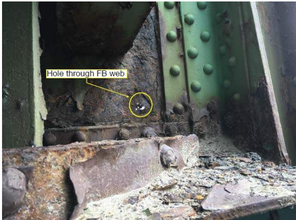
Photo # 14: General view of corrosion and hole through the web of the non-sidewalk (eastern) end of FB5 in span 1 (8/1/16)
