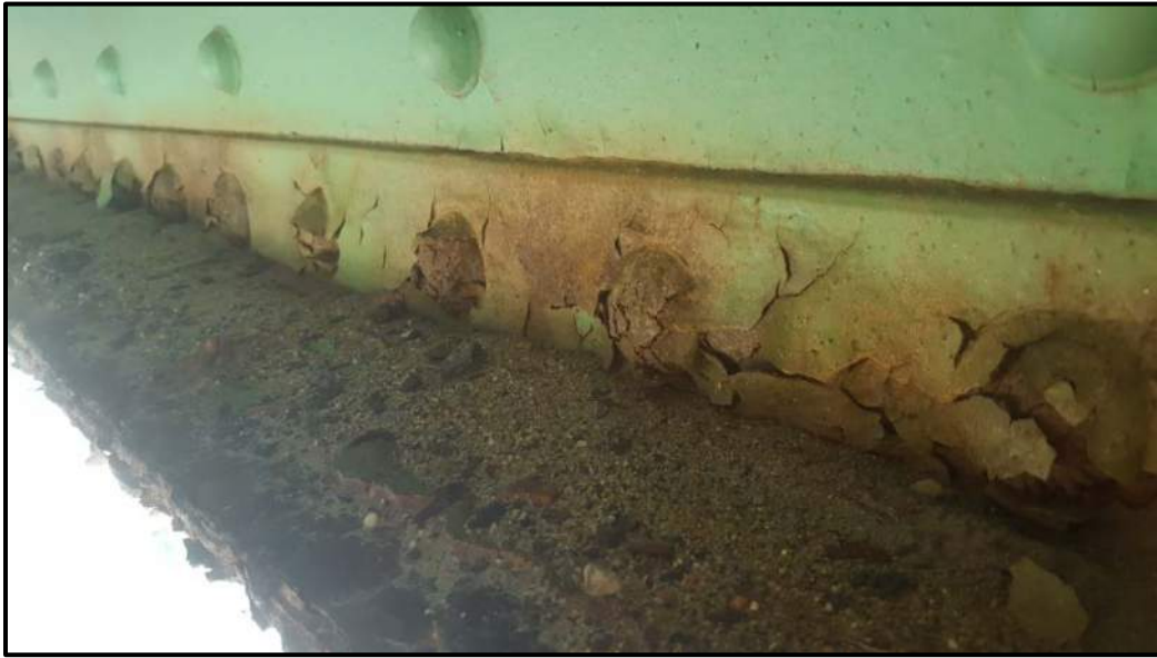
Photo A8 - View of the inside of Sidewalk Truss's lower angle depicts continuous corroding rivet heads and sand, salts and debris occupying the angle flange.
