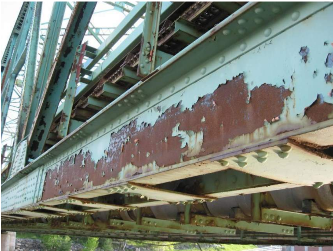
Photo 25 – The east face of the Span 1 roadway truss between L8 and L9 exhibits missing paint and active corrosion over a 15 foot length.
