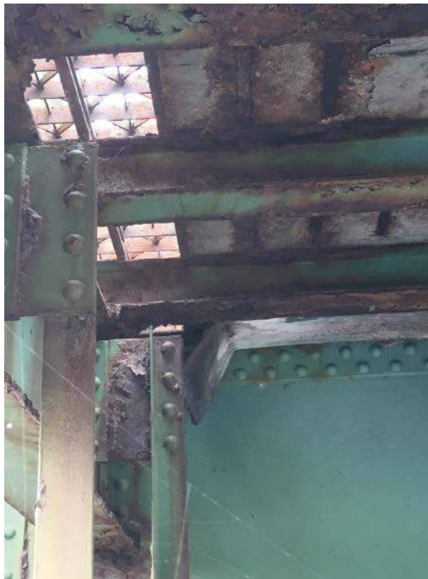
Photo #44: Moderate corrosion to cross beams (needle beam) (Typ.) (8/1/16)
