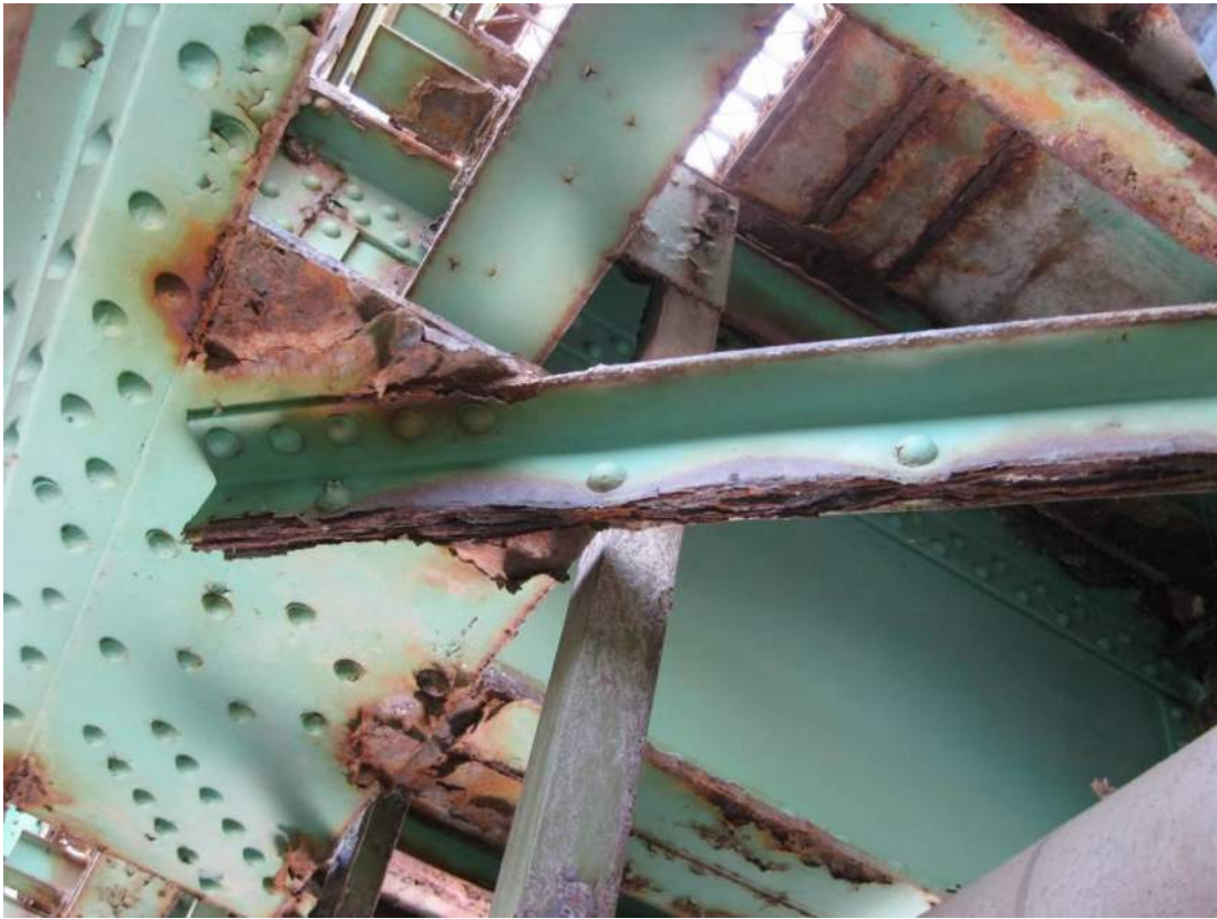
Photo 71 – Severe pack rust with active corrosion over a 4' length of lower lateral bracing angle connecting Span 1 L3 roadway truss and L4 sidewalk truss at the L3 end.
