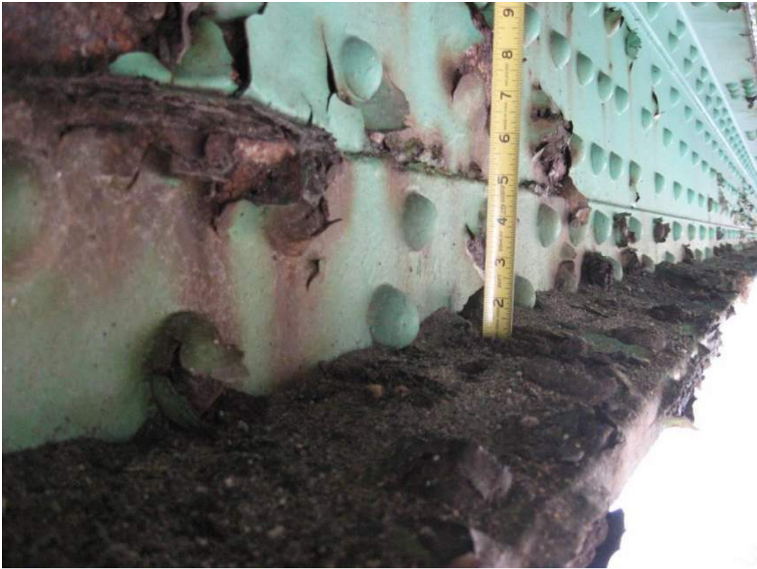
Photo 27 – Span 2 sidewalk truss lower chord east face has debris accumulations up to an inch deep over top of bottom flange of side channel for at least half of the span length.
