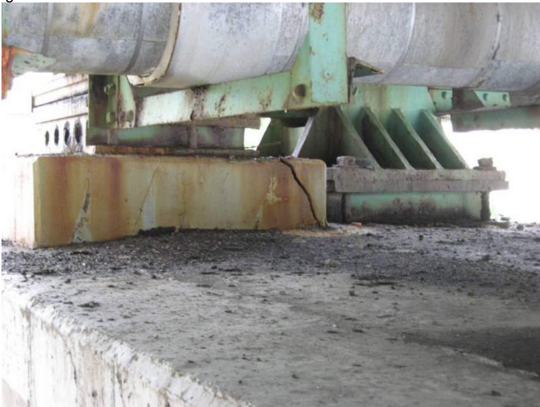
Photo 84 – Pier 2 has a wide diagonal crack in the southwest corner of the sidewalk truss bearing pedestal which extends for the full height of the concrete pedestal.
