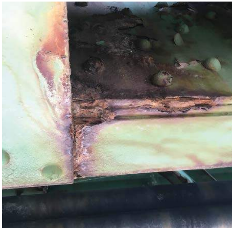
Photo #34: Pack rust between lattice plate and bottom angle on the the bottom chord of the sidewalk truss in span 3 (8//16)
