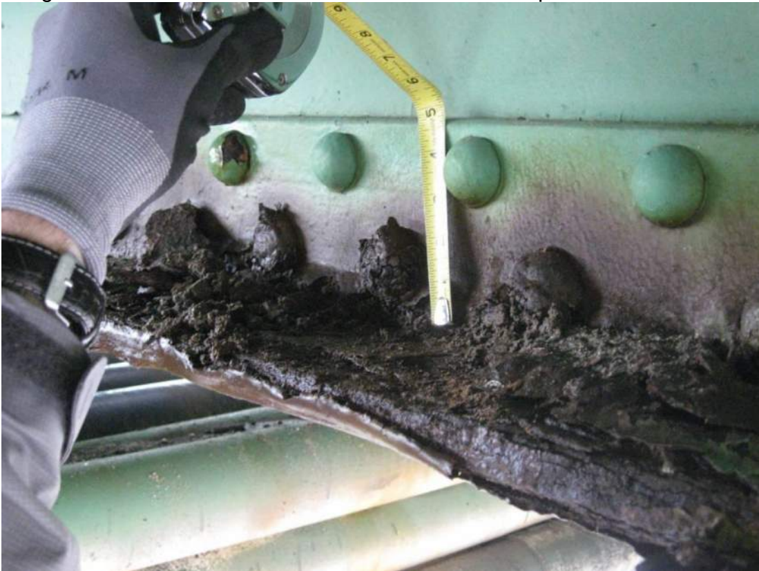
Photo 46 – Span 2 FB6 has a zone of significant active corrosion and 1/8 inch section loss to the top of the bottom flange on the south side of the web between S3 and S4.
