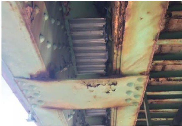
Figure 13: Bottom chord lattice plate bowing
