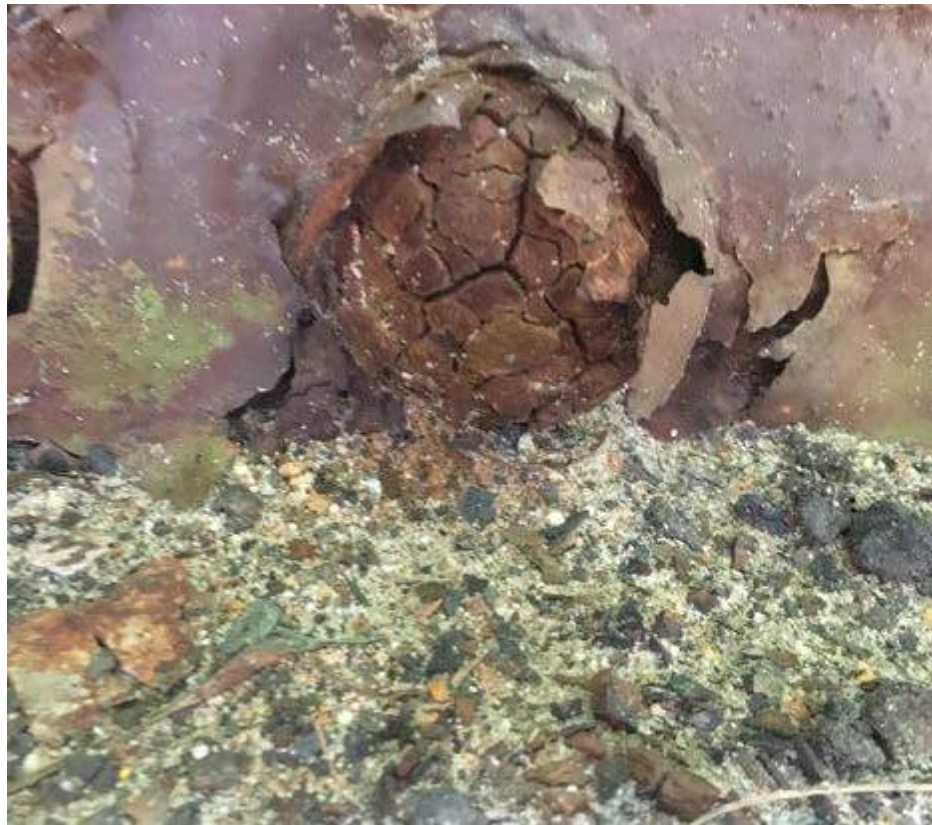
Photo #38: Severely deteriorated rivet heads on the bottom chord of the sidewalk side truss, span 3 (8/2/16)
