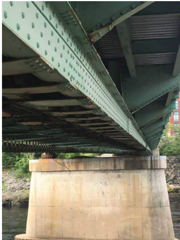
Photo #3: General view of the underside of the sidewalk side of the bridge (western side, Span 2 looking south) (8/1/16)
