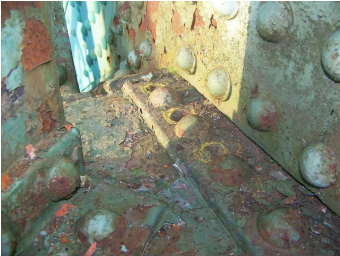
Photo 15 – Three additional mis-drilled rivet holes interspersed with the rivet holes were observed at the Span 2 roadway truss U9 west side channel lower angle. Looking north.
