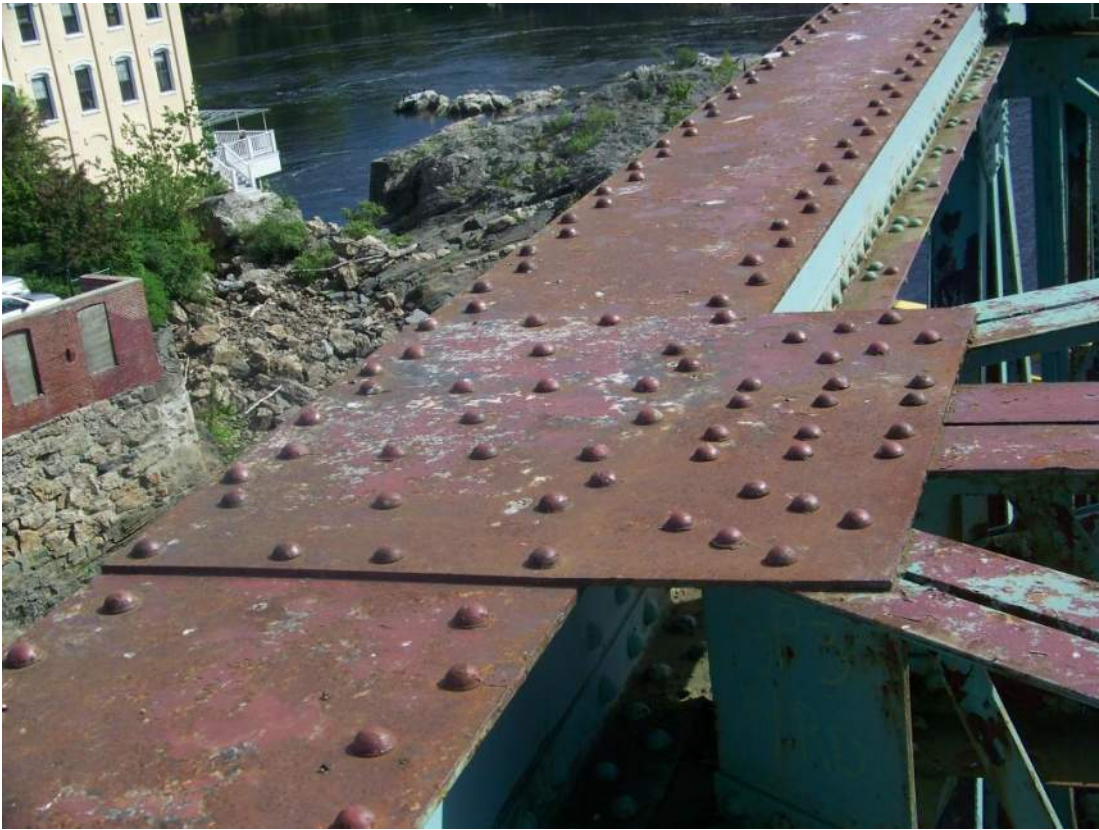
Photo 13 – Paint system is failed over more than 40% of exterior surfaces of upper chords with significant and widespread areas of missing paint and active corrosion.
