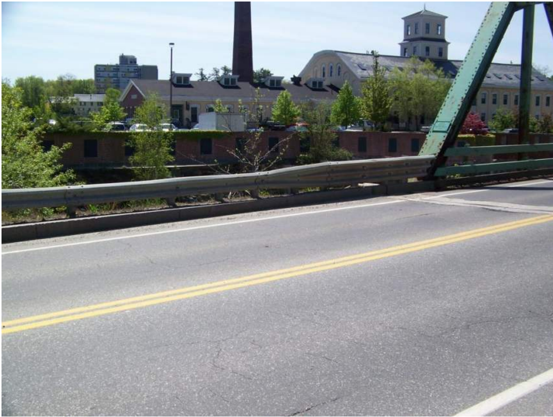
Photo 85 – Both approach pavements are in fair condition with several transverse and longitudinal cracks clustered in the wheel paths. Looking southeast at northeast corner.
