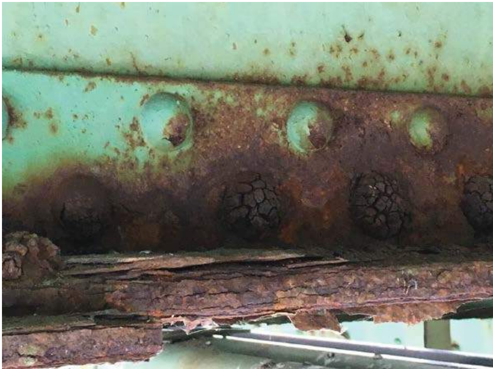
Photo # 19: Severe corrosion to the rivets as well as corrosion & pack rust between the bottom flange of the floor beam and the cover plate near midspan of FB5 in span 2 (span 2 FB4, FB6 & FB7 similar) (8/2/16)
