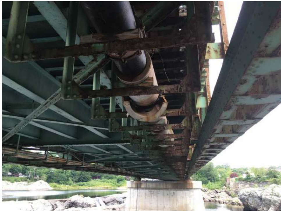
Photo #7: General view of utility pipe supported by a hanger system attached to the stringers (eastern side of structure looking north) (8/1/16)
