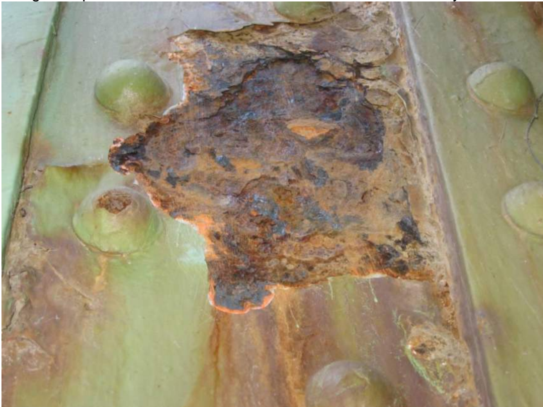
Photo 22 – In Span 1 roadway truss at L4 section loss of 1/16 inch depth was observed over a 4” long by 8 “ high area on east face of L3-L4 chord west side channel cover plate.
