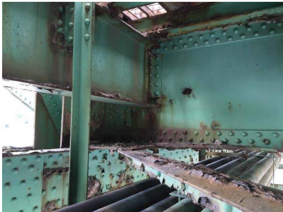
Photo #24: Typical exterior stringer (S3 & S8) to floor beam connection (Typ. all spans) (8/1/16)
