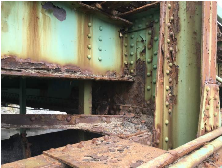
Photo #5: General view of the Floor Beam, Stringer & Vertical Truss member connection (8/1/16)
