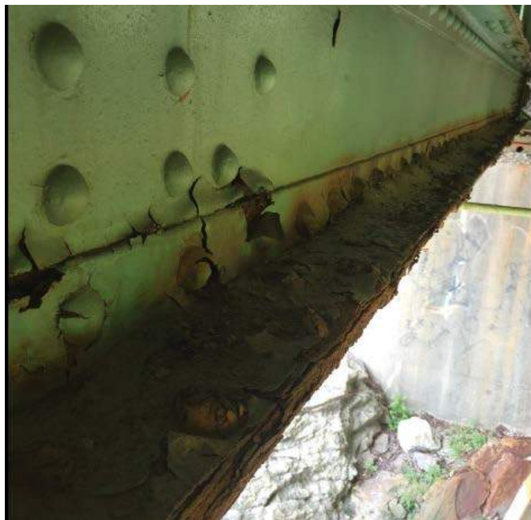
Photo #36: Corrosion to the bottom flange of the bottom chord of the sidewalk side truss in span 3 (western side of the bridge looking north) (8/2/16)
