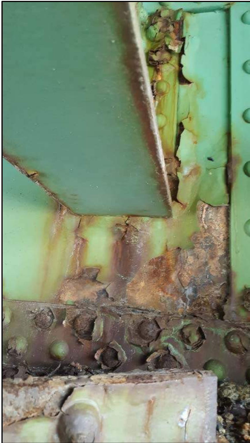
Photo A13 – Looking at the condition of north end of Stringer 8 attached to Floorbeam 3.
