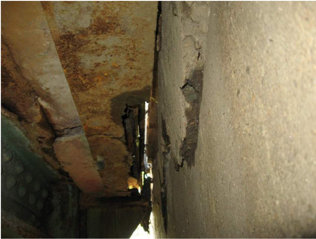
Photo 59 – A three inch width of the bottom flange south edge is missing from the south abutment transverse cross-beam over a 4 foot length between S7 and S8.
