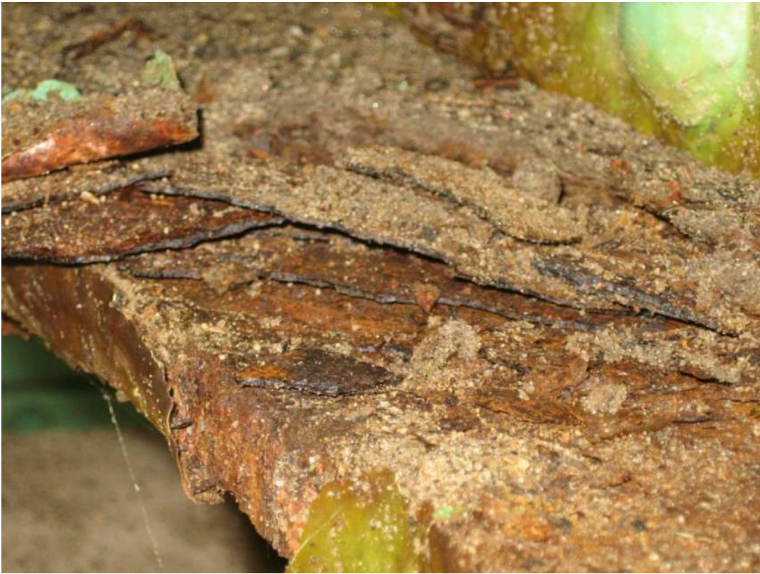
Photo 45 – Span 2 FB8 has significant active corrosion and delamination to top of bottom flange angle on north side of web between S6 and S8 with up to 1/8 inch section loss.
