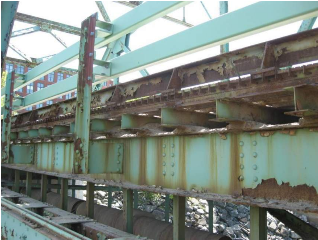
Photo 55 – Stringer S8 in Span 1 has heavy debris accumulations along the top flange at each of the grid deck cross beams between L2 and L3.
