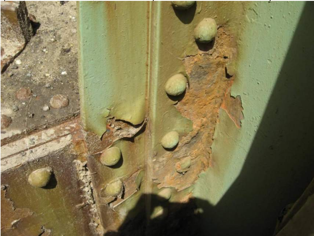
Photo 34 – Span 1 roadway truss U1-L1 has section loss of 1/16 inch to the east face of the vertical west flange over the half of the flange width south of the vertical web.
