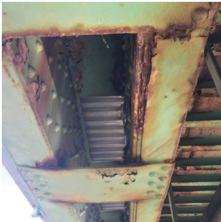
Photo #30: Typical corrosion of the bottom chord of the truss members, showing “bowing” of the Lattice plates due to pack rust (8/2/12)
