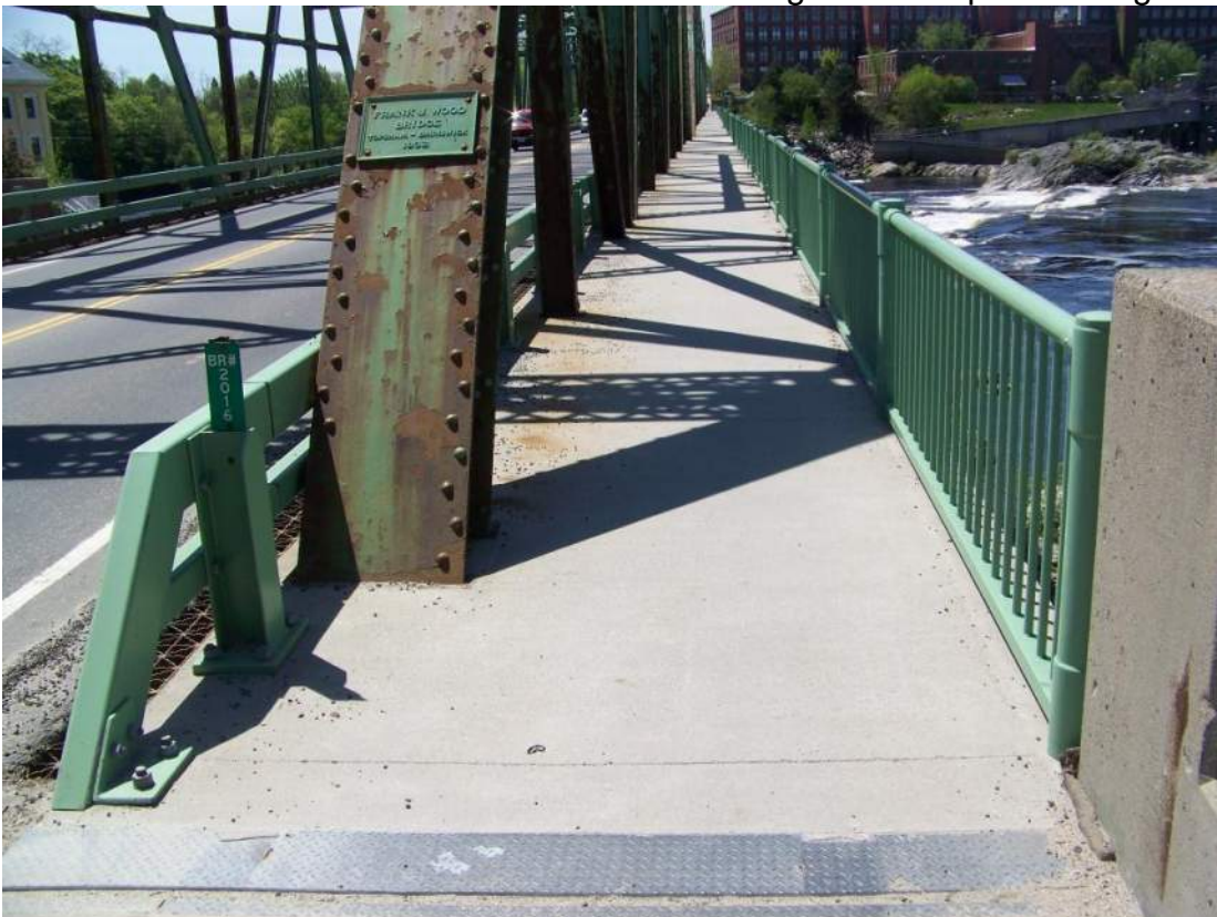
Photo 6 – The concrete curbs and sidewalk on the west side of the bridge are in good condition having been rehabbed relatively recently. Looking south from north abutment.
