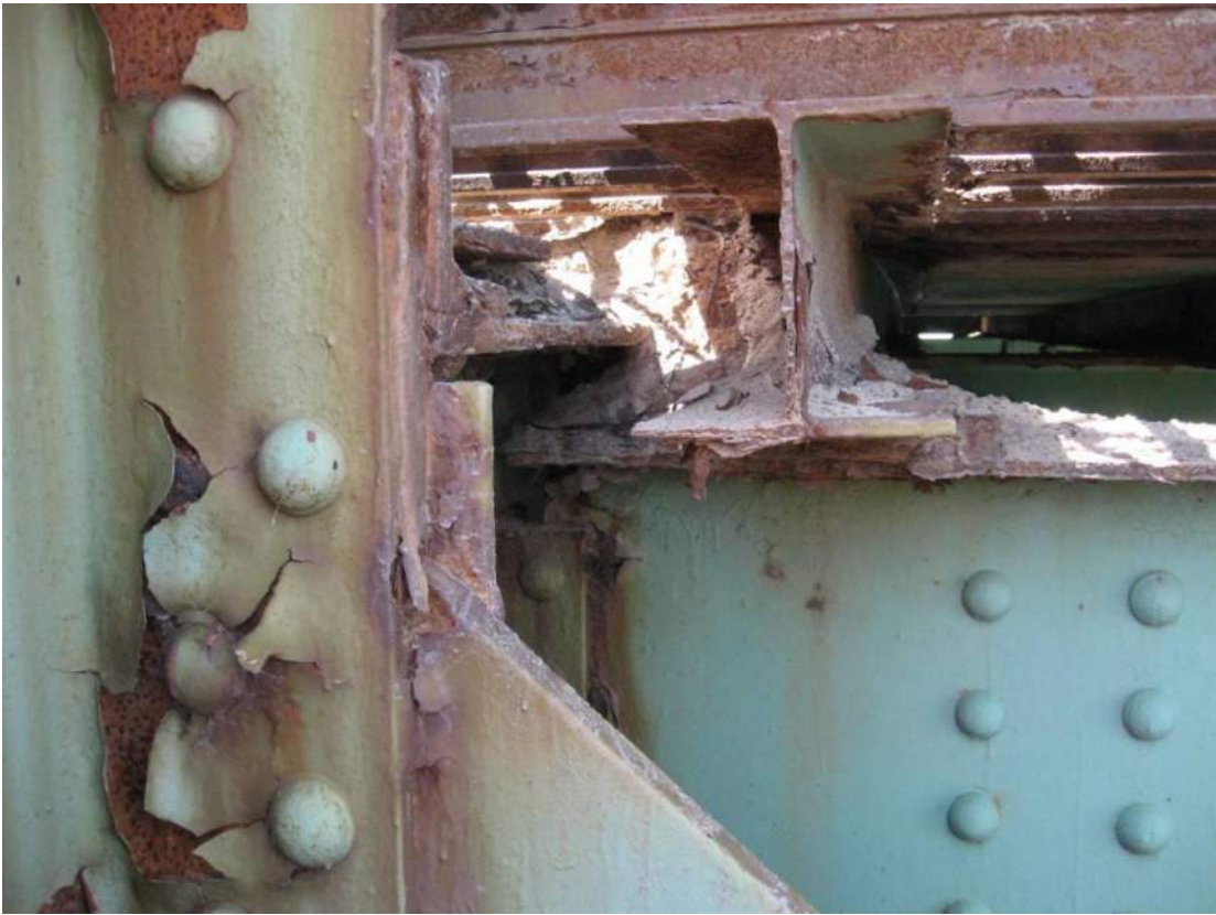
Photo 41 – Span 1 FB2 has heavy debris accumulation from 4 to 6 inches deep on the top of the floorbeam flange. View looking west at roadway truss.
