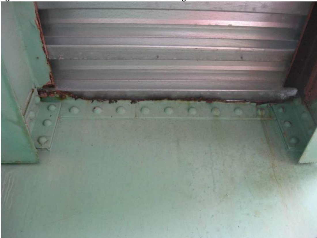
Photo 54 – Top flange angles of floorbeam cantilever brackets exhibit severe section loss, amounting to 100% of horizontal legs on both sides of the web between S1 and S2.
