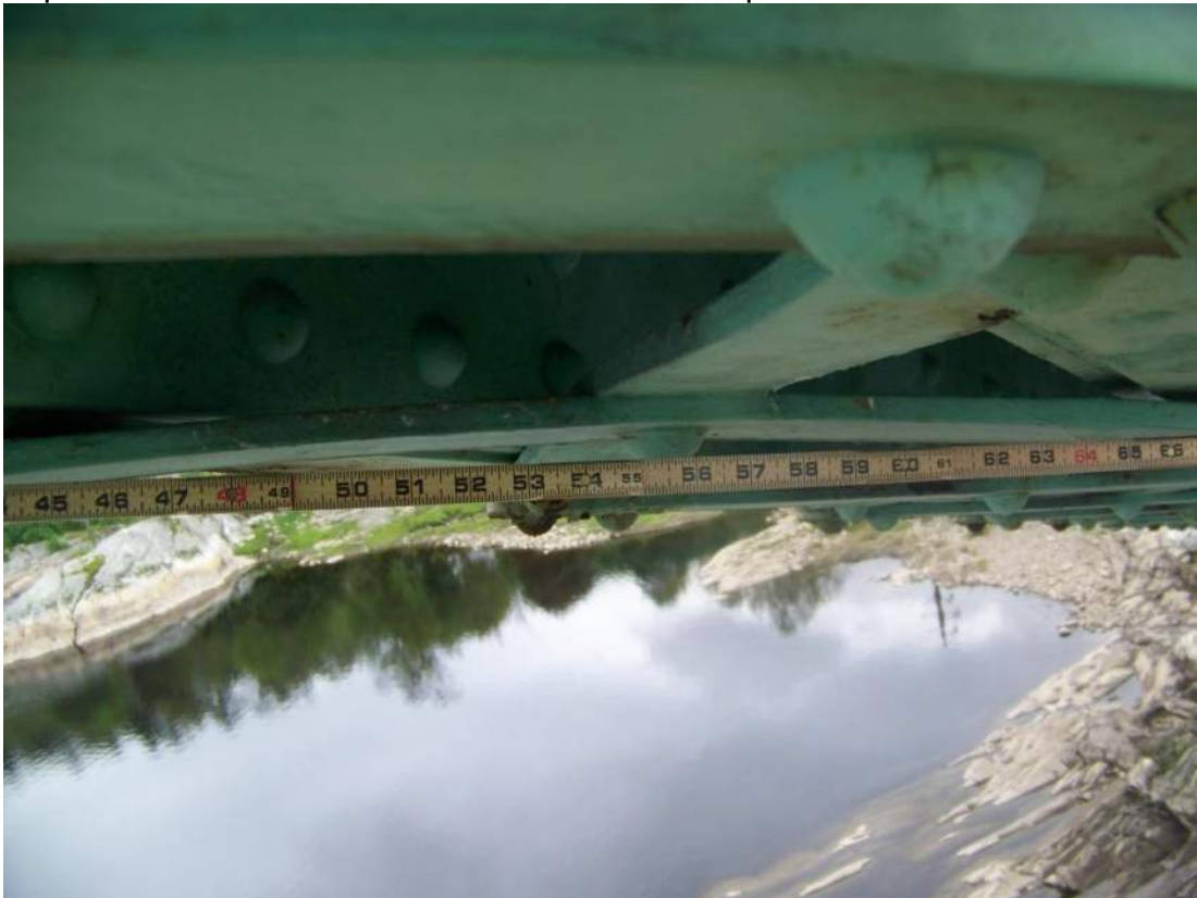
Photo 18 – The double lattice lacings bars in the Span 2 sidewalk truss U7-U8 upper chord have noticeable upward deflection. View is looking west.
