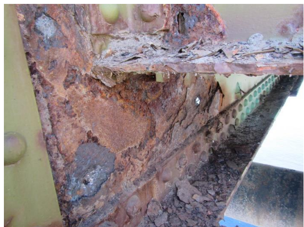
Figure 10: Deteriorated floor beam
