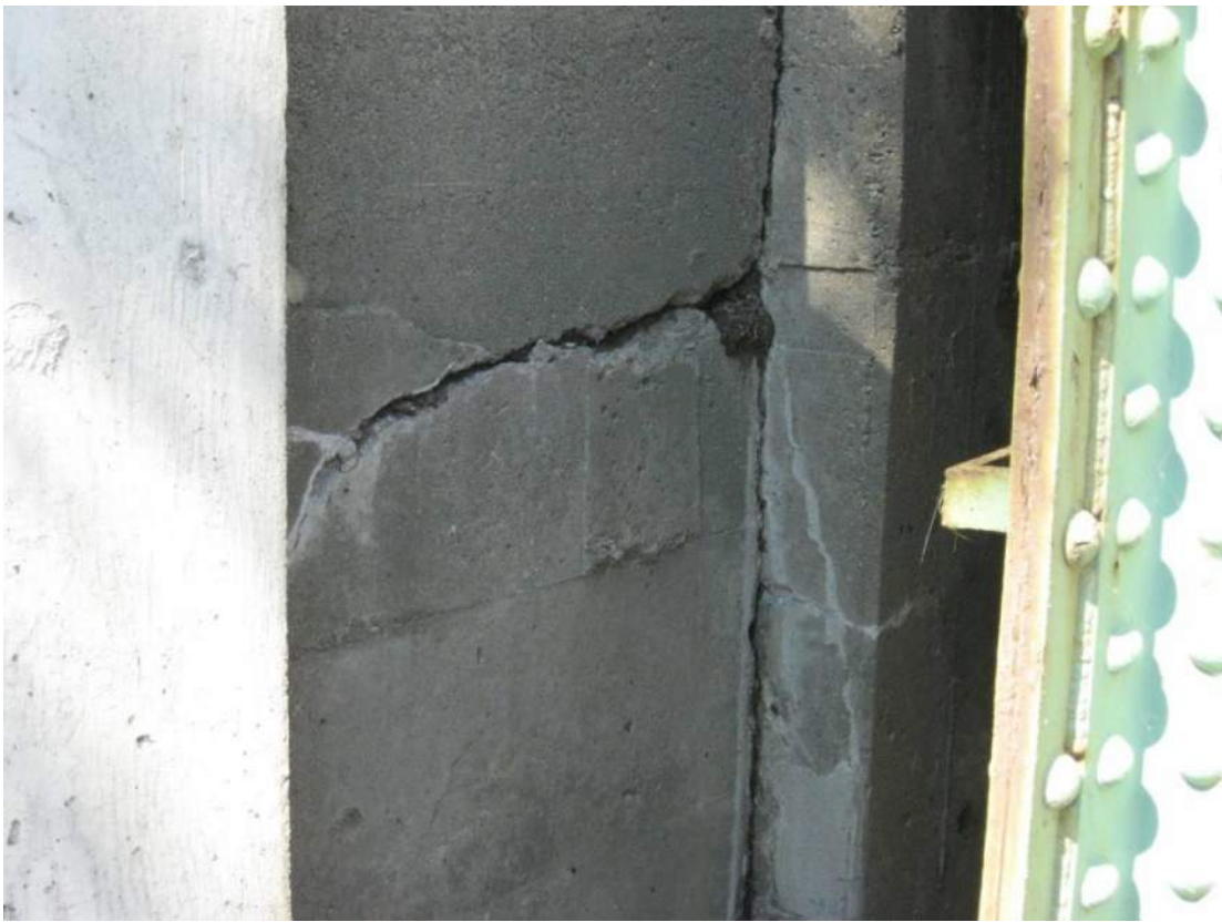
Photo 77 – The south abutment backwall has a wide 2 foot long horizontal crack near the wingwall corner at approximately 4 feet above the bridge seat.
