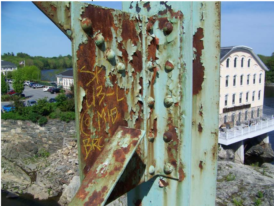
Photo 68 – The mid-lateral sway frame bracing connection plates at U3 to U7 typically have peeling or failed paint. View at Span 2 roadway truss U3-L3 mid-lateral.
