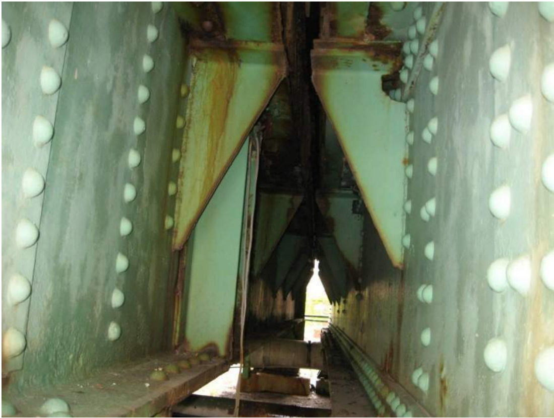
Photo 49 – Partial height welded stiffeners on face of web below deck joint also observed at Pier 2 for the Span 2 and 3 end floorbeams (fatigue-sensitive details in FCM's).
