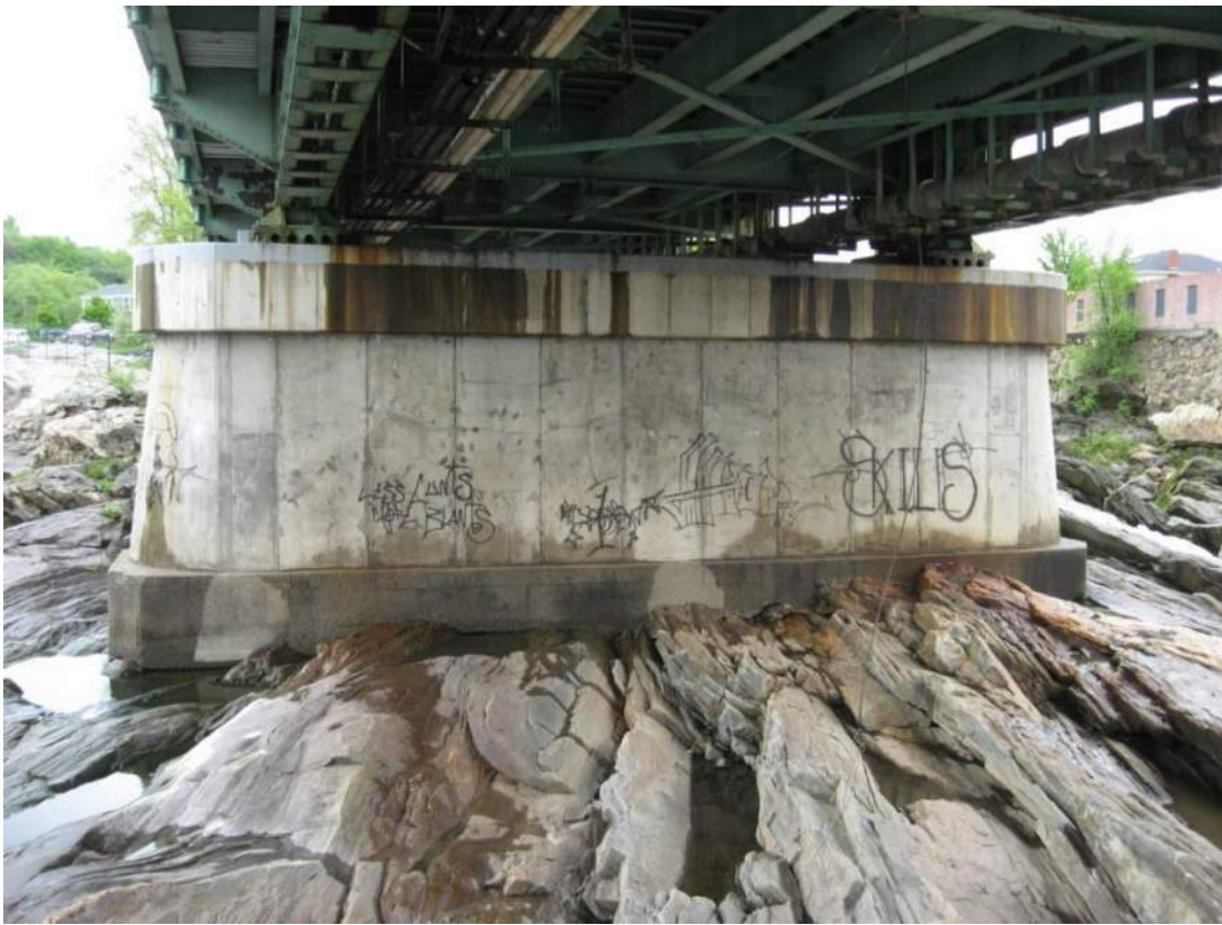
Photo 83 – Piers are in satisfactory condition with no significant visible defects. View looking north at south face of Pier 2.
