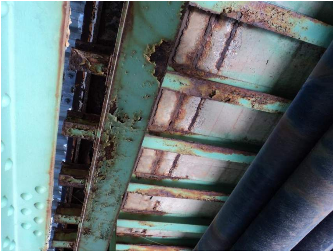
Photo 5 –Along outer edges of deck at S3 and S8 exposed main longitudinal grid deck bars were visible and exhibited active corrosion. Looking north in Span 1 along S3.
