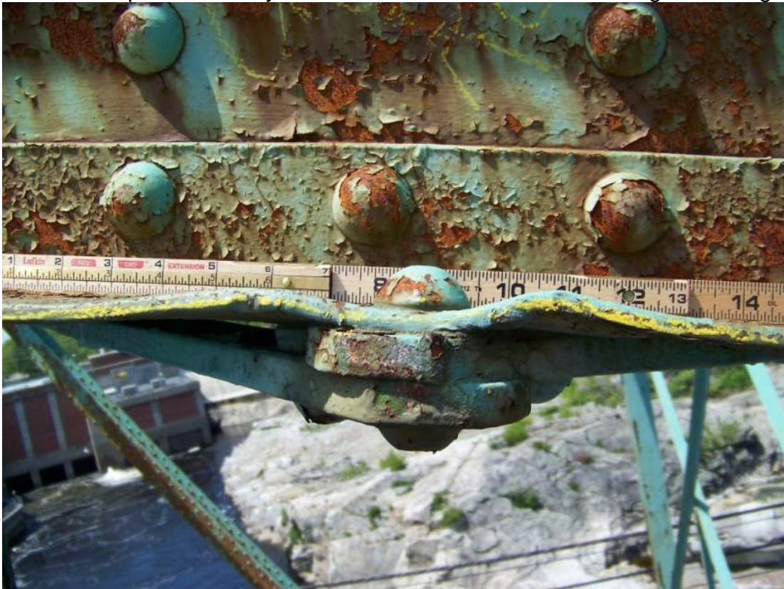
Photo 16 – Slight vertical distortion was noted in the bottom flange angles at and/or between the lacing bars at various locations. View at Span 1 U7-U8 sidewalk truss.
