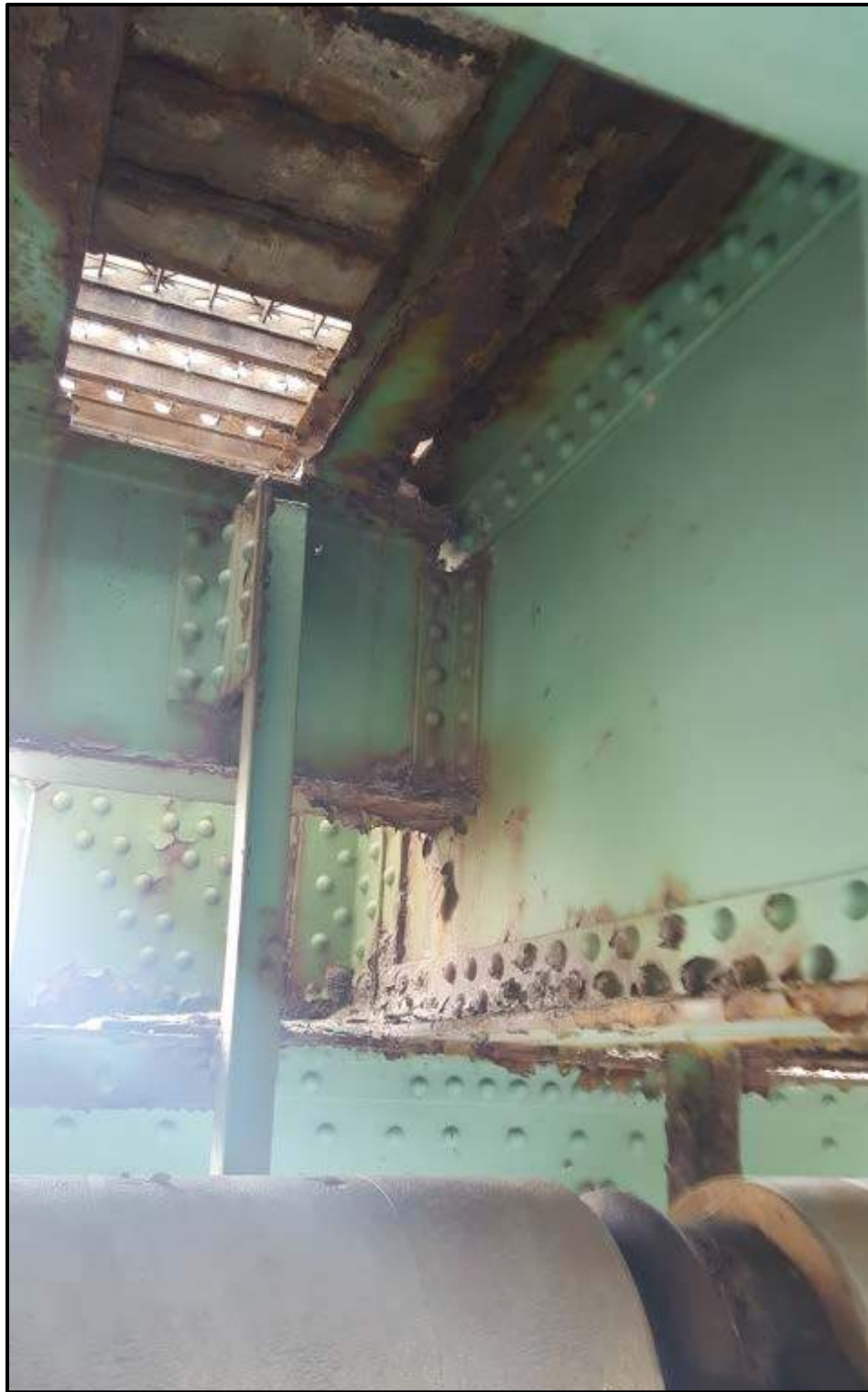
Photo A14 – Stringer 8 connection to Floorbeam 6, Roadside Truss, may warrant a reattachment repair within 5 years. Similar connection conditions @ Stringer 3 to Floorbeams 6 and 7.
