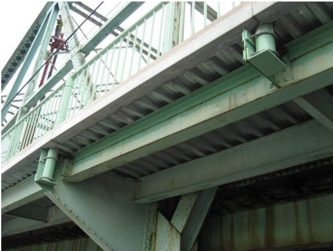
Photo 57 – Sidewalk stringer S1 has been previously repaired at numerous panels by stitch welding a pair of angles to top of web, to restore section loss to original top flange.
