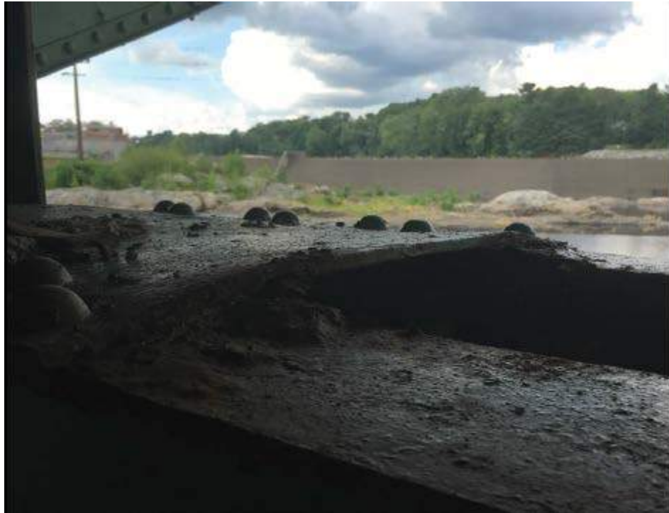
Photo #33: "Bowing" of lattice plates on the top of the bottom chords of the sidewalk truss in span 3 (8//16)
