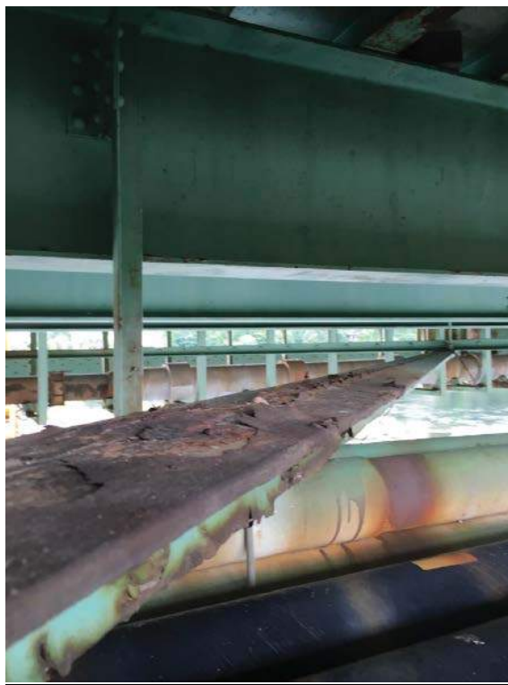
Photo #52: General top view of lateral bracing span (inverted) from non-sidewalk truss to sidewalk truss in spans 1 & 2 (8/2/16)
