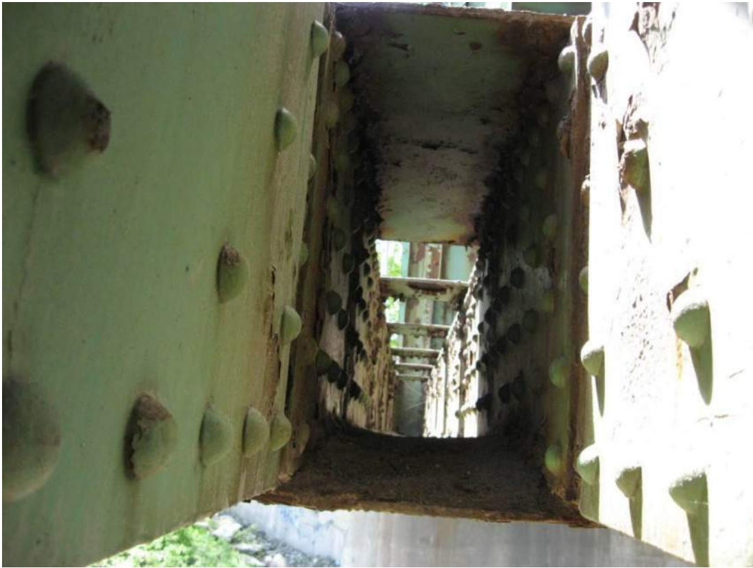
Photo 19 – Heavy debris accumulations up to four inches deep were observed on the top of the lower chord bottom plate near the Span 1 roadway truss L2 splice region.
