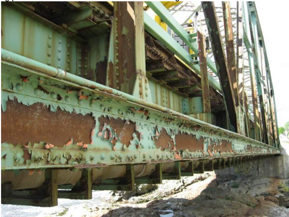
Photo 26 – In Span 3 the entire length of the east face of the roadway truss has severe paint failure with active corrosion. Looking north toward north abutment.
