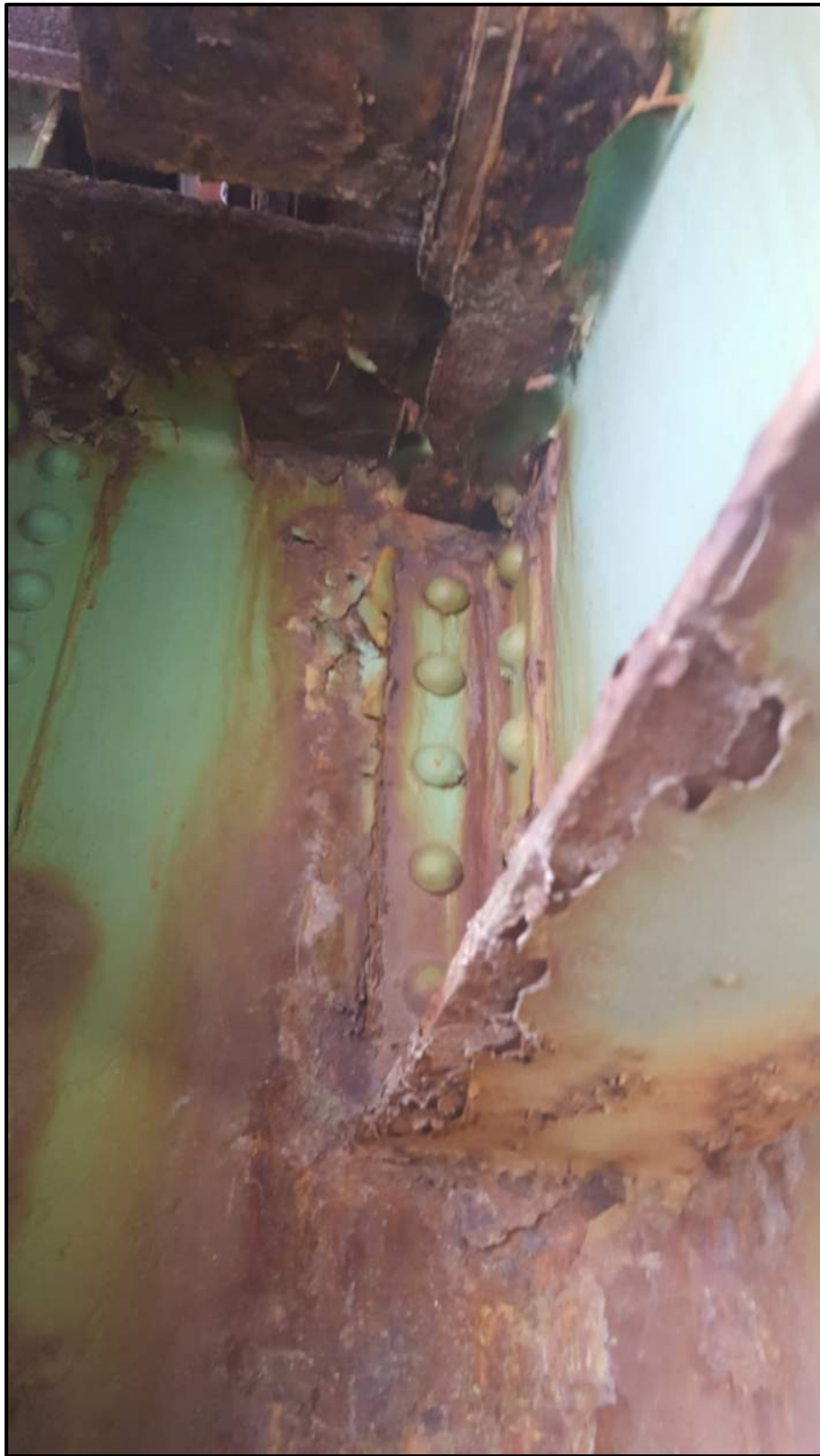
Photo A19 – Stringer 8 connection to Floorbeam 6 will likely require repairs within 5 years.
