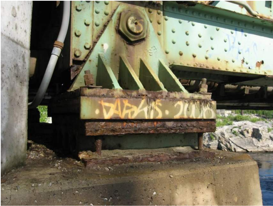
Photo 75 – The two anchor bolts on the east side of the south abutment roadway truss bearing were noted to be bent off plumb in opposite directions.
