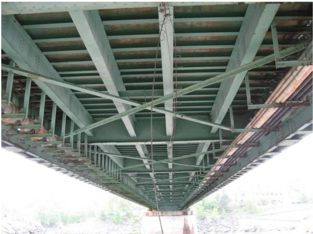
Photo 91 – Remnants of an abandoned wire cable attached to the floorbeams were observed dangling at several locations. View looking south in Span
