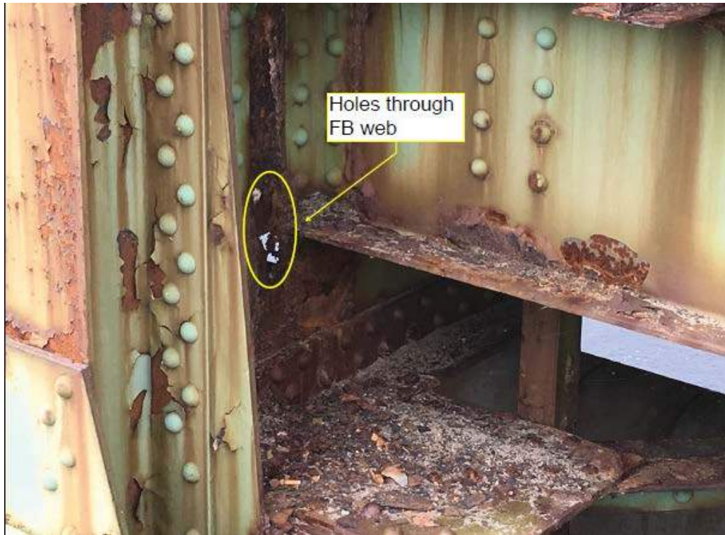
Photo # 15: General view of corrosion and holes through the web of non-sidewalk (eastern) end of FB7 in span 1 (8/1/16)
