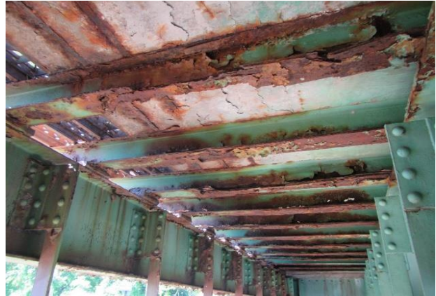
Figure 8: Deteriorated crossbeams & deck
