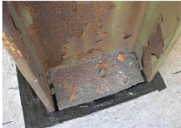
Figure 13: Plate welded to truss vertical
