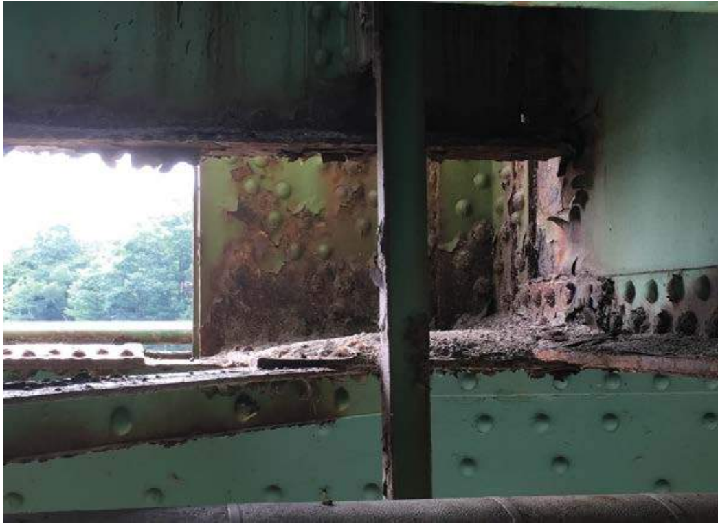
Photo # 11: General view of typical paint loss & debris collection at floor beam ends (8/1/16)
