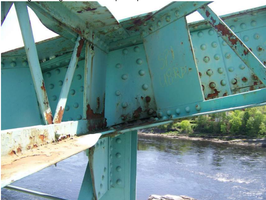
Photo 66 – The ends of the top laterals at numerous locations have intentional crimping-related distortion to accommodate the member slopes at the upper panel points.
