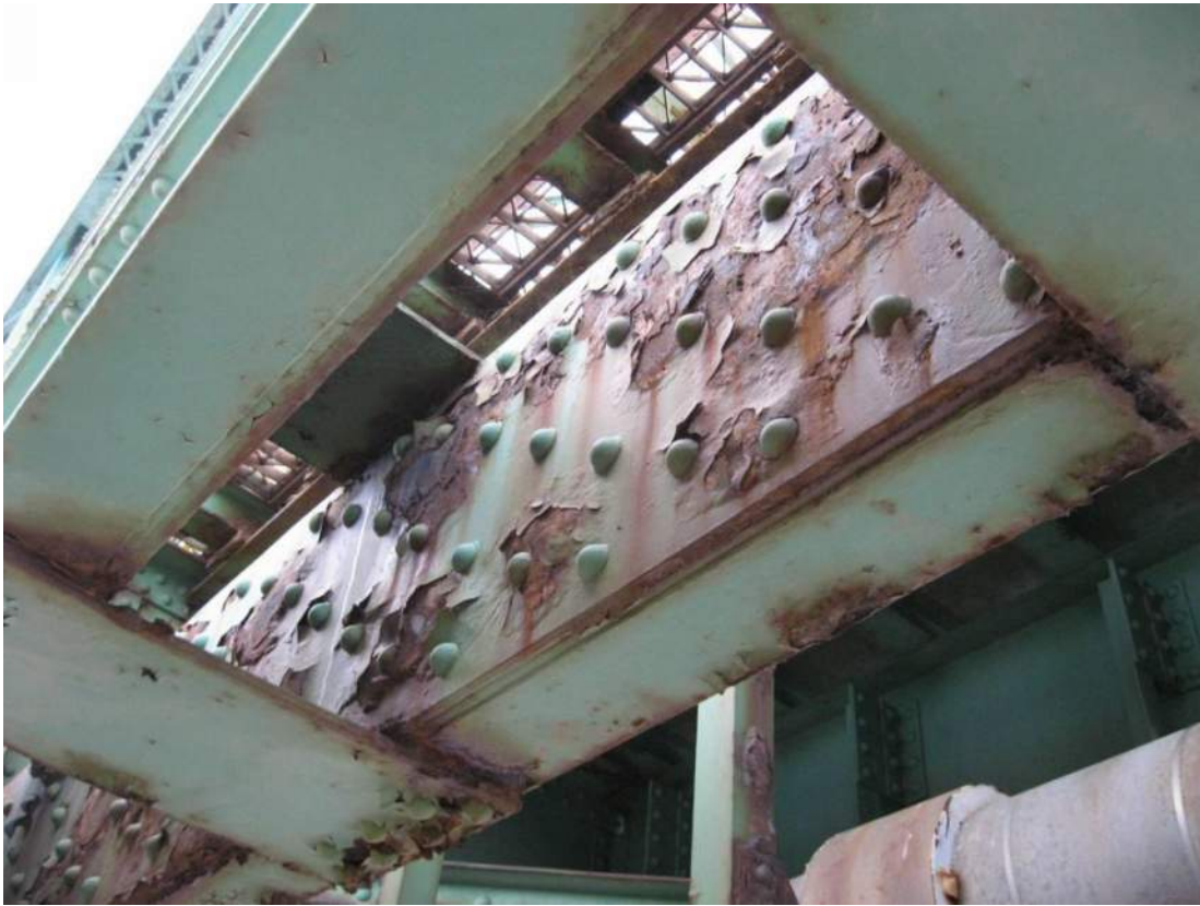
Photo 33 – Interior vertical side channels of Span 3 roadway truss L3-L4 exhibit areas of failed paint, active corrosion, and raised expansive exfoliation similar to pack rust.
