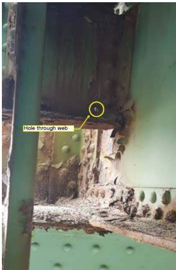
Photo #26: Hole through the web of S8 at FB2 in span 1 (8/1/16)
