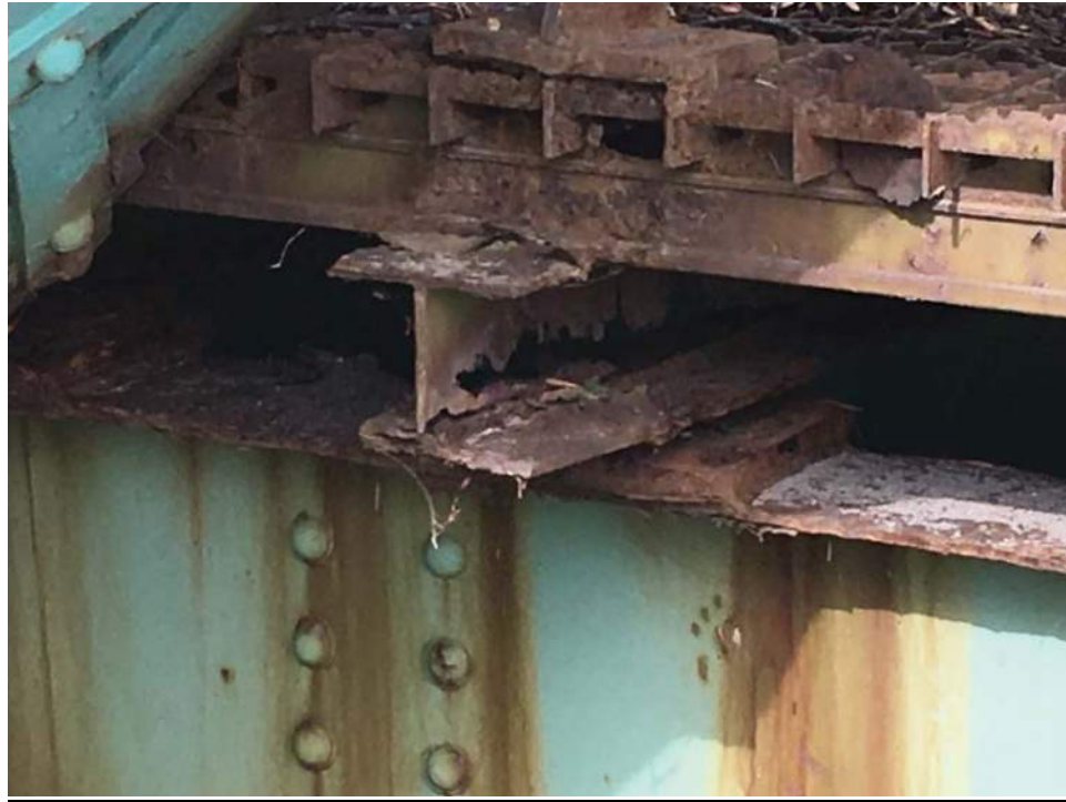
Photo #45: Severe corrosion to a cross beam (needle beam) near FB 1 in span 1 of non-sidewalk (eastern) truss (8/1/16)
