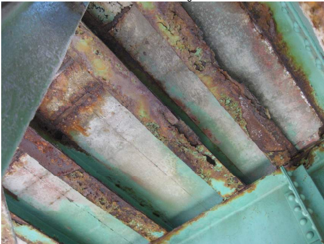
Photo 60 – Section loss and perforation to two cross-beams in Span 1 near FB2 between S7 and S8 where bottom flange has up to 3/16" section loss over 2 inches along edge.
