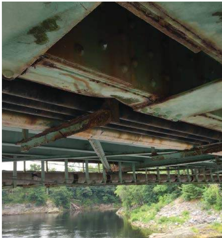
Photo #40: "Dent" to the interior member making up the bottom chord on the sidewalk (western) truss, located near midspan of span 1, likely due to impact of debris during extreme high flood waters (8/1/16)
