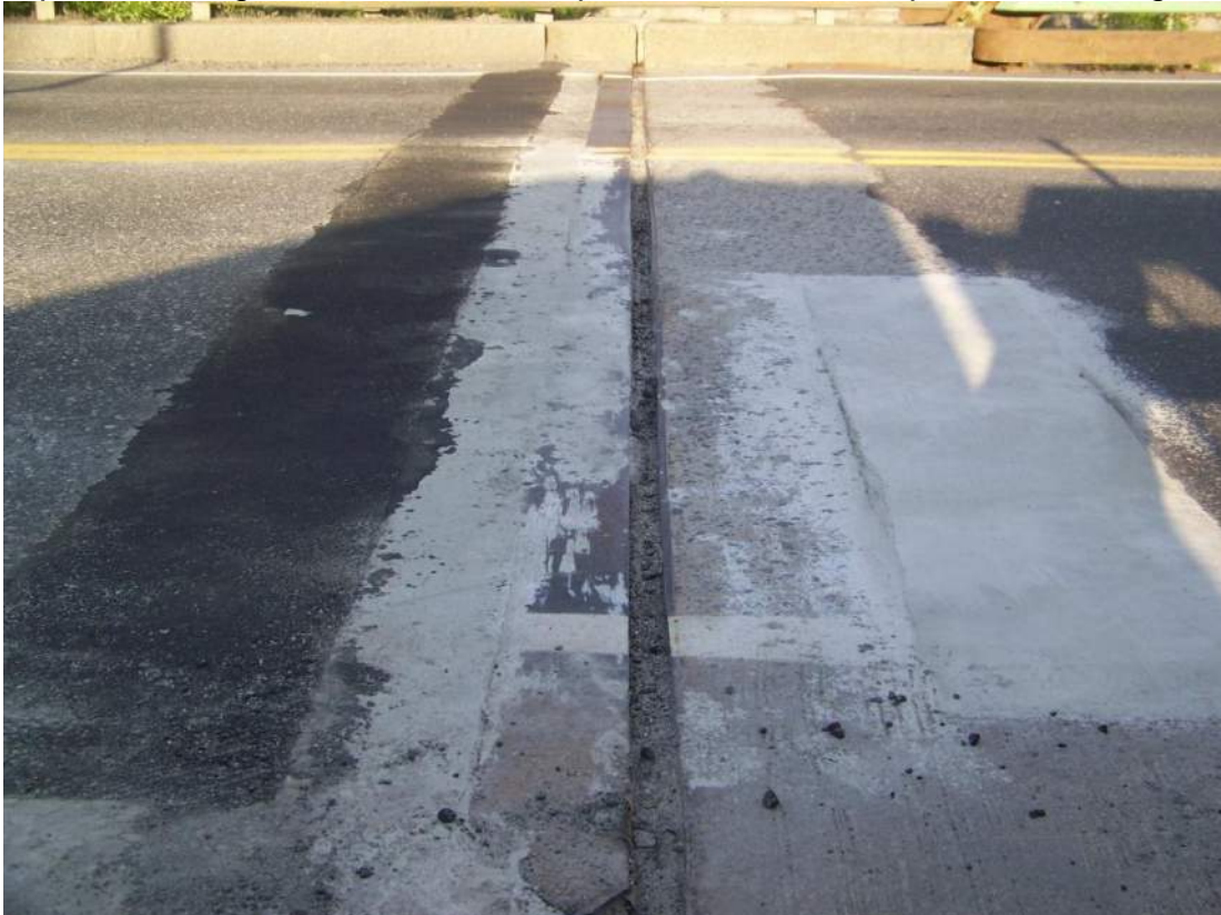
Photo 10 – The north abutment compression seal type deck joint is filled with debris and the concrete headers were patched with quick-setting concrete during the inspection.
