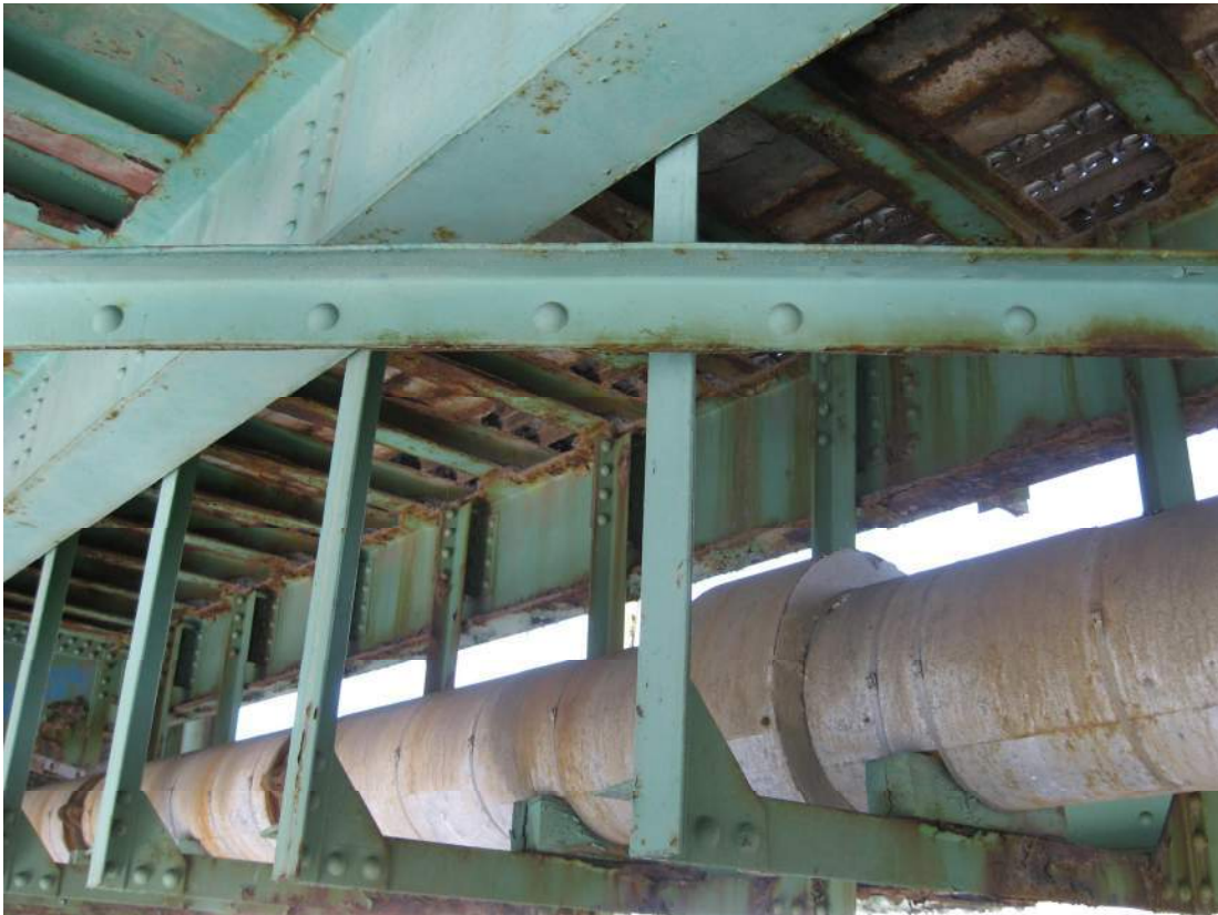
Photo 61 – The typical paint condition on grid deck cross-beams between S7 and S8 is poor throughout the bridge length with active corrosion on most cross-beams this bay.
