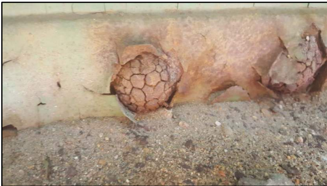
Photo A9 - Typical rivet head condition along Sidewalk Truss Lower Chord of Span 3 for at least 100 ' length of angle to plate connection.
