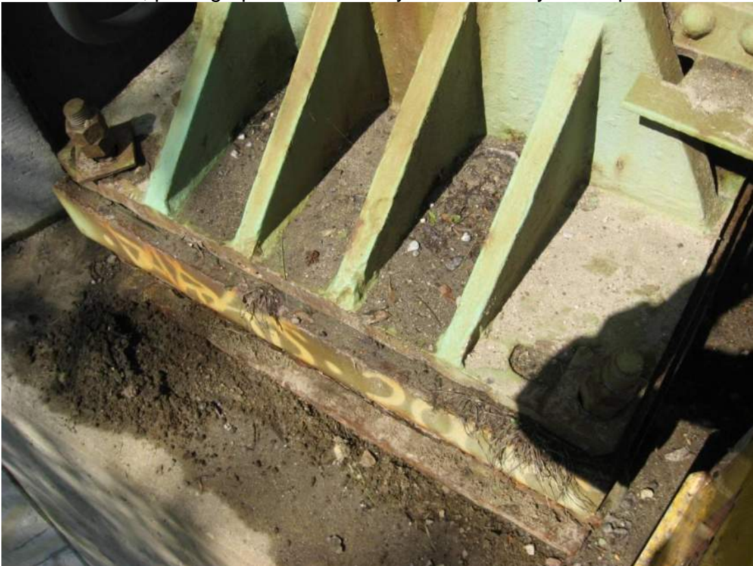
Photo 74 – Expansion slots in the south abutment roadway truss bearing upper shoe are completely filled with debris accumulations which preclude normal thermal movement.
