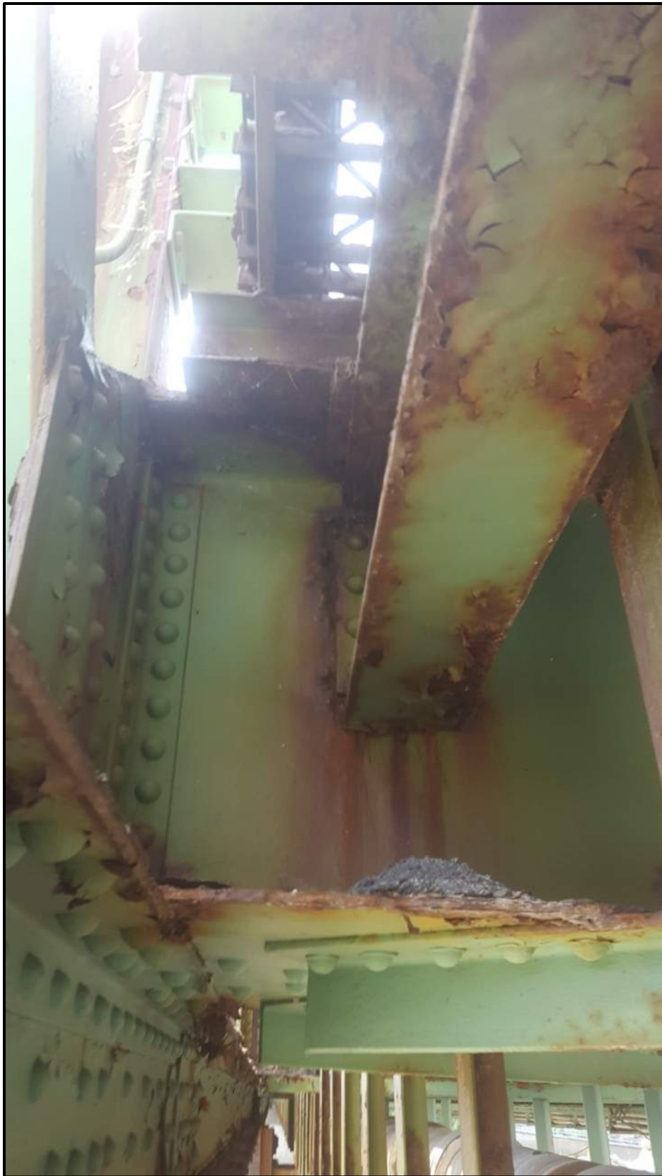
Photo A16 – Stringer 8 connection to Floorbeam 2 will likely need repair within 5 years.
