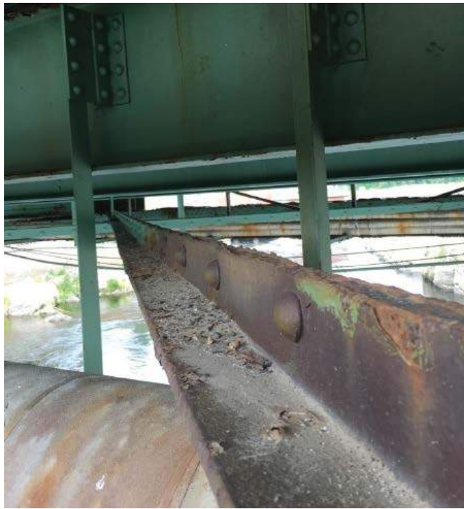
Photo #53: General top view of lateral bracing span from sidewalk truss to non-sidewalk truss in spans 1 & 2 (8/2/16)
