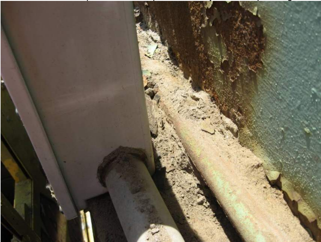
Photo 20 – Packed debris up to two inches deep on top of Span 1 roadway truss L2 lower chord outboard channel where electrical conduits and junction box trap and collect dirt.
