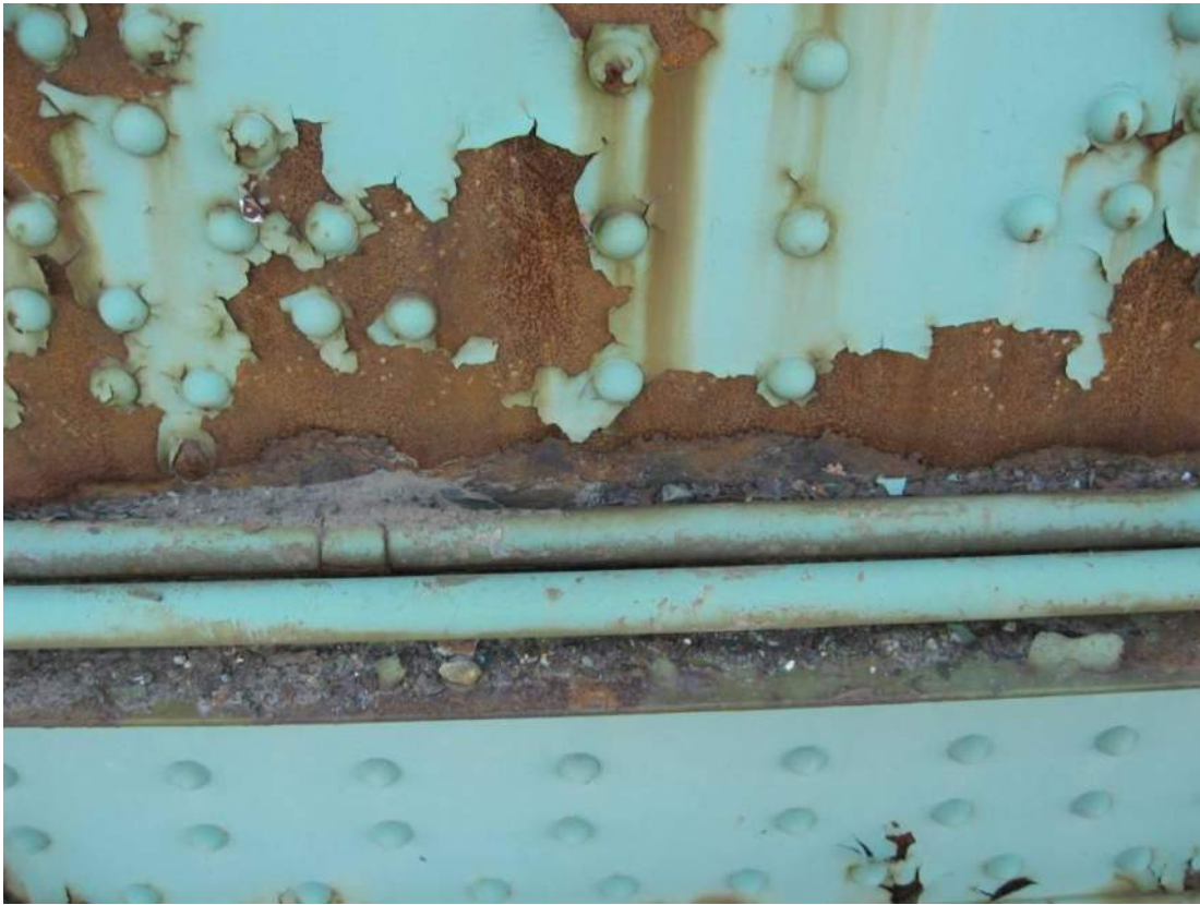
Photo 21 –In Span 1 roadway truss L4 joint minor exfoliated rusting was noted over 3” of outboard gusset plate due to moisture and dirt accumulation caused by the conduits.
