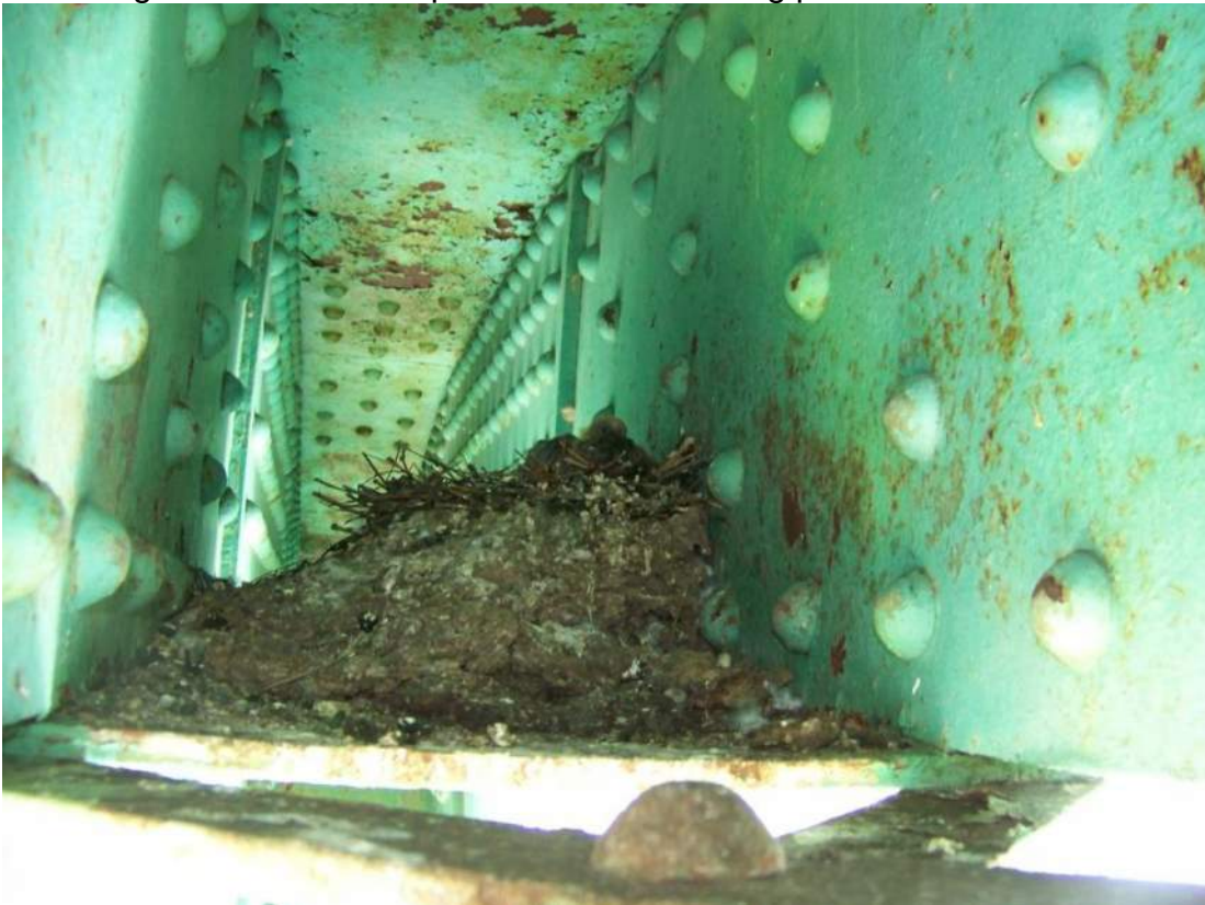
Photo 14 – The interior surfaces of upper chords exhibit paint failure rates averaging 10% and there are bird nests present on top of nearly all of bottom face batten plates.
