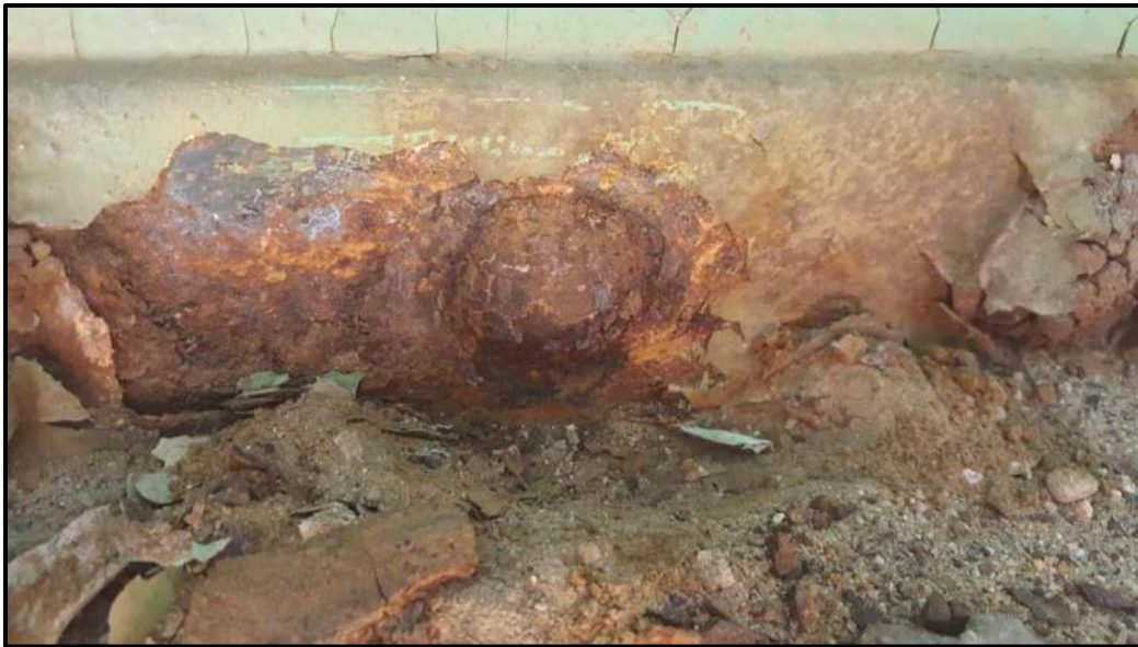
Photo A10 – This is the same rivet as above after briefly pounding loose corrosion away. The rivet head size is significantly smaller than the diameter and height of a new rivet head.
