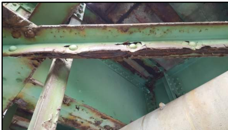
Photo A26 – In general, a good amount of deterioration exists in the lateral bracing system.
