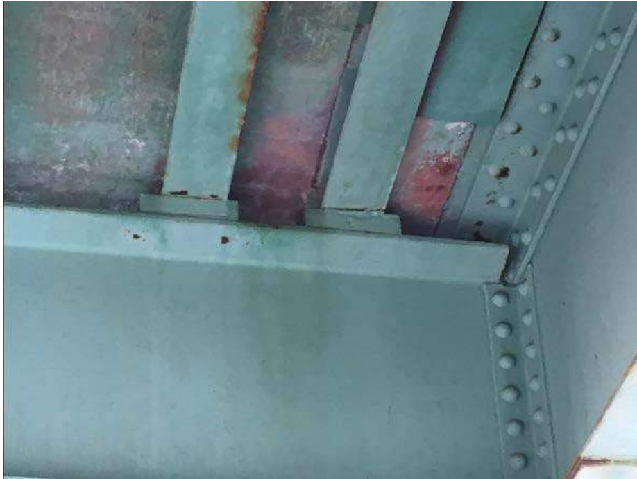
Photo #47: Failed weld between needle beam and an interior stringer in span 1 (8/1/16)
