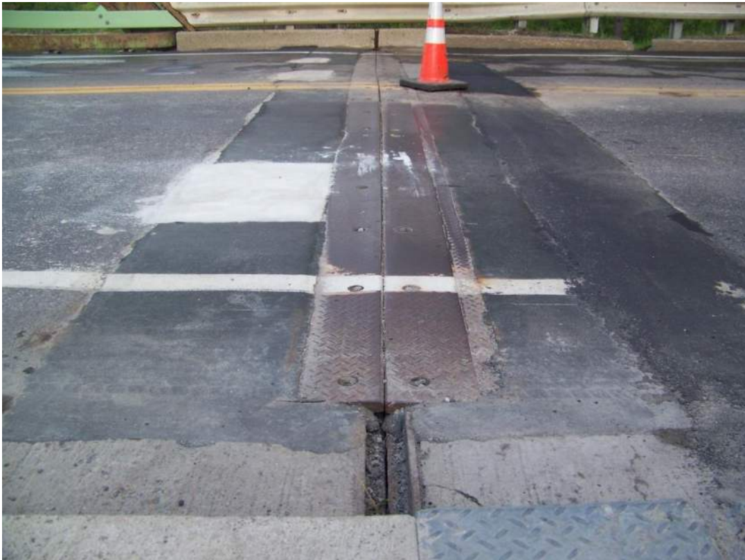
Photo 7 – South abutment open plate deck joint was previously patched with bituminous material; additional bituminous and concrete patching and other repairs were being performed during the inspection.
