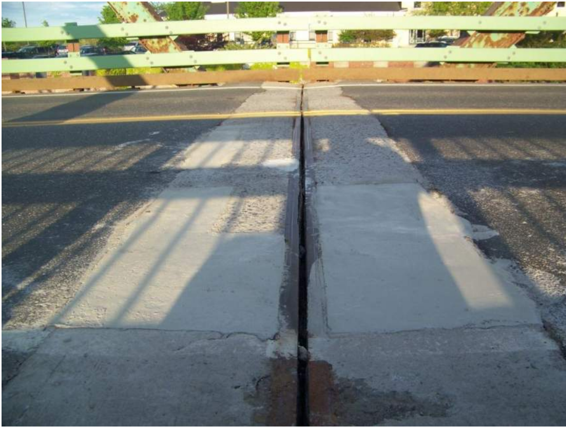
Photo 9 – The north pier strip seal type deck joint has three quick-setting concrete patch repairs placed during the lane closures implemented for the inspection. Looking east.
