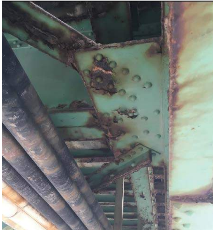
Photo #49: Typical view of lateral bracing connection to bottom horizontal gusset plate in spans 1 & 2 (8/1/16)
