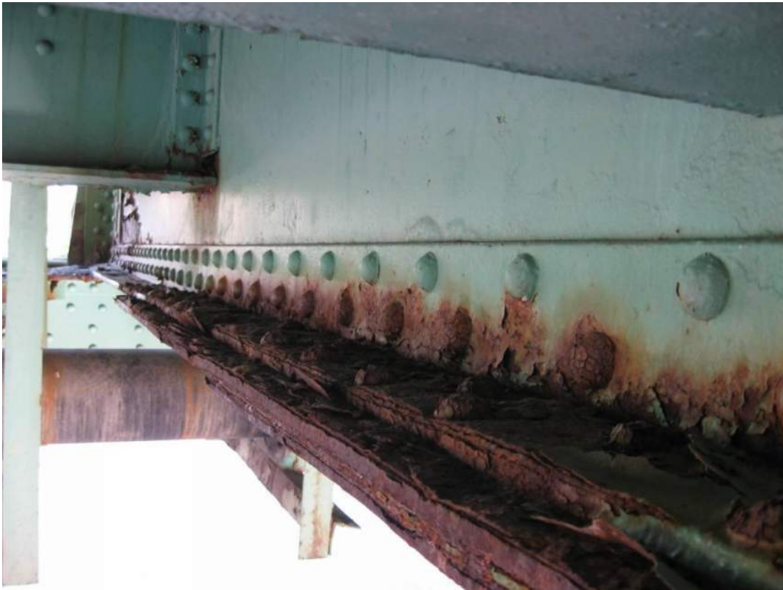
Photo 43 – Span 1 FB5 has a zone of significant active corrosion to top of bottom flange on north side of web between S6 and S7 with up to 1/8 inch section loss to rivet heads.
