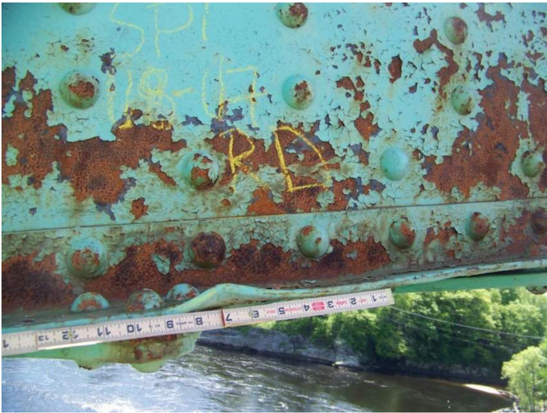
Photo 17 – Minor localized bends in flange angles with up to 5/8 inch vertical deflection of flange tip were observed at a few locations. View at Span 1 U7-U8 sidewalk truss.
