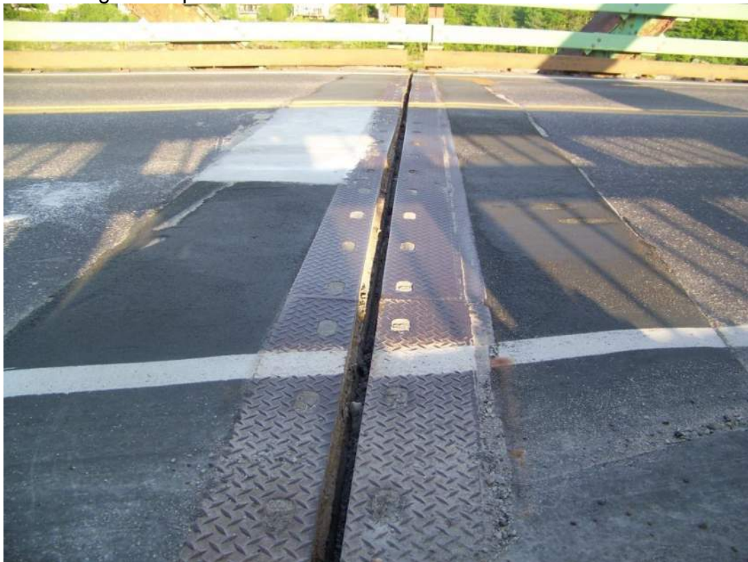
Photo 8 – The south pier strip seal type deck joint was previously patched with bituminous material and a concrete patch was placed during the inspection.
