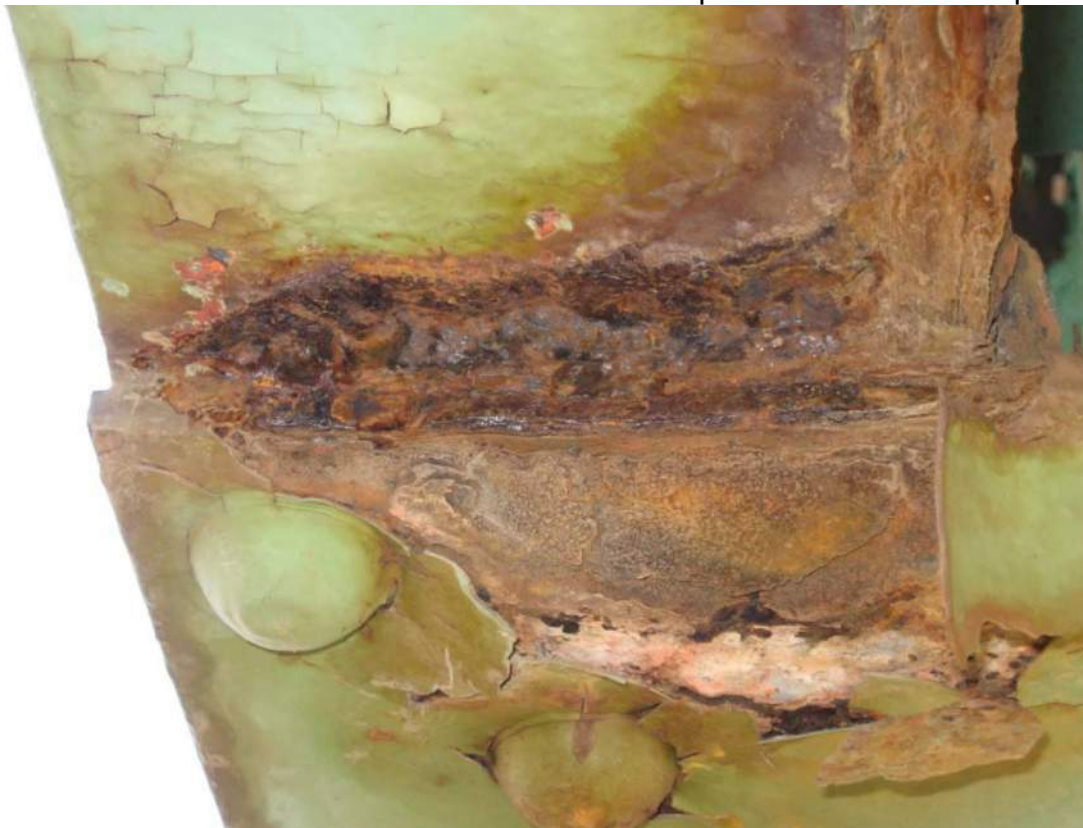
Photo 32 – Span 3 roadway truss L6-L7 has 1/4 inch of section loss over 4 inch width on east side channel and 1/8 inch section loss over a 4 inch width to west side channel.
