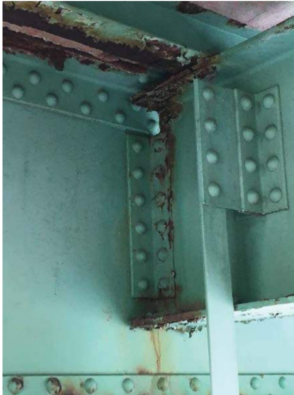
Photo #29: Typical interior stringer (S4 through S7) to floor beam connection (Typ. all spans) (8/1/16)
