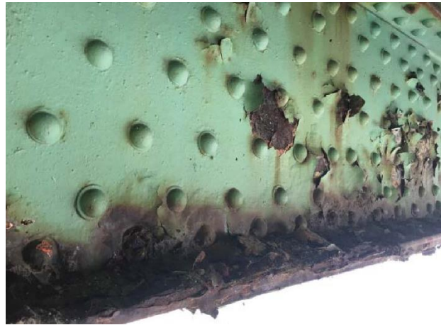
Figure 11: Bottom chord bottom flange corrosion
