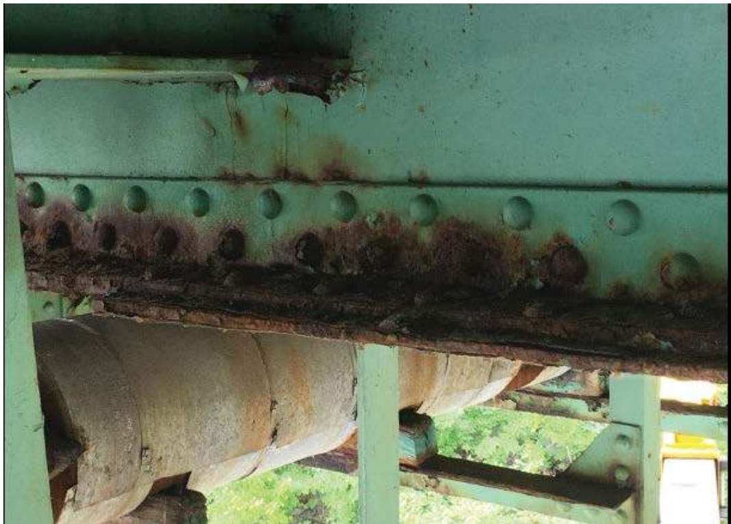
Photo # 18: Severe corrosion & pack rust between the bottom flange of the floor beam and the cover plate near midspan of FB5 in span 2, (span 2 FB4, FB6 & FB7 similar) (8/2/16)
