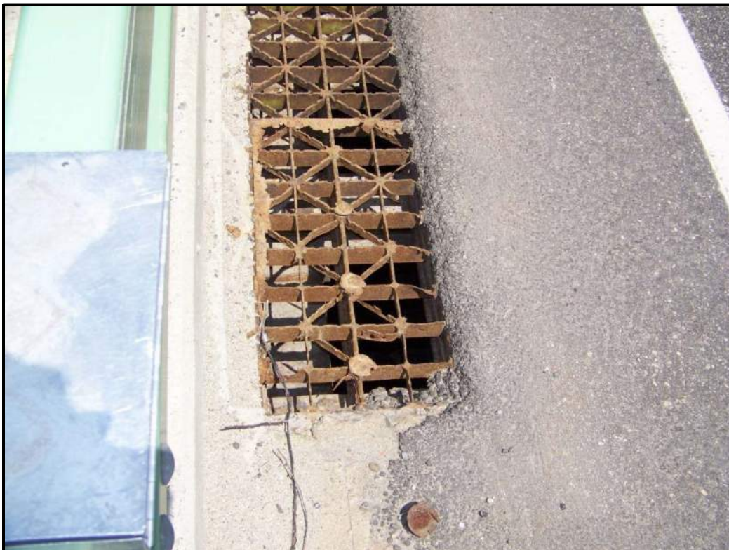
Photo A22 – An open grid approximately 1 foot wide runs parallel to Stringers.
