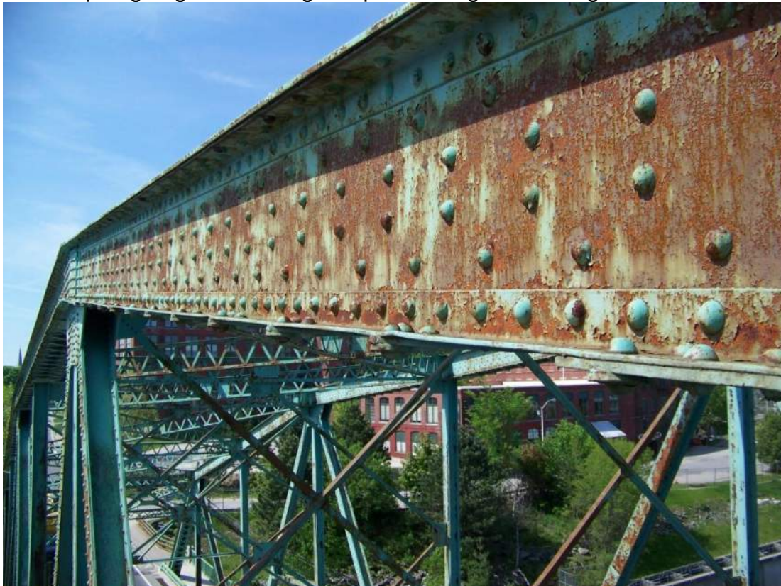
Photo 12 – Paint system is failed over more than 40% of exterior surfaces of upper chords with significant and widespread areas of missing paint and active corrosion.
