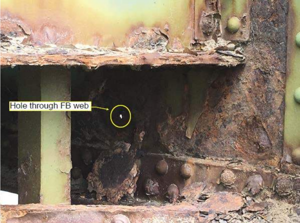
Photo # 12: General view of corrosion & hole through the web on the non-sidewalk (eastern) end of FB2 in span 1 (8/1/16)
