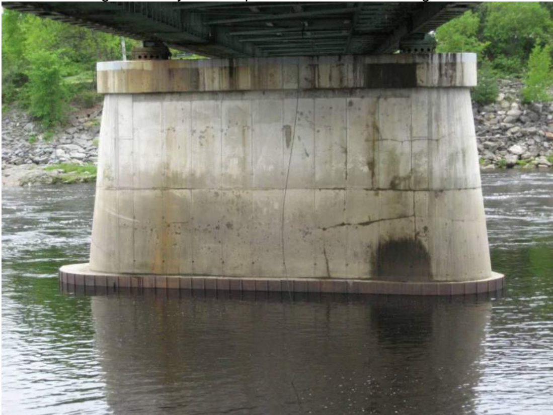
Photo 82 – Piers are in satisfactory condition with no significant visible defects. View looking south at north face of Pier 1.
