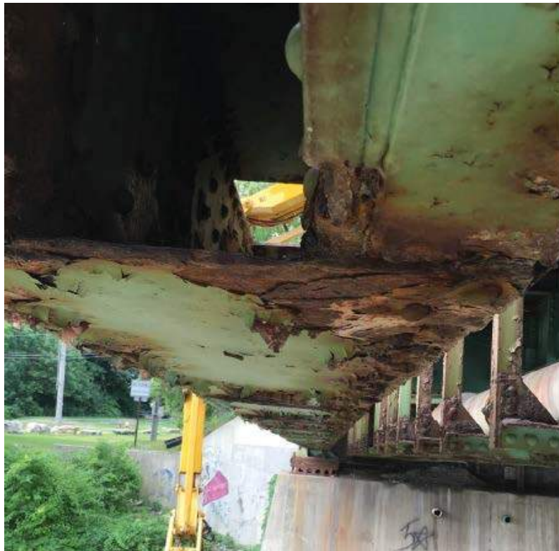
Photo #31: Corrosion of lattice plate on bottom chord of non-sidewalk truss in span 1 (8/1/16)
