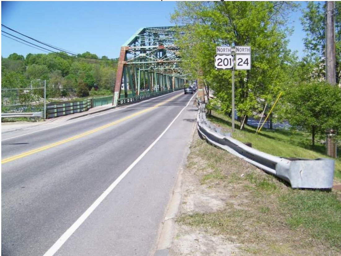
Photo 86 – No guiderail is present at southwest bridge corner (at left) because there is a section of railing attached to the U-shaped wingwall. Also note guiderail impact damage.
