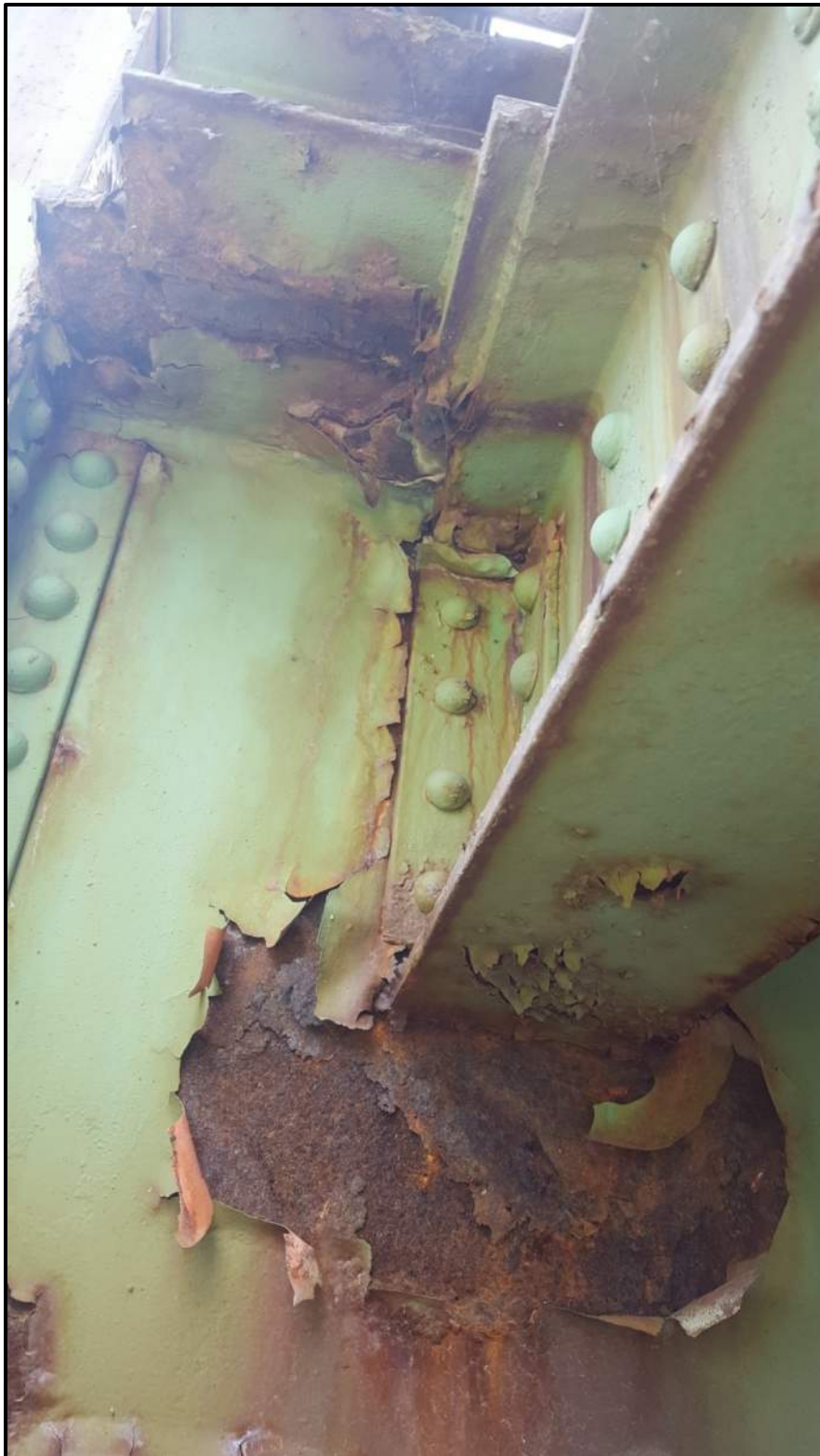
Photo A17 – Stringer 8 connection to Floorbeam 5 shows active corrosion.
