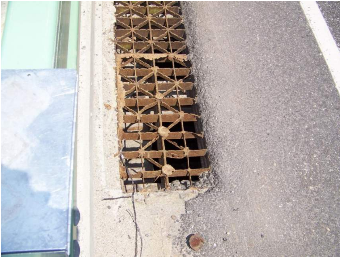
Photo 11 – Several damaged, perforated, and failed secondary distribution bars were observed in open grid gutter drainage strips. Looking north along west curb near Pier 2.
