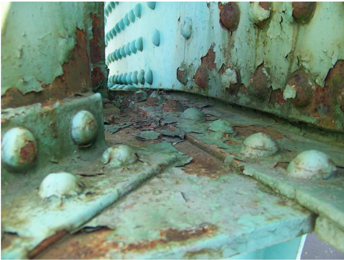
Photo 67 – Many of the upper chord lateral bracing connection plates have paint failures and active corrosion. View at Span 1 roadway truss U8.
