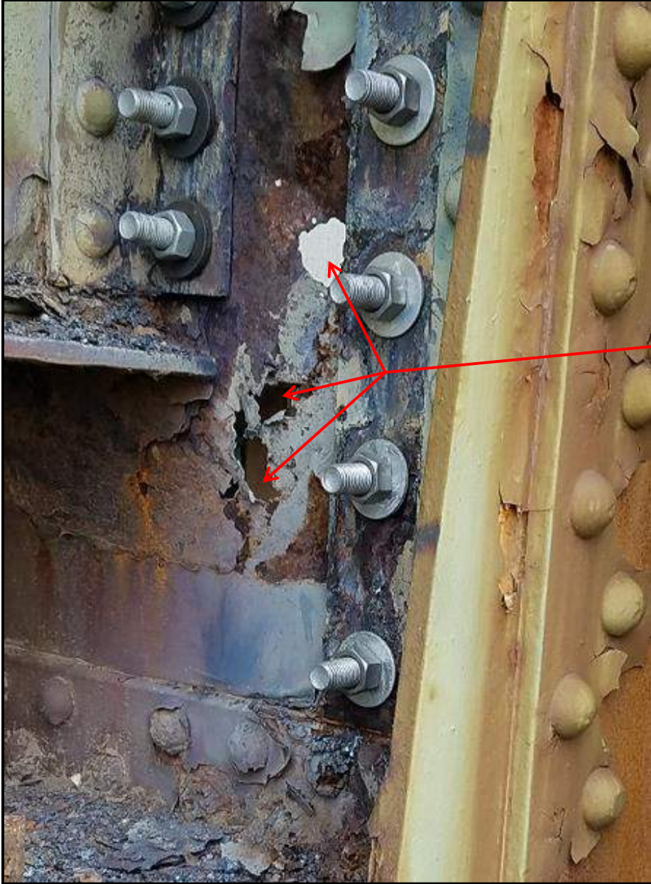
Floorbeam 7 was in the worst condition.
