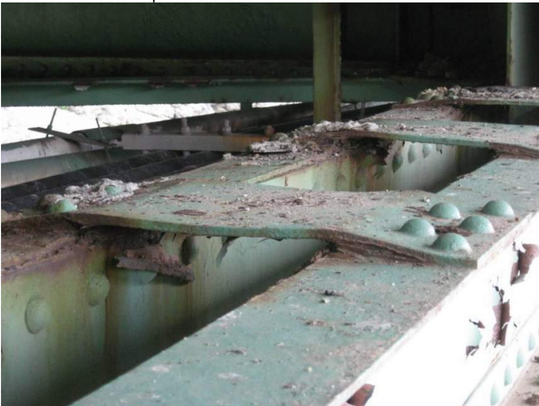
Photo 30 – The most severe instance of bowing of the top face lower chord tie plates was observed at Span 3 sidewalk truss at the third tie plate north of L0.
