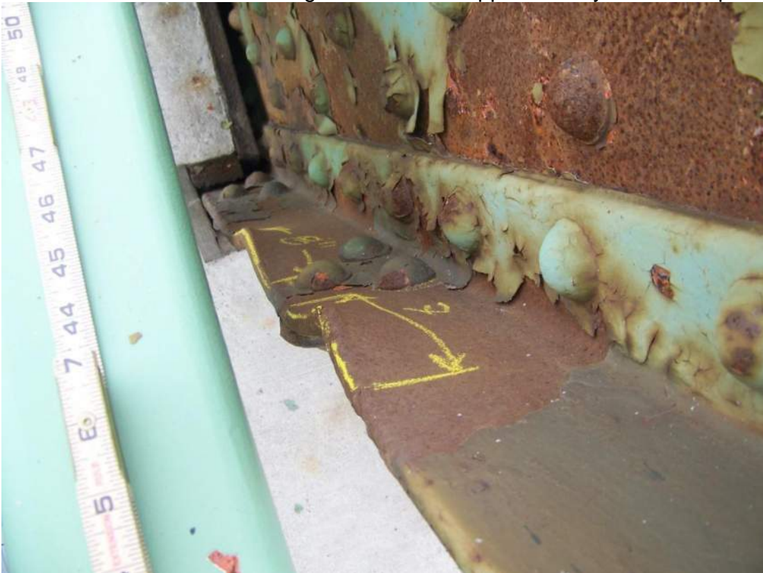
Photo 36 – Impact damage to the Span 3 sidewalk truss L0-U1 end post was observed which has caused two bends of \frac{3}{4} to 1 inch to the northeast corner angle.
