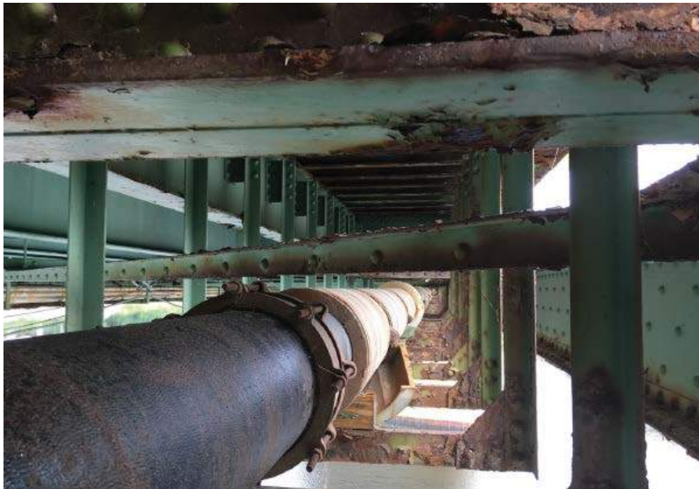
Photo #48: General view of lateral bracing spanning between utility supports in span 1 & 2 (8/1/16)
