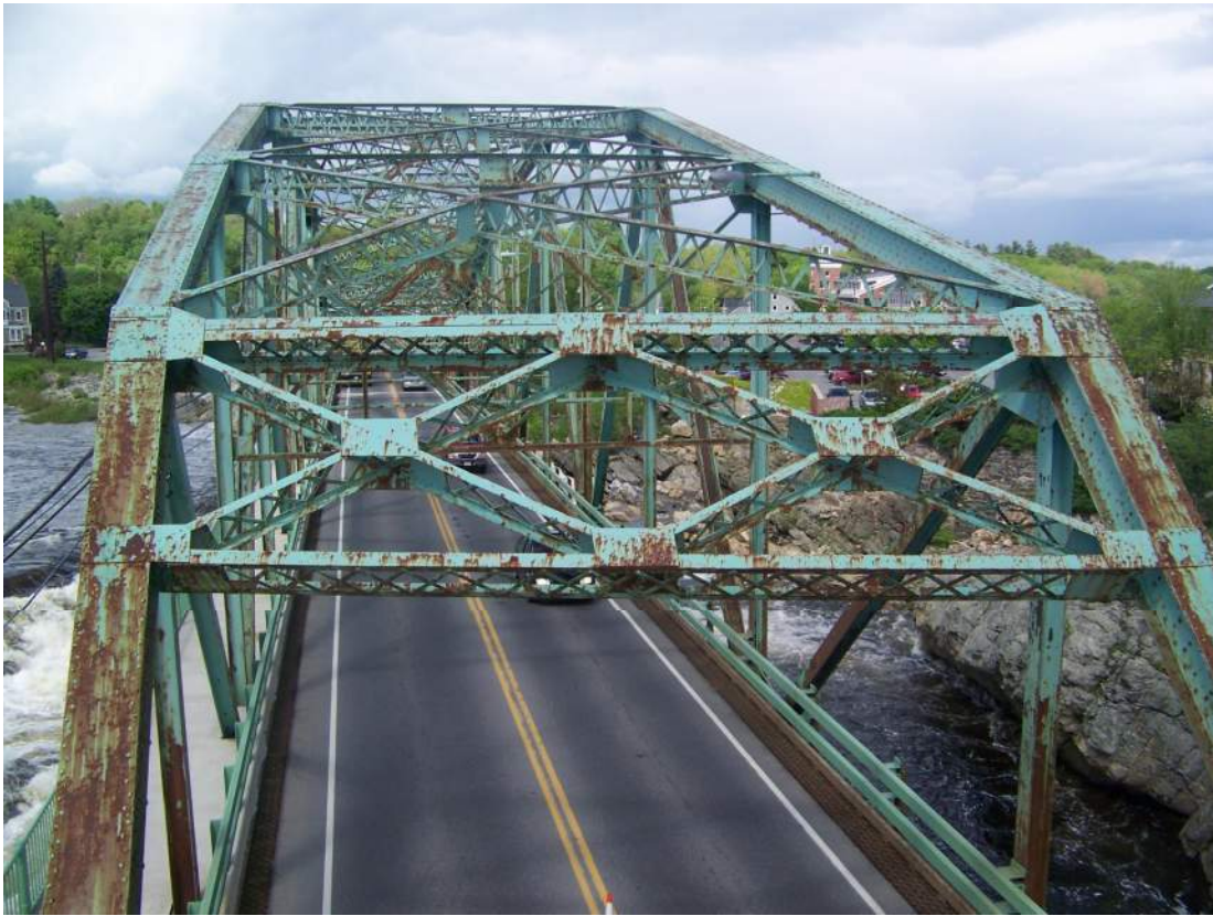
Photo 65 – The paint system is failed over more than 30% of the surfaces of the top chord lateral bracing. Looking north toward Span 2 portal.
