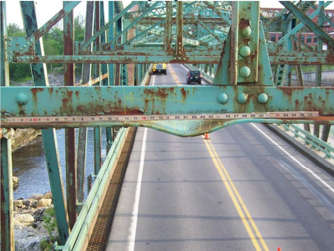
Photo 70 – Span 3 U6 sway frame strut has impact damage which has deflected the north horizontal leg downward by 1\frac{1}{4} " over northbound lane just east of bridge centerline.
