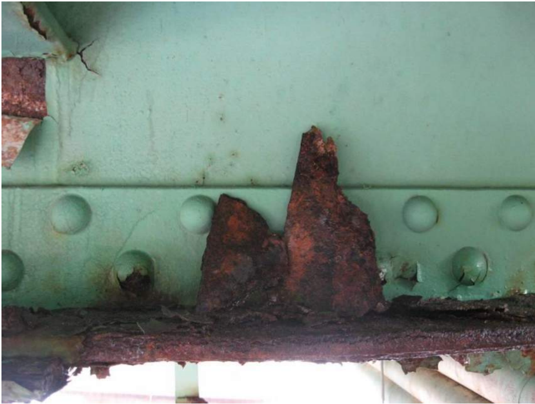
Photo 47 – Span 2 FB4 has a 4” wide by 8” long zone of active corrosion/ delamination with 1/8” section loss to top of bottom flange on north side of web at 2 feet west of S4.
