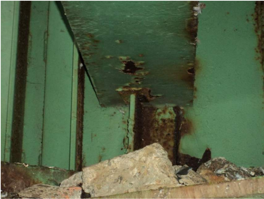
Photo 53 – The north face of the Span 1 end floorbeam FB0 has a welded plate stringer bearing stiffener below S3 which constitutes a fatigue-sensitive detail in a FCM.
