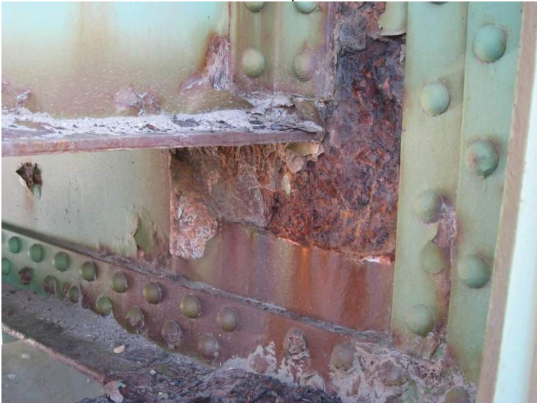
Photo 44 – At Span 1 FB7 below S8 both faces of the web exhibit active corrosion with section loss of 1/8 inch depth over a height of 8 inches and length of 12 inches.
