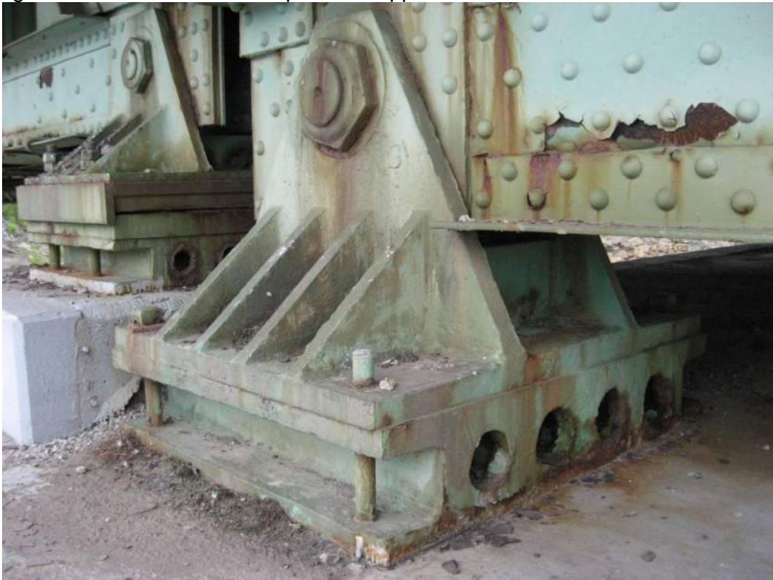
Photo 76 – The Span 2 sidewalk truss fixed bearing at Pier 2 is missing a nut on the southwest anchor bolt. View looking northeast.
