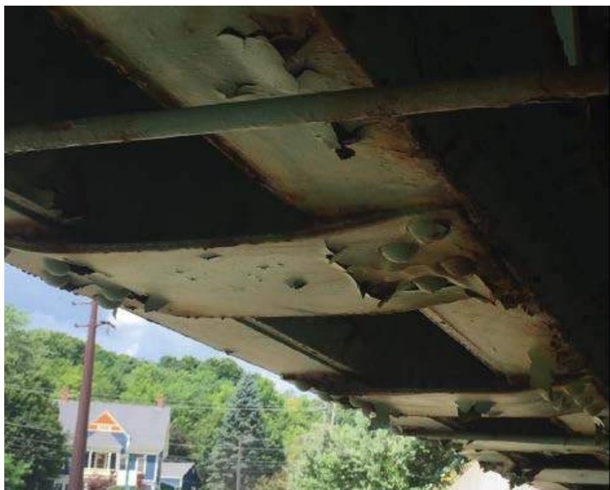
Photo #32: "Bowing" of lattice plates on the bottom chord of the sidewalk truss in span 3 (8/2/16)
