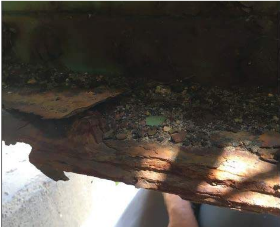
Photo #37: Pack rust between plates on the bottom chord of the non-sidewalk truss in span 3 (eastern side of the bridge) (8/2/16)
