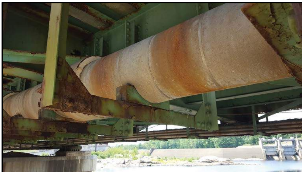
Photo A24 – The Utility Brackets are in poor condition with extensive active corrosion.
