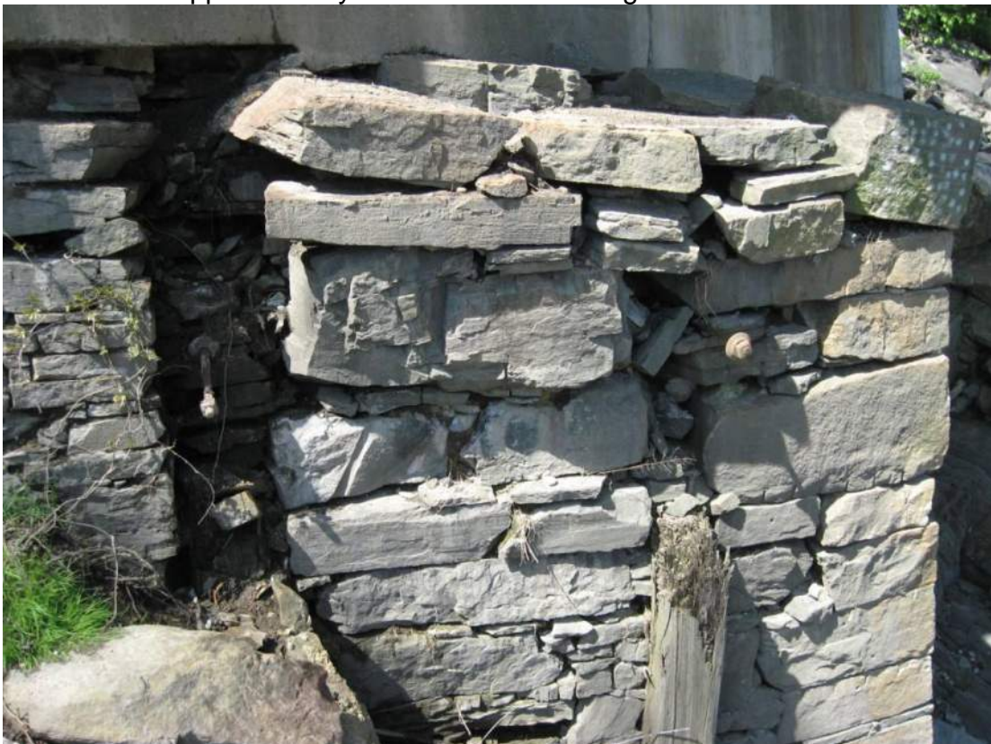
Photo 78 – Older stone masonry portions of south abutment exhibit remnants of missing timber bracing anchors and possible signs of outward shifting of a few of the stones.
