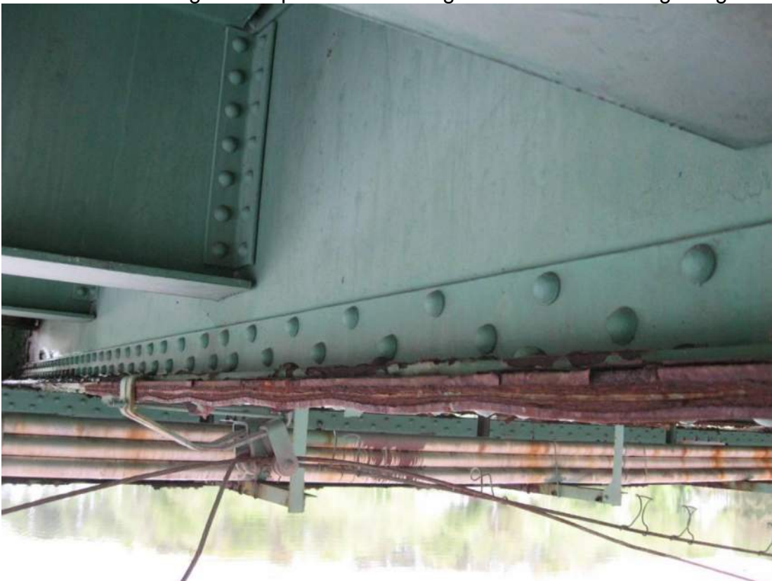
Photo 40 – An active pack rust condition was noted in the Span 2 FB5 floorbeam between S5 and S6.
