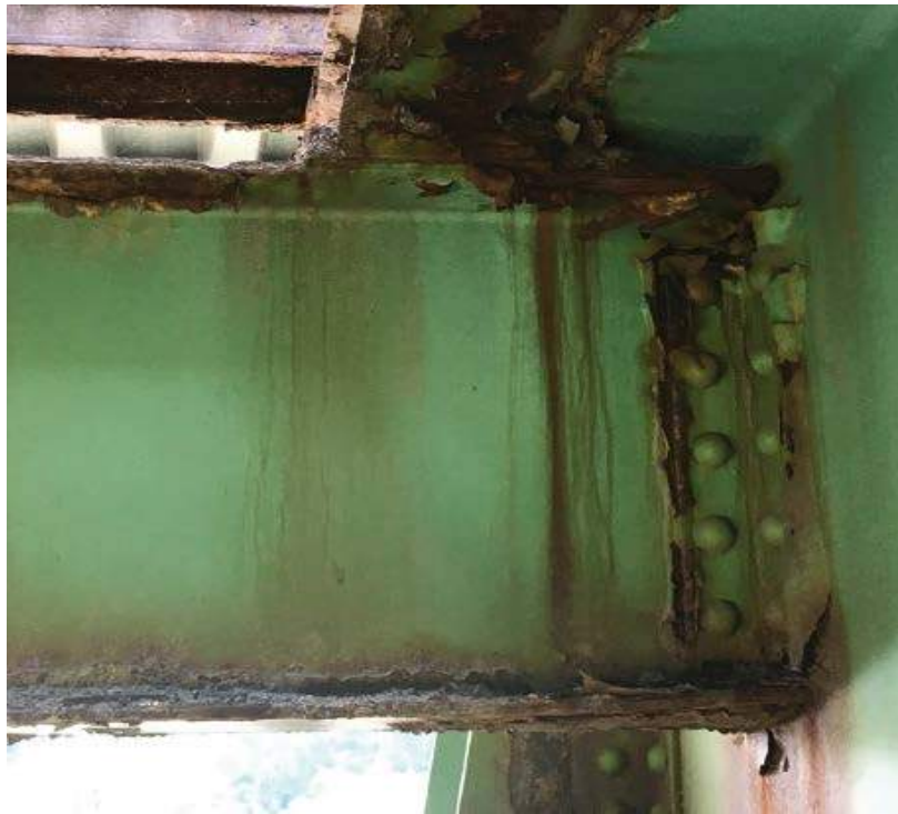
Photo #27: Moderate corrosion to S3 in span 3 near FB4 (8/2/16)
