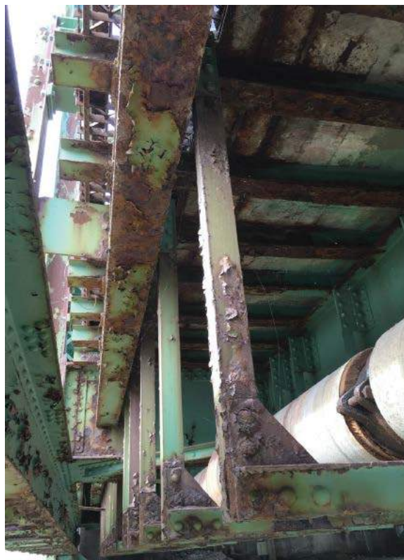
Photo # 8: General view of paint loss and corrosion to bays below the open grid decking in the travel way shoulders on the non-sidewalk side (eastern) of the bridge (8/1/16)
