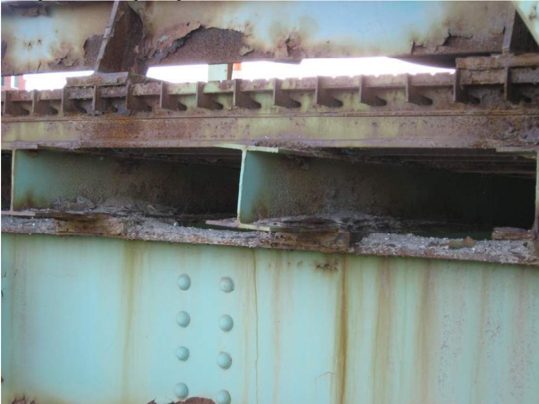
Photo 62 – The east end of a grid deck cross-beam above S8 between L7 and L8 was observed to be twisted around cross-beam axis due to pack rust at the S8 connection.
