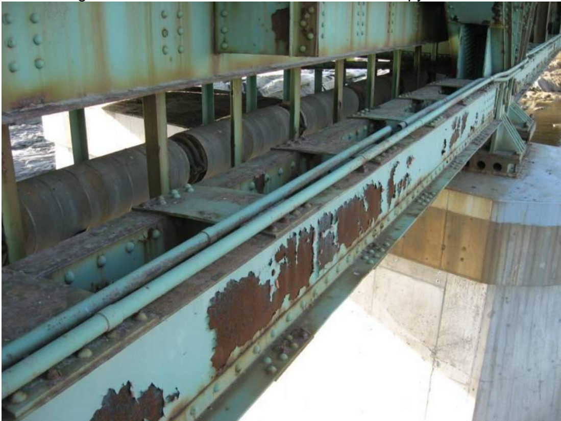
Photo 88 – Two conduits for bridge lighting have a 3" separation in one conduit in Span 1 along top face of roadway truss between L9 and L10 with exposed electrical cables.
