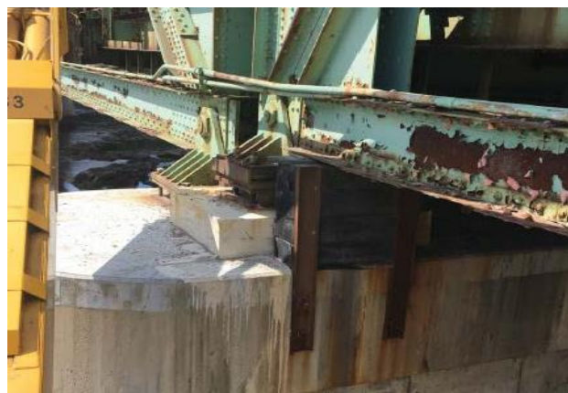
Figure 16: Damaged concrete pedestals
