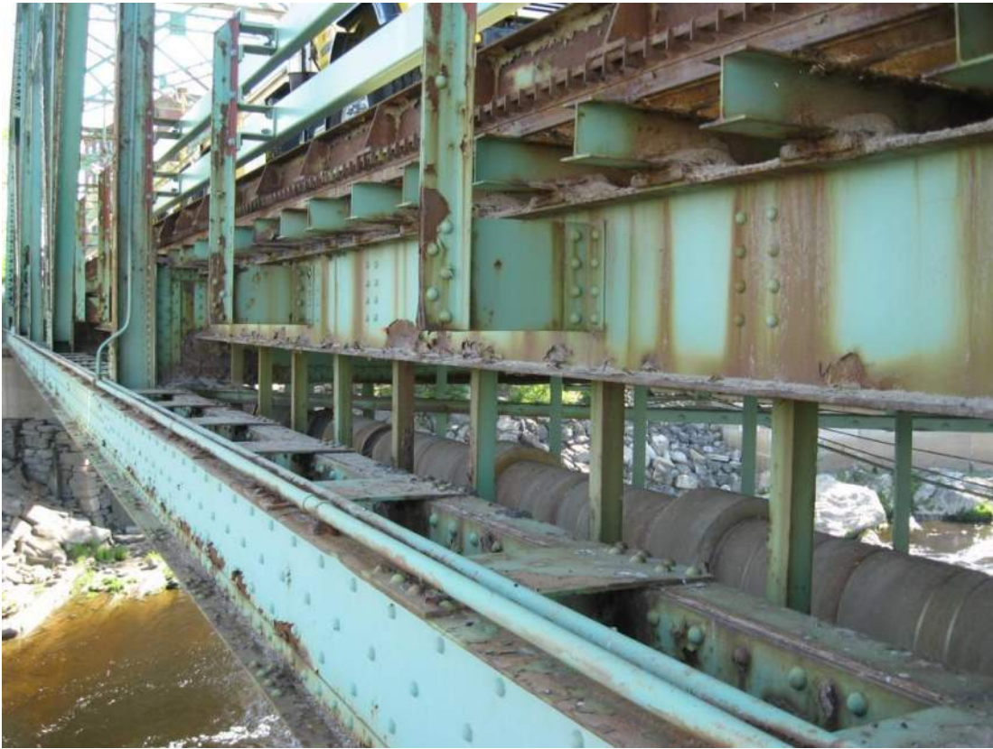
Photo 23 – The roadway truss lower chord top face exhibits poor paint condition with missing paint and active corrosion typical throughout bridge. View of Span 1 L5-L6.
