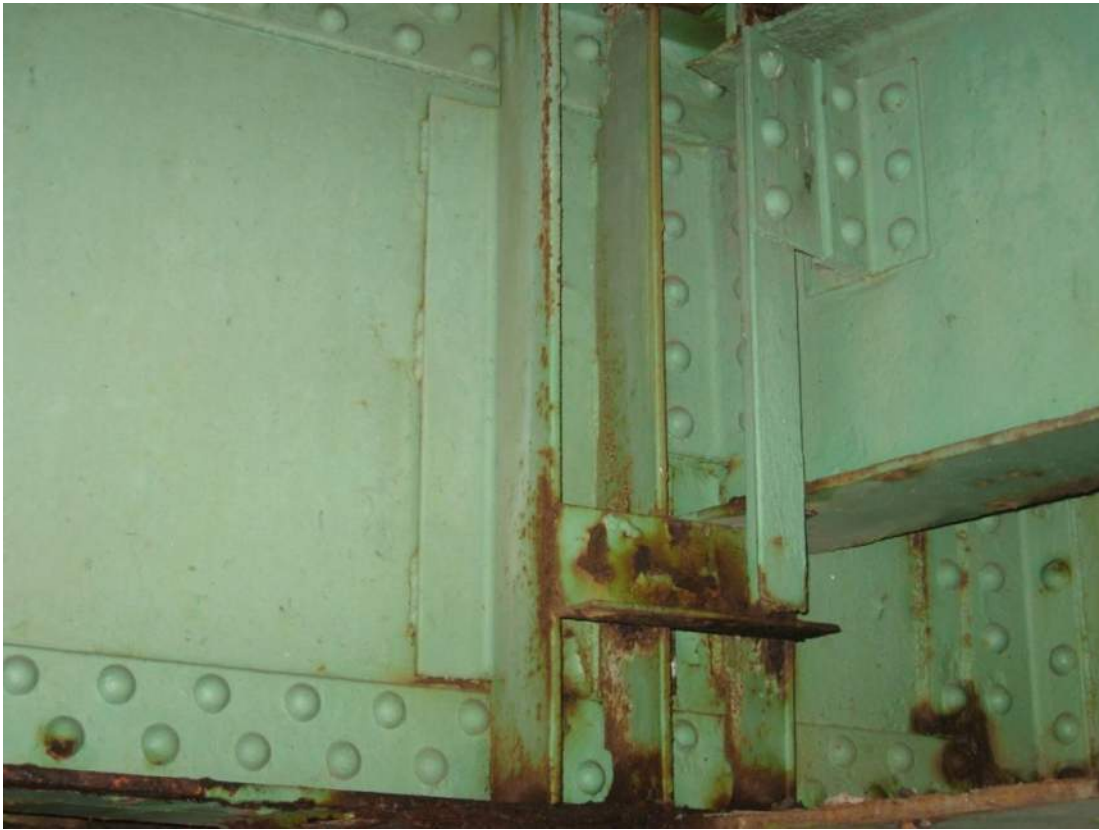
Photo 51 – Full height welded jacking stiffeners were also noted on north face of Span 2 and 3 FB0 webs (on face opposite deck joint) at sidewalk and roadway truss ends.
