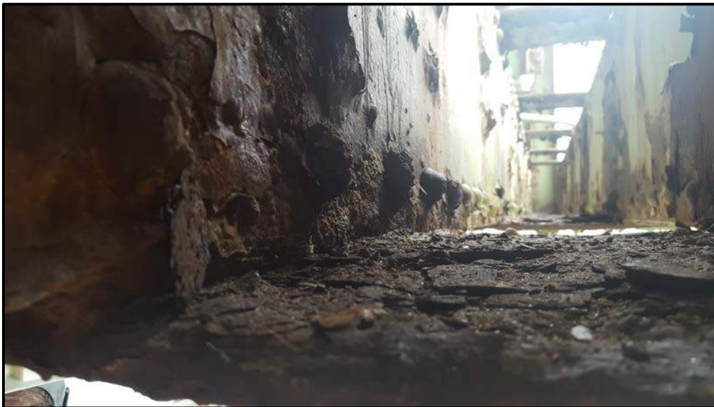
Photo A11 – This is the general condition view of the inside lower chord truss member collecting rust and debris on the lacing bars.
