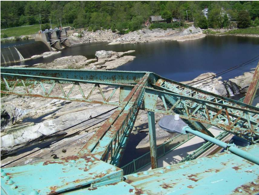
Photo 64 – The paint system is failed over more than 30% of the surfaces of the top chord lateral bracing. View looking northwest in Span 1 toward U9 sidewalk truss.
