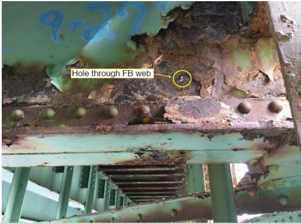
Photo # 13: Closer image of hole through the web of FB2 in span 1 (8/1/16)
