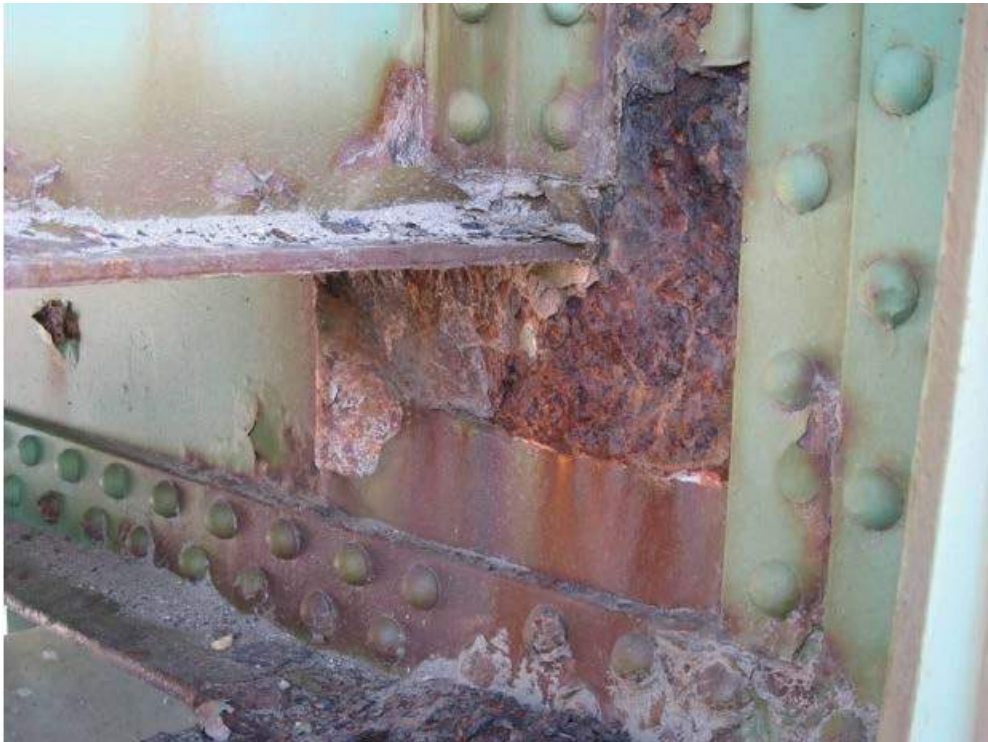
Photo 44 – At Span 1 FB7 below S8 both faces of the web exhibit active corrosion with section loss of 1/8 inch depth over a height of 8 inches and length of 12 inches.
