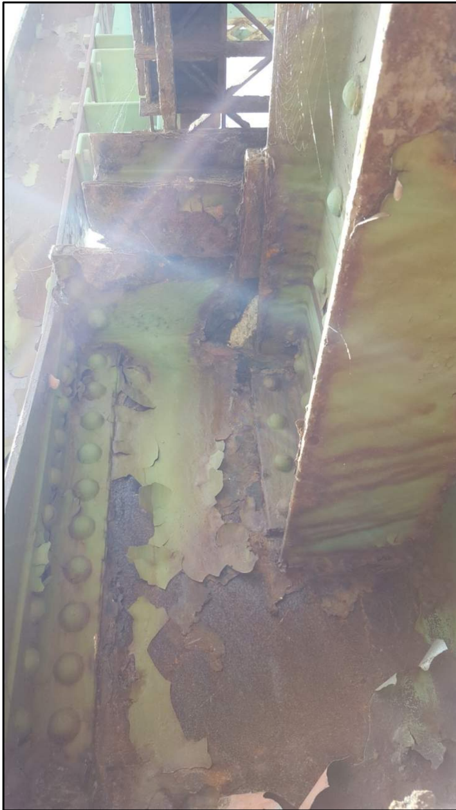
Photo A15 – Stringer 8 connection to Floorbeam 1 showing active corrosion.
