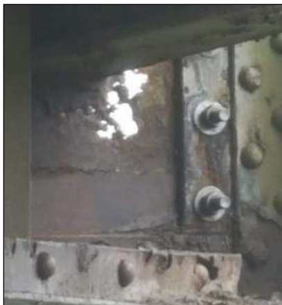
Another view of Floorbeam 7 deterioration prior to repair.
