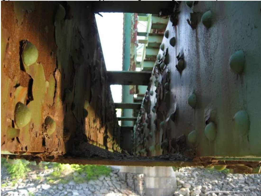
Photo 24 – The interior vertical faces of the roadway truss lower chord also exhibit poor paint condition with missing paint and active corrosion typical throughout. Span 1, L6-L7.
