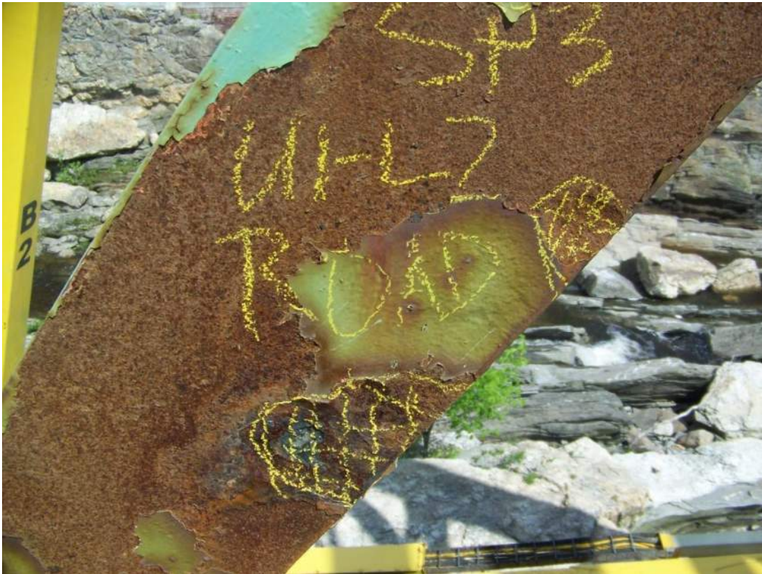
Photo 35 – At 5 feet above the deck in Span 3 roadway truss U1-L2 there is a zone of 1/8 inch section loss to west face of flange over an area approximately 5 inches square.
