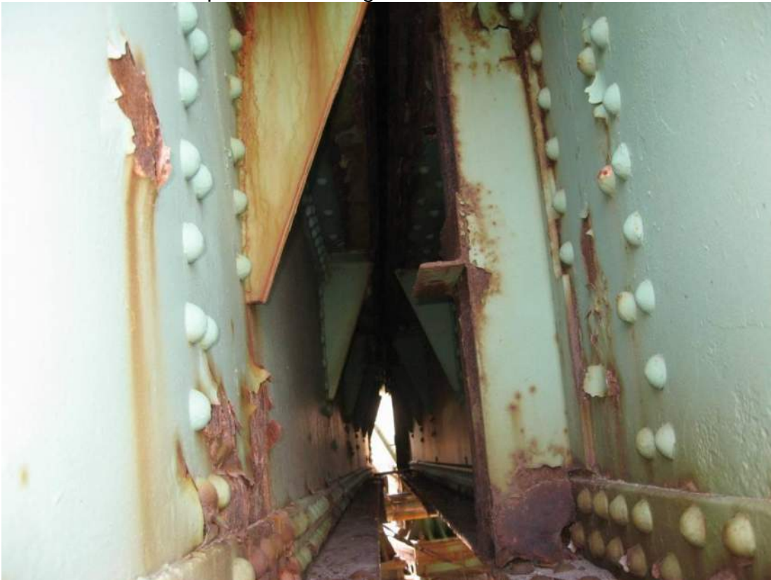
Photo 48 – The end floorbeams over Pier 1 have partial height welded stiffeners on face of web below deck joint, which constitutes a number of fatigue-sensitive details in FCM's.
