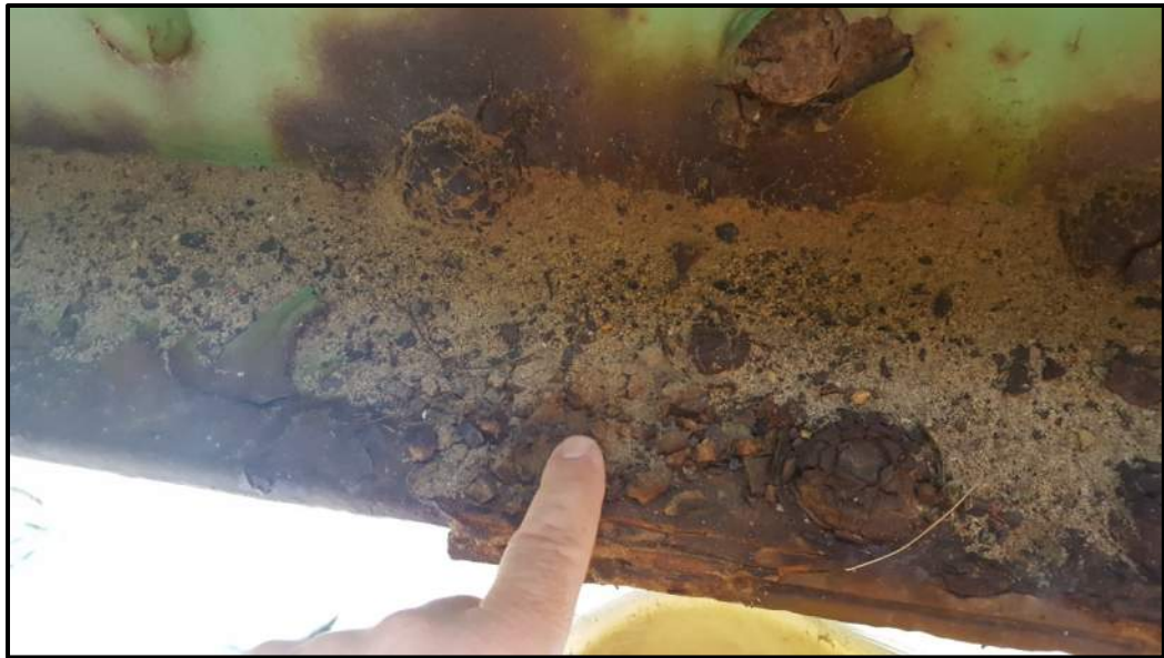
Photo A5 – Floorbeam 5 coverplate has enough deterioration issues to expect a repair within 5 years.
