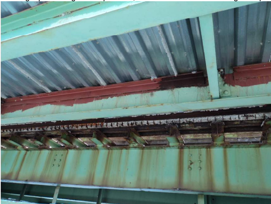
Photo 58 – Similar repairs were also observed on sidewalk stringer S2 where the top flange angle repair was left prime-painted only on both sides of the stringer.
