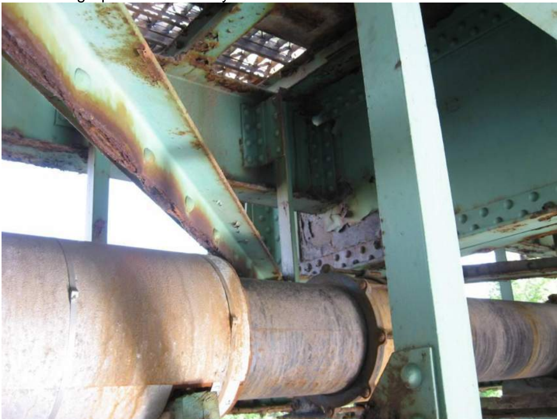
Photo 72 – Severe pack rust with active corrosion between back to back angles of lower lateral bracing connecting Span 1 L5 roadway truss and L6 sidewalk truss at L5 end.
