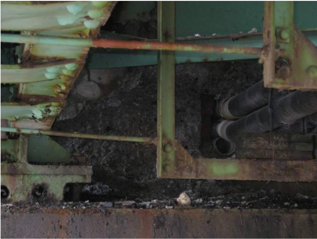
Photo 81 – There is a large 3 foot by 3 foot by 3 inch deep spall in lower portion of backwall around edges of utility conduit penetration and extending behind sidewalk truss.
