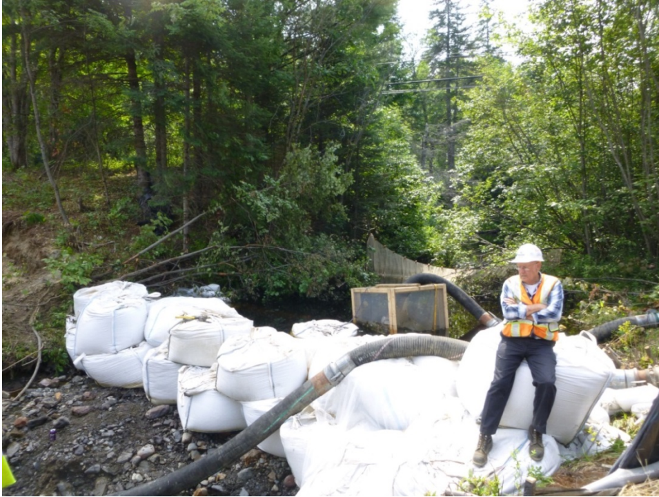
Cofferdam made of industrial sandbags. Bypass pump intake upstream of the cofferdam.
