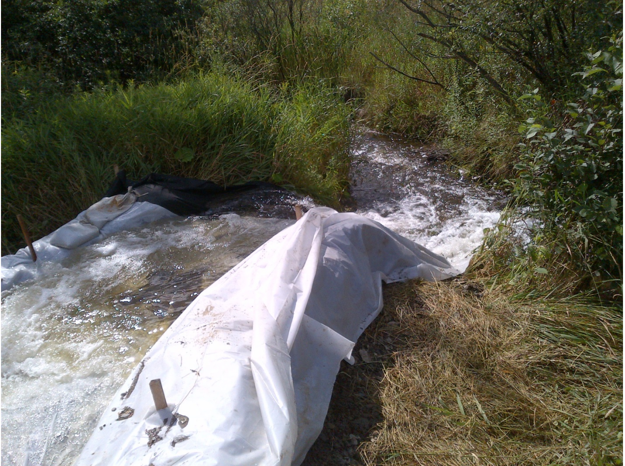
Poly and Hay Bales used for a pump outlet or the outlet of a bypass channel
