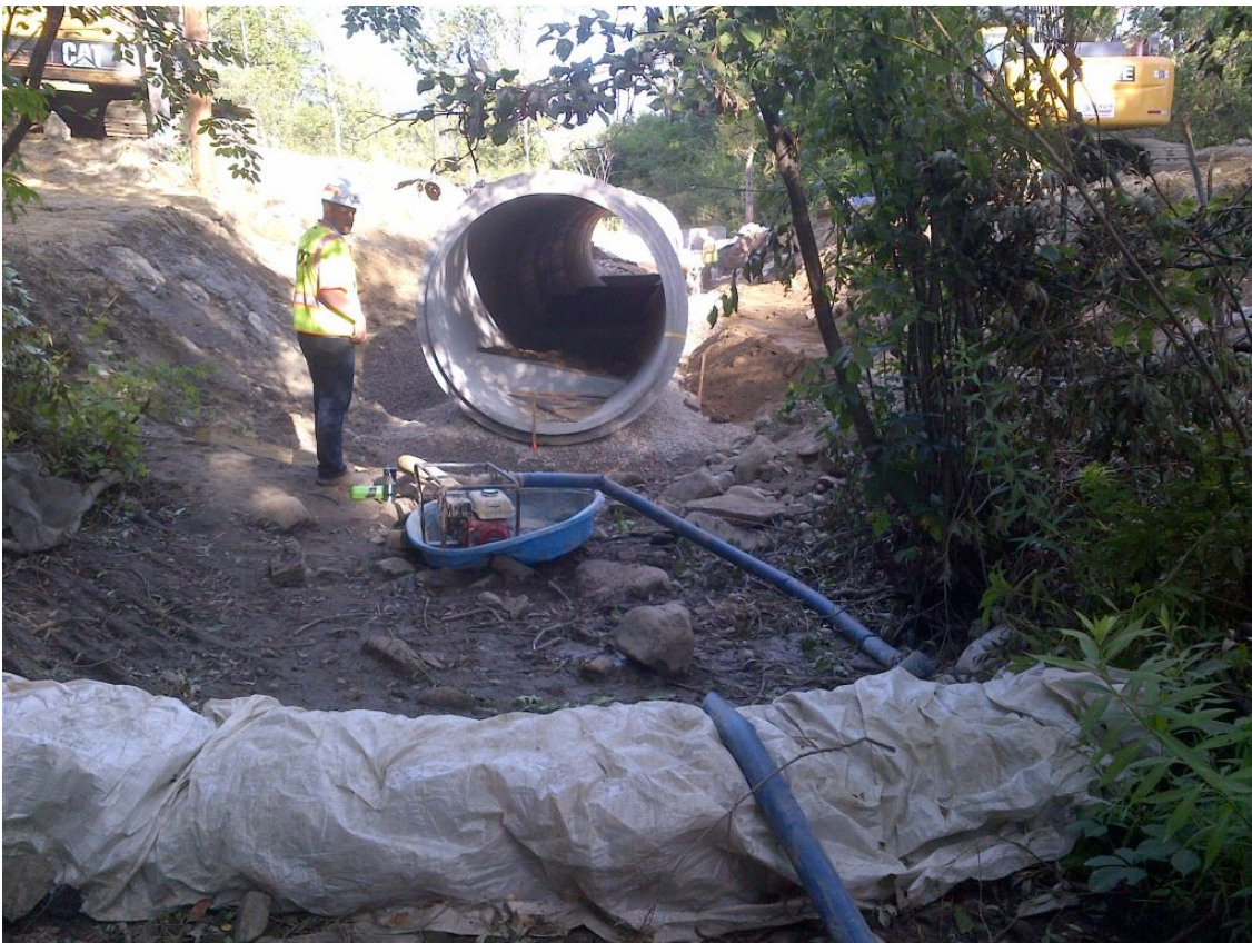
A dewatered work area with a small pump to maintain the dry work area.
