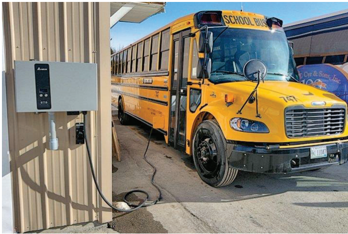
2 Electric bus and charging station
