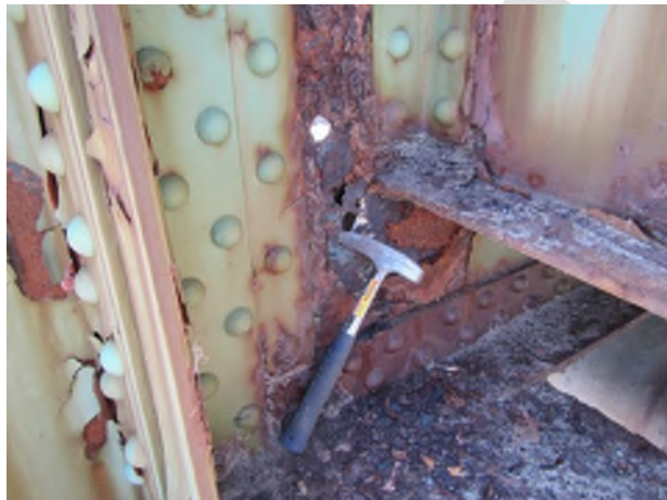
Figure 8: Hole in floorbeam
