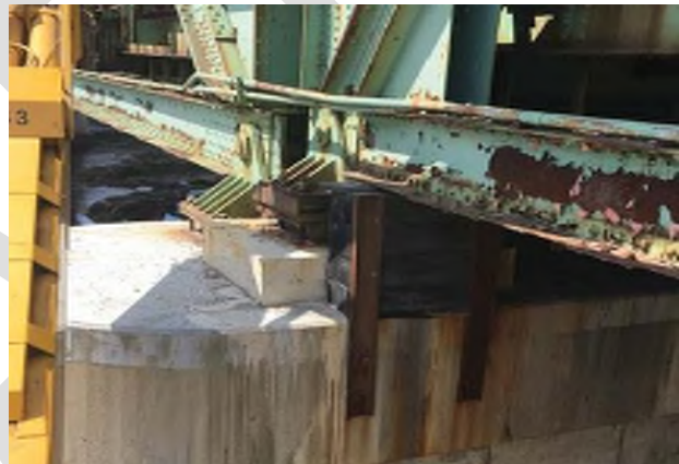
Figure 13: Damaged concrete pedestals
