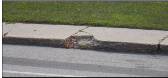
Many sidewalks through downtown are narrow, cracked, and chipped, creating safety challenges.
