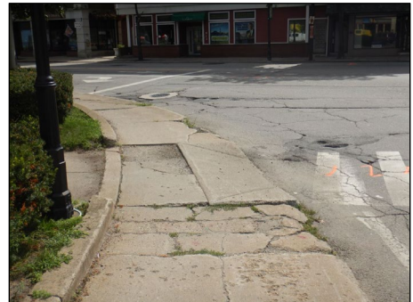
This crosswalk landing lacks ADA amenities and sidewalk cracks make it difficult to negotiate.
