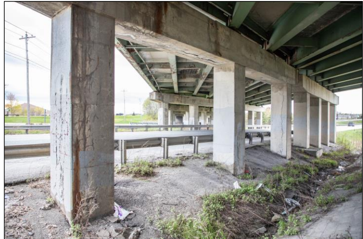
Figure 11 Under the overpass showing spalling and deterioration to the concrete.
