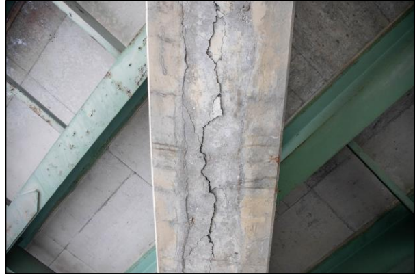
Figure 14 Cracks in concrete caps.
