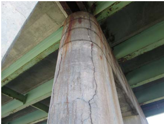
Merrill Road Bridge – South cracking Column
