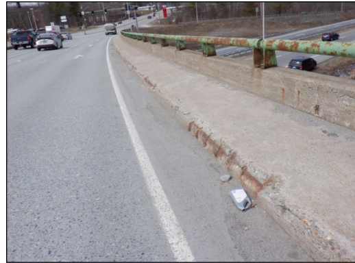
Curb exhibiting exposed rebar unsatisfactory to stop a vehicle moving at 35 mph.
