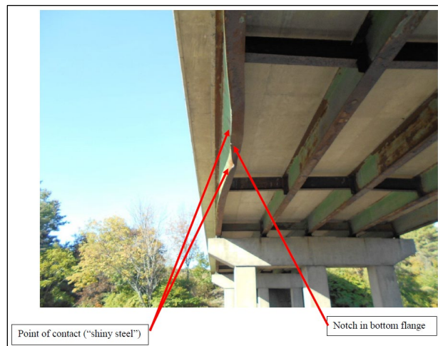
Ramp F following impact with an excess height vehicle in 2017.
