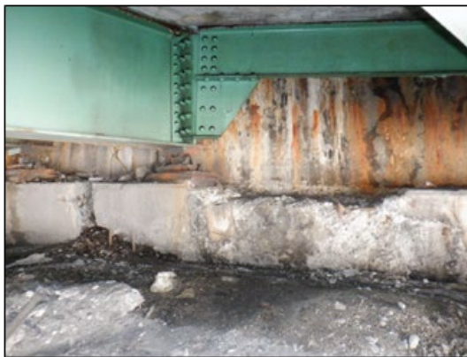
Deterioration at west abutment.
